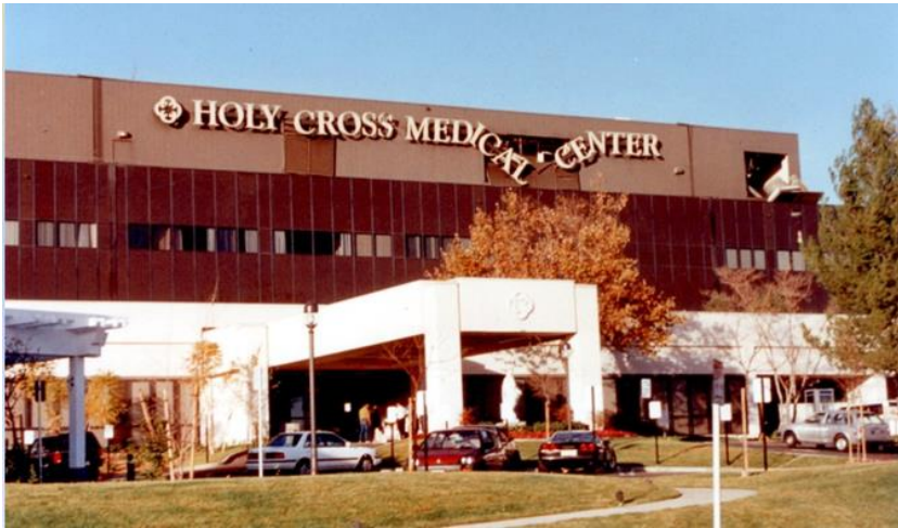
Figure 2.4.3-2 HVAC damage at Holy Cross Medical Center in Sylmar in the 1994 Northridge Earthquake. Damage to signage and louvers was caused when suspended fans in the mechanical penthouse swung and impacted the louver panels. HVAC service outage caused the temporary evacuation of patients (FEMA 74, 1994).
