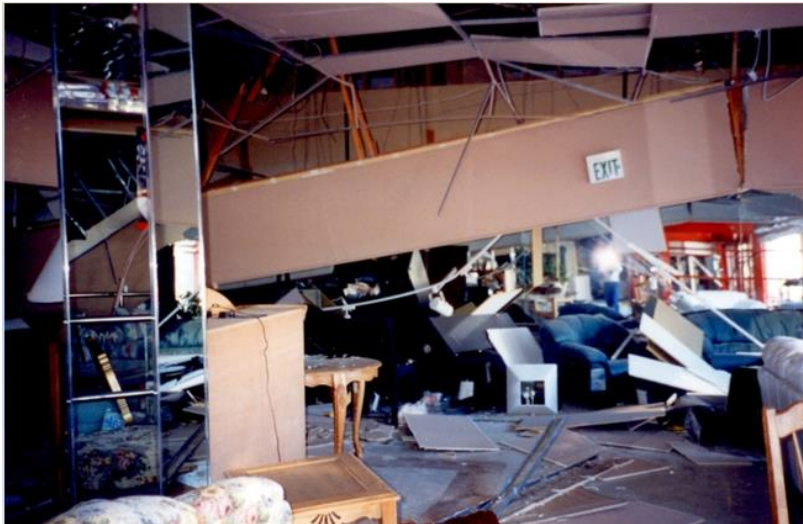
Figure 2.4.1-3 Failure of suspended ceilings and light fixtures in a furniture store (FEMA 74, 1994).
