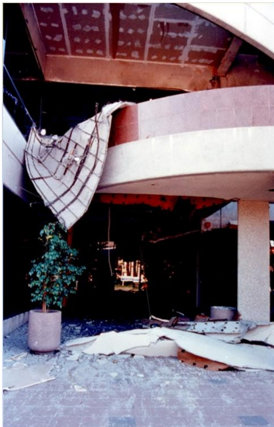
Figure 2.4.1-4 Failure of heavy stucco soffit at building entrance in the 1994 Northridge Earthquake (FEMA 74, 1994).
