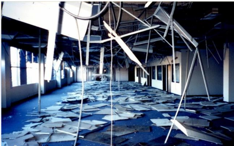
Figure 2.4.2-1 Complete loss of suspended ceilings and light fixtures in the 1994 Northridge Earthquake (FEMA 74, 1994).
