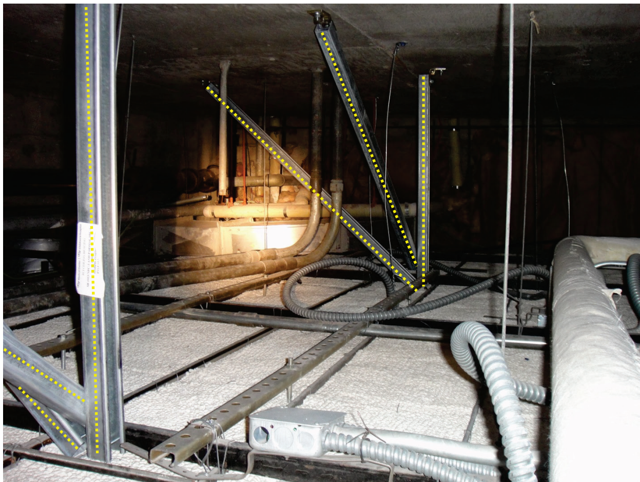
Figure 6.3.4.3-4 Details of suspended and braced plaster ceiling,. Rigid bracing and compression posts (highlighted) are provided at 6 ft by 8 ft on center. Note cross furring saddle tied to black channel (main runner) from below; supplementary framing for lights runs parallel to cross furring and saddle tied to main runner from above (Photo courtesy of Maryann Phipps, Estructure).
