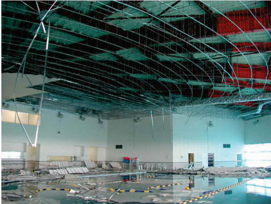
Figure 6.3.4.3-2a Complete collapse of a large suspended gypsum board ceiling over a swimming facility in Japan (Photo courtesy of Shojiro Motoyui, Tokyo Institute of Technology). This type of failure has been replicated on the E-defense shake table and occurs when the U-shaped clip holding the cross furring (M-bar) to the main runners (channel) opens into a V-shape and drops the furring grid. This type of failure is not common in the U.S.
