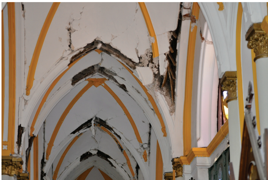
Figure 6.3.4.3-1 Damage to ornate wire lath and plaster ceiling in the 2010 magnitude-8.8 Chile Earthquake (Photo courtesy of Eduardo Fierro, BFP Engineers). Wire lath is attached to arches or to wood furring suspended from the roof framing.
