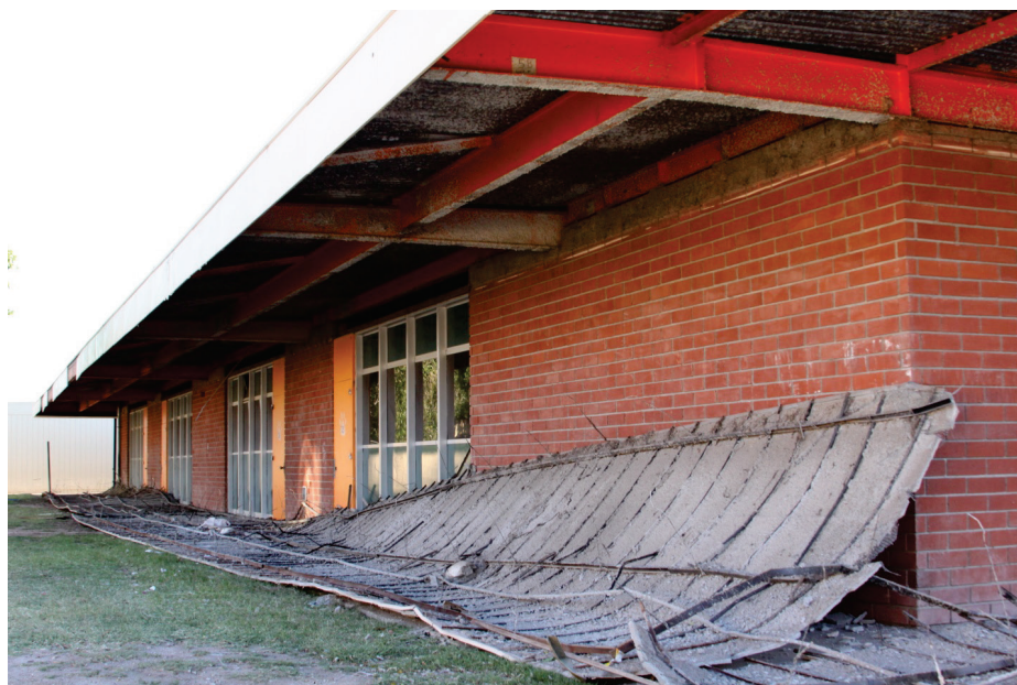
Figure 6.3.4.3-3 Collapse of exterior soffit at Jefferson Elementary School in Calexico in the 2010 Baja California Earthquake; approximately 1200 sq ft of soffit collapsed at this school built in the 1960's (Photo courtesy of Baja Earthquake Reconnaissance Team, Earthquake Engineering Research Institute (EERI), published in the EERI July 2010 Newsletter).
