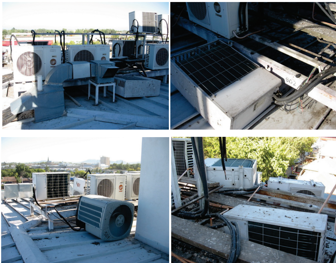
Figure 6.4.1.4-3 Numerous poorly anchored rooftop units toppled in the 2010 Chile Earthquake (Photos courtesy of Rodrigo Retamales, Rubén Boroschek & Associates).
