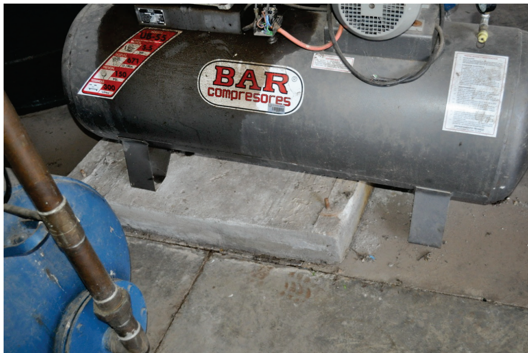
Figure 6.4.1.4-1 Poorly anchored compressor jumped off the undersized anchor bolts in the 2010 magnitude-8.8 Chile Earthquake (Photo courtesy of Eduardo Fierro, BFP Engineers).
