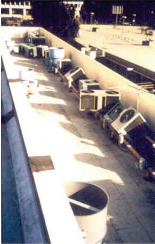
Figure 6.4.1.4-2 Unanchored rooftop units thrown off their supports during an earthquake (Photo courtesy of Maryann Phipps, Estructure).
