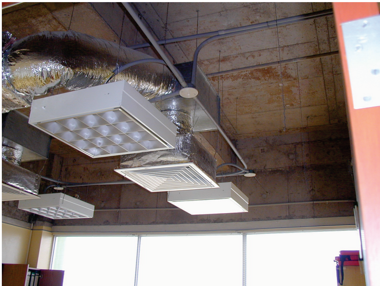
Figure 6.4.6.2-2 HVAC diffuser attached to the structure with four vertical hangers; ceiling system was damaged beyond repair in the 2001 Peru Earthquake but none of the diffusers or lights fell. Ceiling was demolished prior to photo (Photo courtesy of Eduardo Fierro, BFP Engineers).
