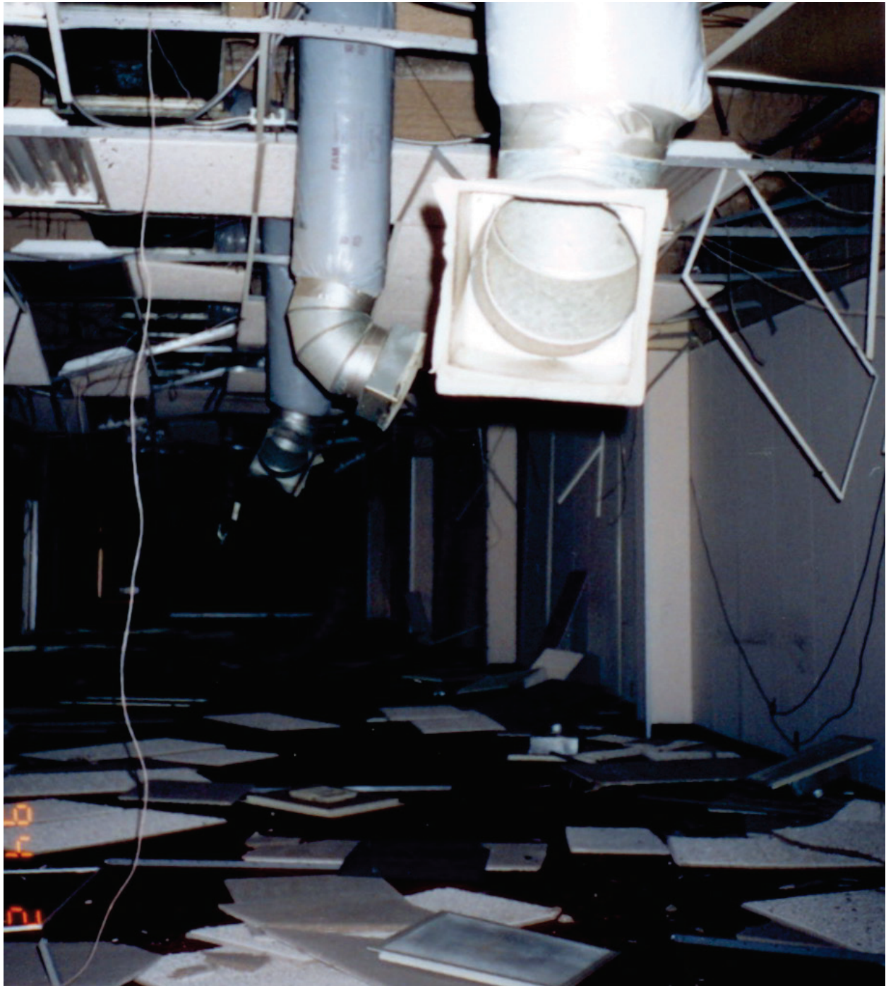
Figure 6.4.6.2-1 Air diffusers fell to the floor; ducts hanging through ceiling grid as a result of the 1994 Northridge Earthquake (FEMA 74, 1994).
