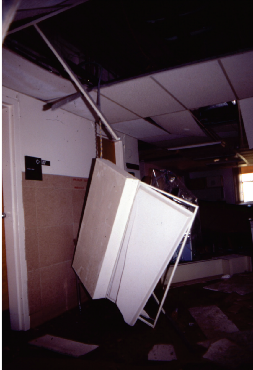
Figure 6.4.9.1-4 Light fixture without independent support dangling from conduit as a result of the 1994 Northridge Earthquake (Photo courtesy of Degenkolb Engineers).
