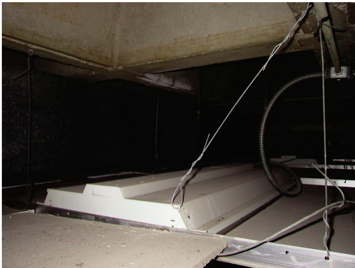
Figure 6.4.9.1-5 Example of light fixture with only one safety wire attached; the Salt Lake City schools require four wires for a fixture of this size and weight and also require tighter turns on the wire (Photo courtesy of Salt Lake City School District). Investigations in ceiling plenums often reveal missing wires.
