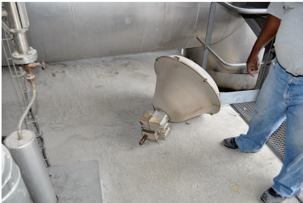
Figure 6.4.9.3-3 Failure of pendant light fixture in the 2010 magnitude-7 Haiti Earthquake; stem of fixture broke and conduit pulled loose (Photos courtesy of Eduardo Fierro, BFP Engineers).
