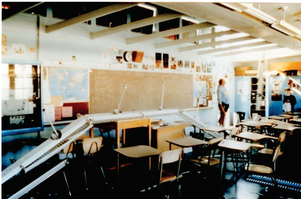
Figure 6.4.9.3-1 Failure of a strip of pendant light fixtures at Dawson Elementary School library as a result of the 1983 magnitude-6.4 Coalinga Earthquake. Note that in this case the support stems failed at the ceiling connection and the stem came down with the lights (Gary McGavin, NGDC, 2009).
