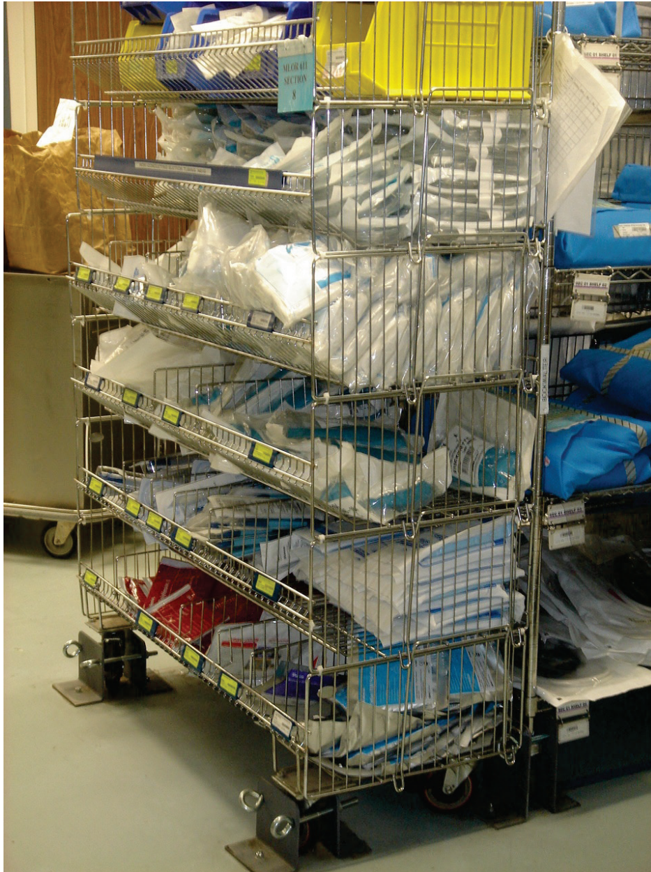
Figure 6.5.1.1-6 Mobile cart restrained at base with removable angles and eyebolts. Back-to-back units are interconnected (Photo courtesy of Maryann Phipps, Estructure).
