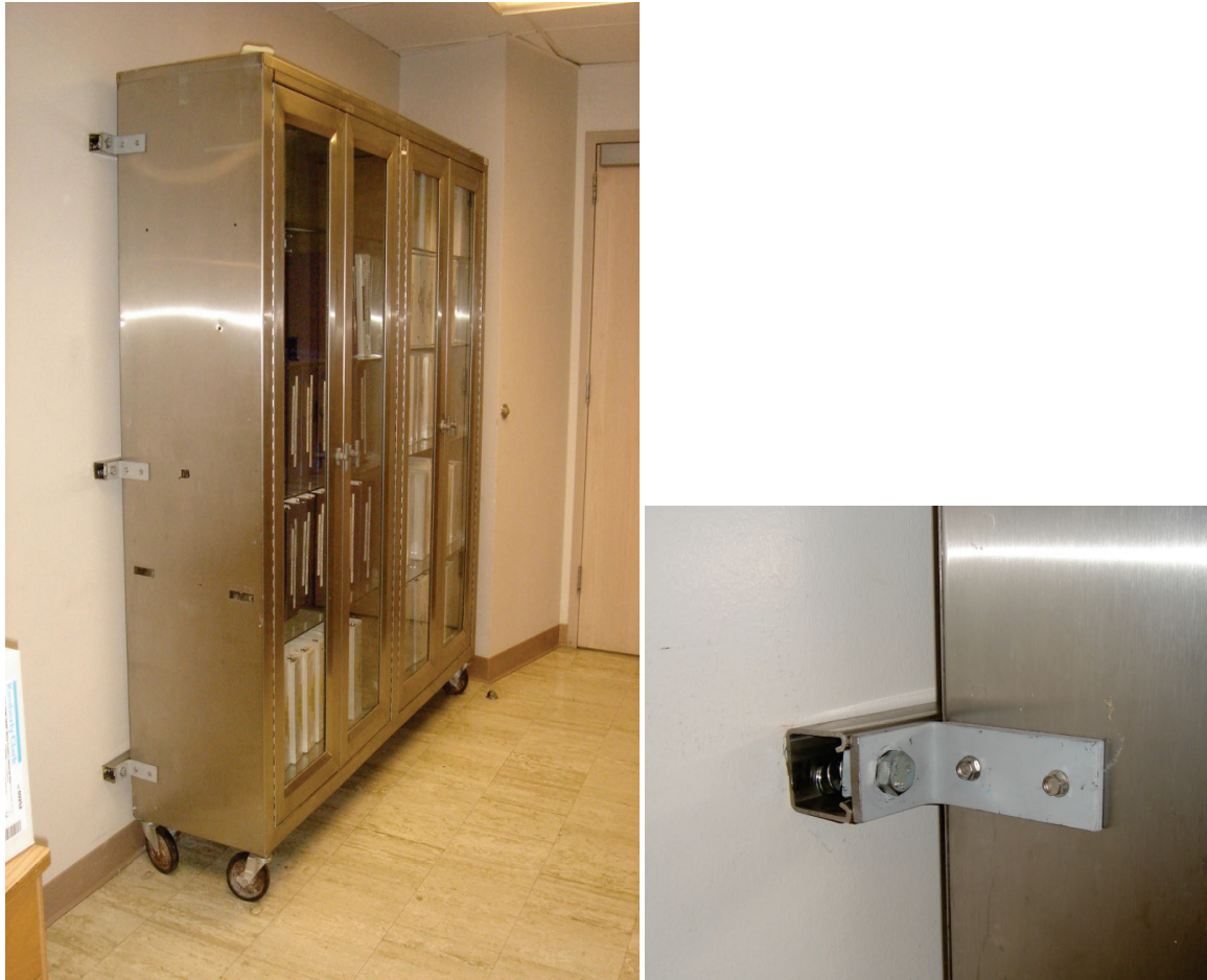
Figure 6.5.1.1-8 Mobile shelving unit restrained by connection to strut fastened to full height metal studs (Photo courtesy of Maryann Phipps, Estructure).
