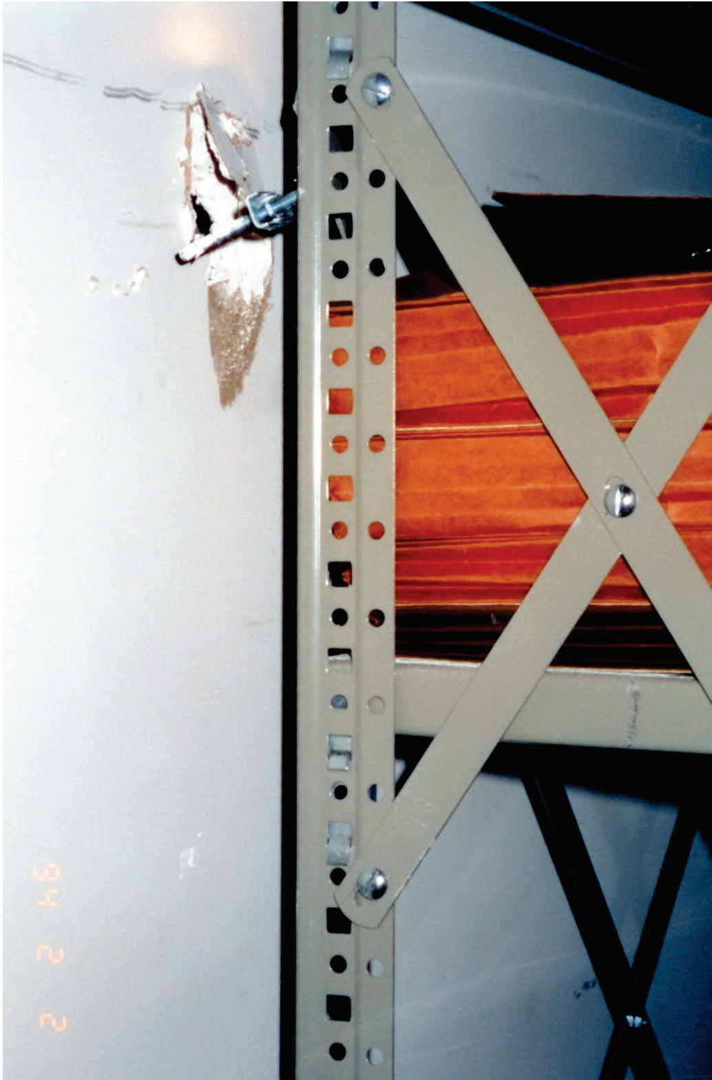
Figure 6.5.2.1-2 Failure of poorly anchored shelving; toggle bolt pulled out of gypsum board wall in the 1994 magnitude-6.7 Northridge Earthquake (Photo courtesy of Wiss, Janney, Elstner Associates).
