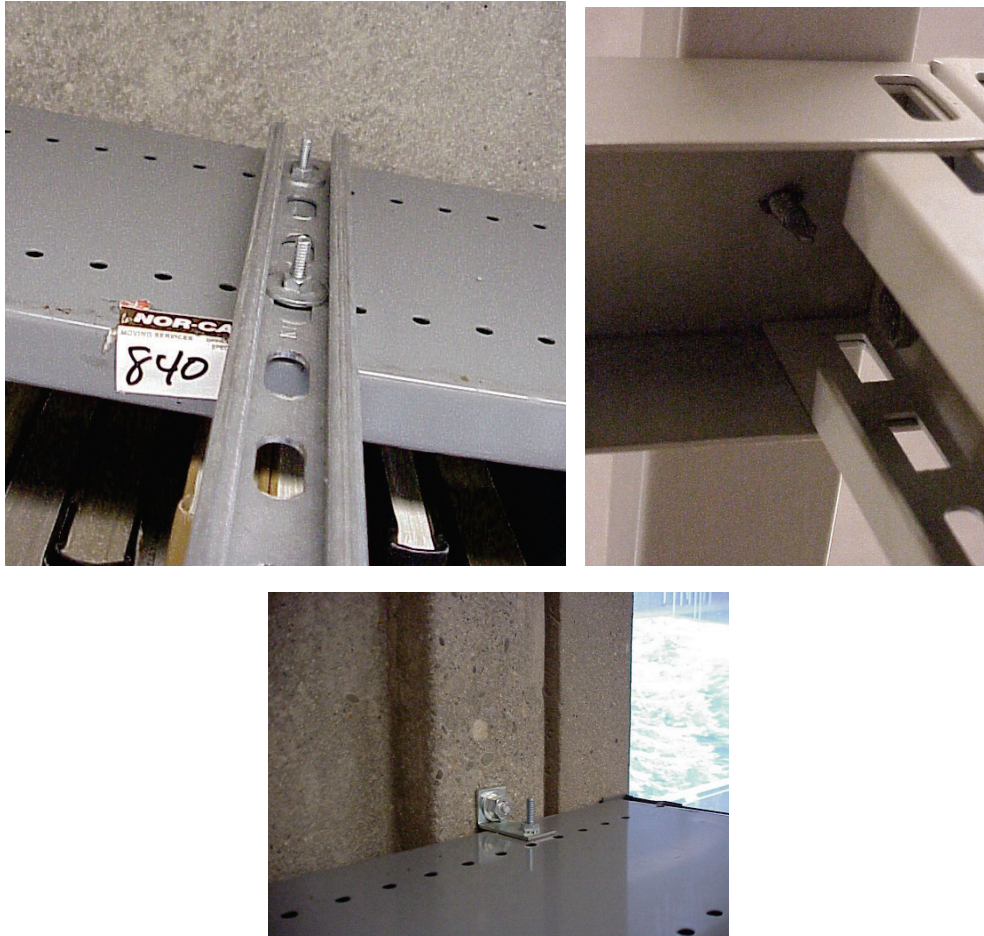
Figure 6.5.2.2-6 Examples of struts and hardware used to retrofit library shelving at the University of California, Berkeley (Photos courtesy of Mary Comerio, Dept. of Environmental Design, University of California Berkeley).
