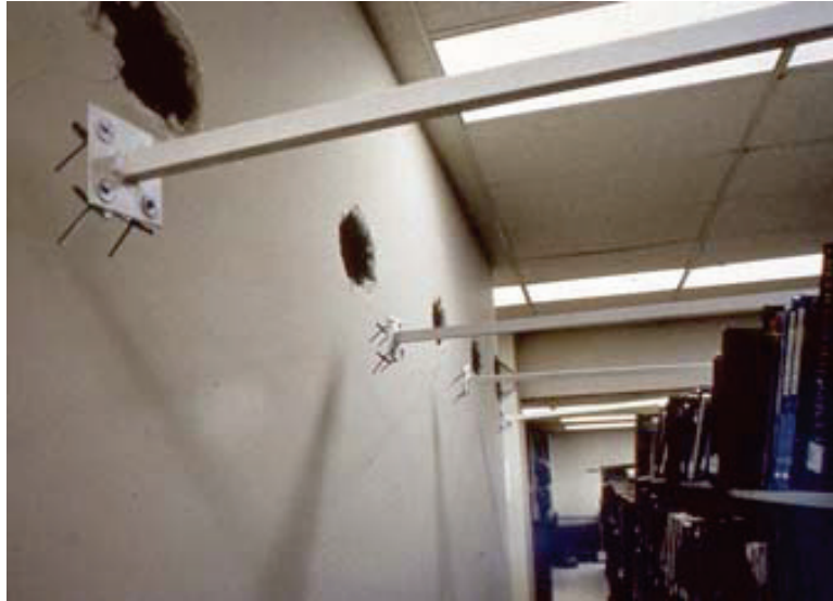
Figure 6.5.2.2-2 Failure of overhead transverse bracing for bookshelves were anchored to gypsum board partition in the 1984 magnitude-6.2 Morgan Hill Earthquake (Photo courtesy of Santa Clara County Office of Emergency Services). The anchors were not attached to wall studs, only to gypsum board.
