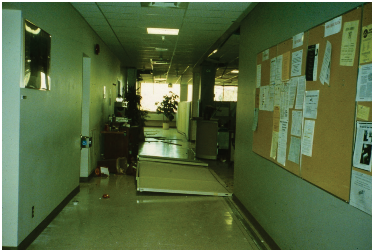
Figure 6.5.5.2-2 Damage to unbraced demountable partition in Silicon Valley office building in the 1989 magnitude-6.9 Loma Prieta Earthquake (Photo courtesy of Maryann Phipps, Estructure).
