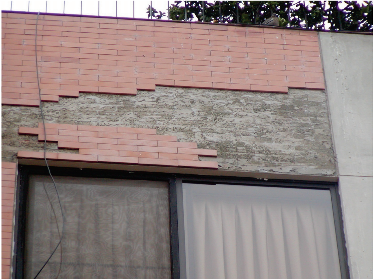
Figure 6.3.1.1-2 Close-up of failed adhered veneer. (Photo courtesy of Eduardo Fierro, BFP Engineers).
