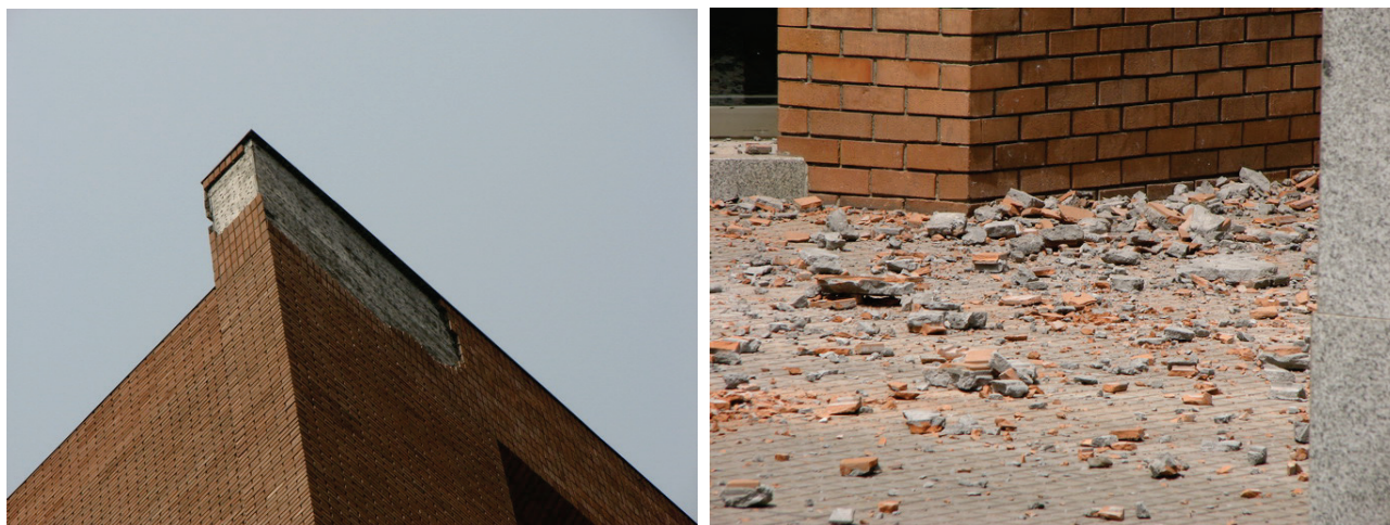
Figure 6.3.1.1-4 Failed adhered veneer fallen from parapet in Santiago following the 2010 magnitude-8.8 Chile Earthquake. (Photos courtesy of Antonio Iruretagoyena, Rubén Boroscheck & Associates)
