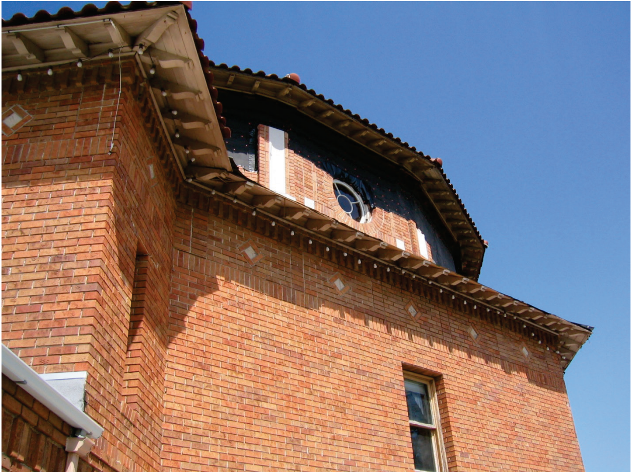
Figure 6.3.1.1-1 Failure of adhered masonry veneer at the Atascadero City Hall in the 2003 magnitude-6.5 San Simeon Earthquake (Photo courtesy of Mike Mahoney, FEMA).
