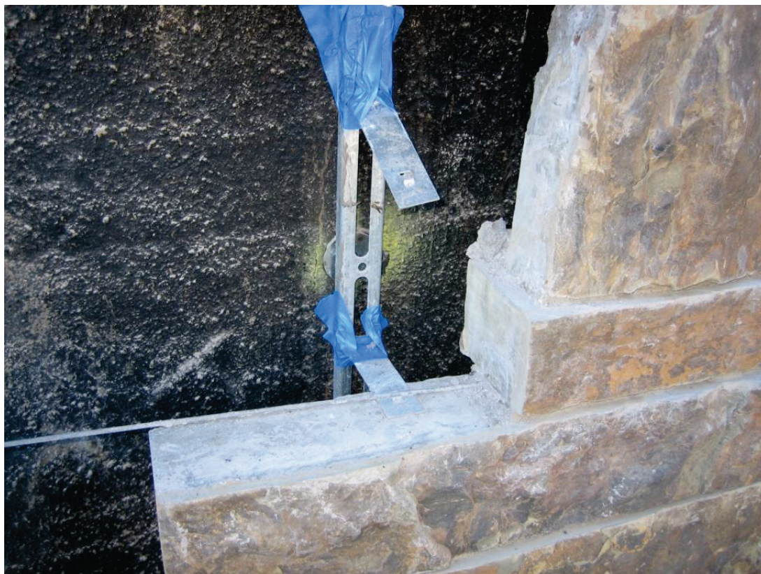
Figure 6.3.1.2-4 Installation of stone veneer showing anchorage to steel dovetail clips which are fastened to steel studs bolted to the grouted reinforced masonry wall behind (Photo courtesy of Simpson Gumpertz and Heger).
