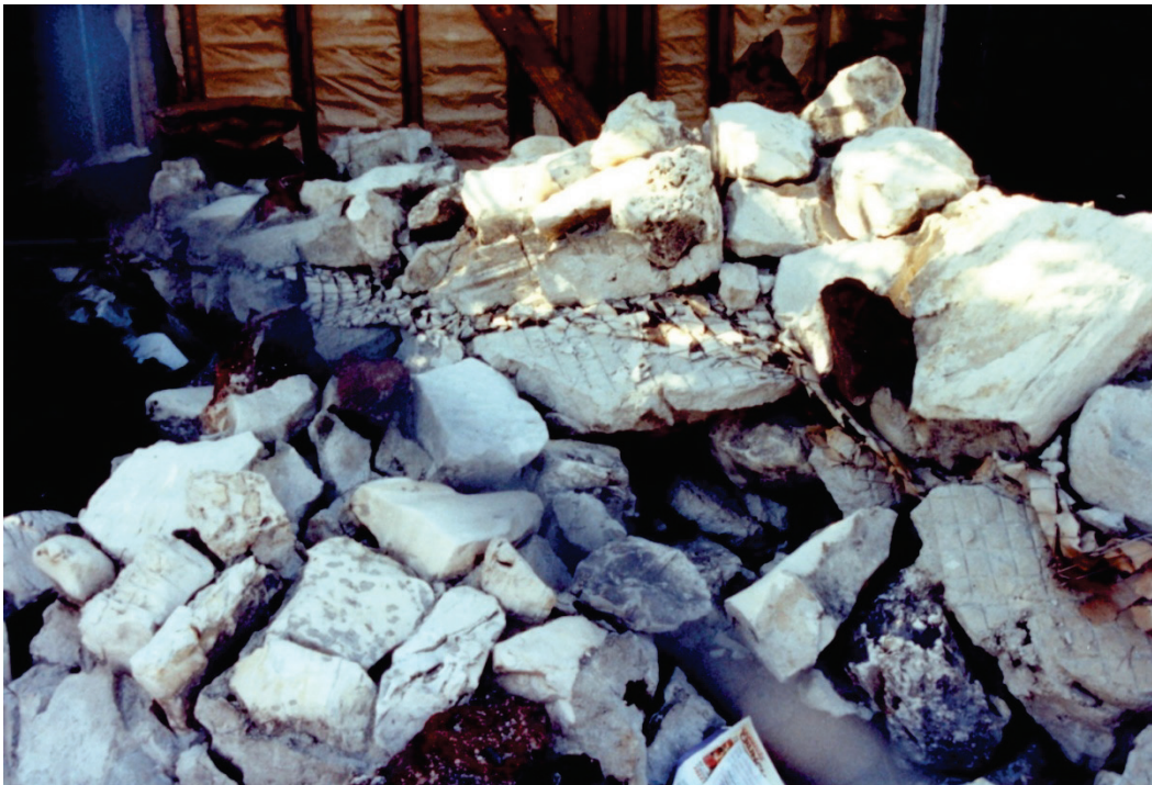
Figure 6.3.1.2-3 Rubble from failed anchored veneer as a result of the 1994 Northridge Earthquake (Photo courtesy of Robert Reitherman).
