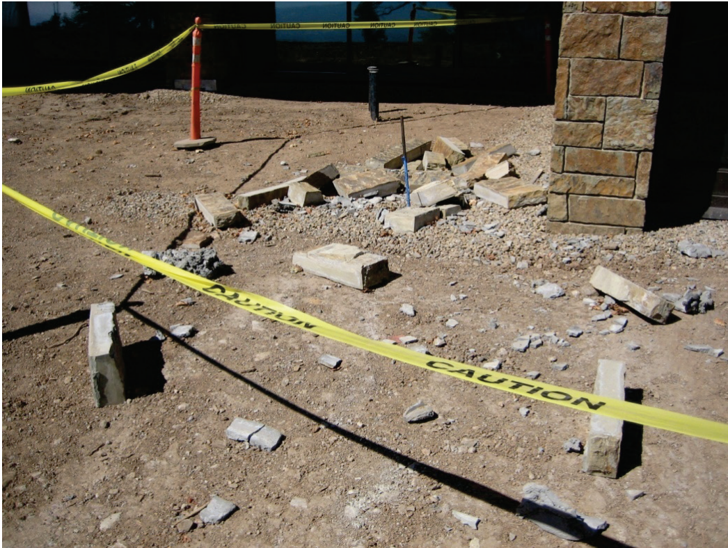
Figure 6.3.1.2-2 Fallen sandstone veneer as a result of a magnitude-4.4 earthquake (Photo courtesy of Simpson Gumpertz and Heger).
