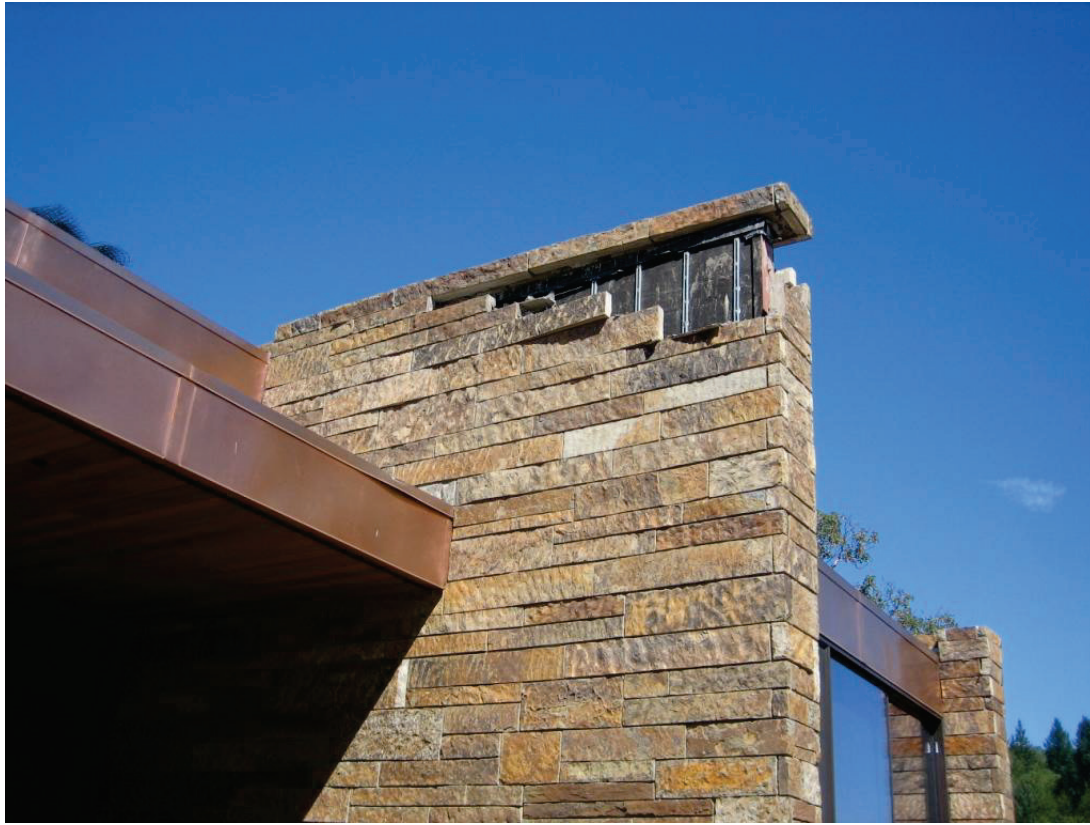
Figure 6.3.1.2-1 Fallen sandstone veneer as a result of a magnitude-4.4 earthquake in northern California. Post-earthquake investigation revealed missing dovetail anchors, missing pencil rods, and weak stone-to-mortar bond (Photo courtesy of Simpson Gumpertz and Heger).
