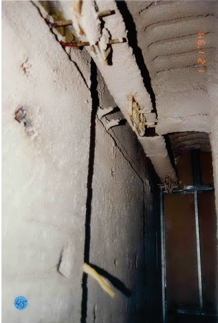
Figure 6.3.1.3-4 Interior view of precast panel showing response of three sets of push-pull connections in the 1994 Northridge Earthquake (Photo courtesy of OSHPD).
