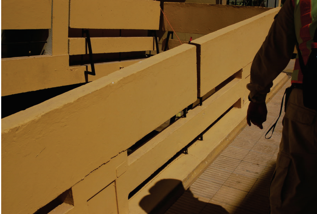
Figure 6.3.1.3-6 Residential building with precast concrete corridor and balcony railing panels. Some panels were damaged and subsequently many were removed to prevent falling. Location in Rancagua, Chile 154 miles northeast of the epicenter; estimated PGA of 0.3g during the 2010 magnitude-8.8 Chile Earthquake (Photo courtesy of Antonio Iruretagoyena, Rubén Boroscchek & Associates).
