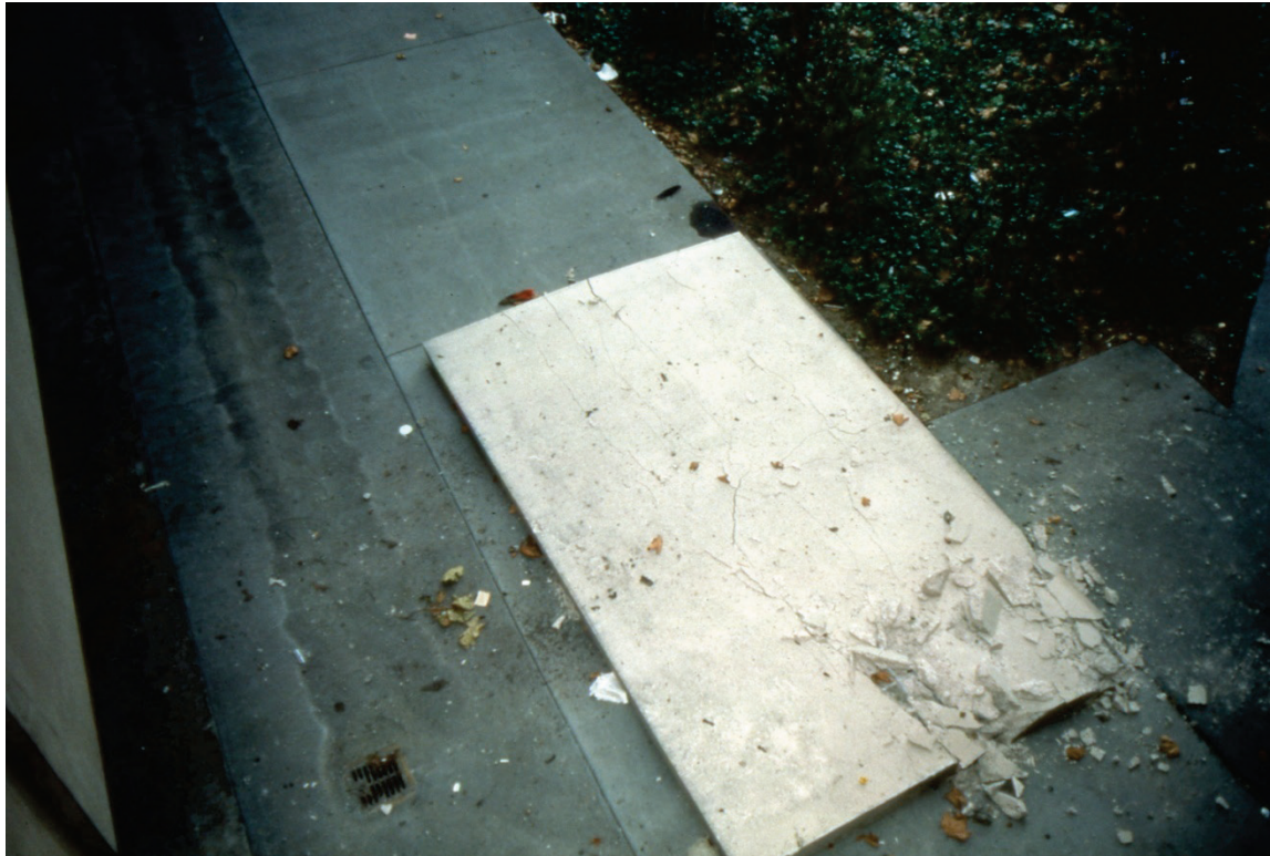
Figure 6.3.1.3-1 Failure of precast panel at parking garage that resulted in fatality in the 1987 magnitude-5.9 Whittier, California earthquake (Photo courtesy of Degenkolb Engineers).
