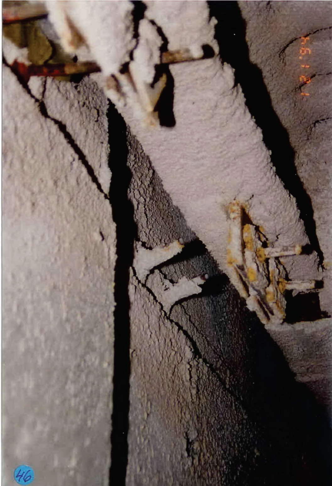
Figure 6.3.1.3-5 Close-up photo of two fractured connection bolts in a prefabricated panel in the 1994 Northridge Earthquake; corrosion of the rods may have contributed to the failure. (Photo courtesy of OSHPD).
