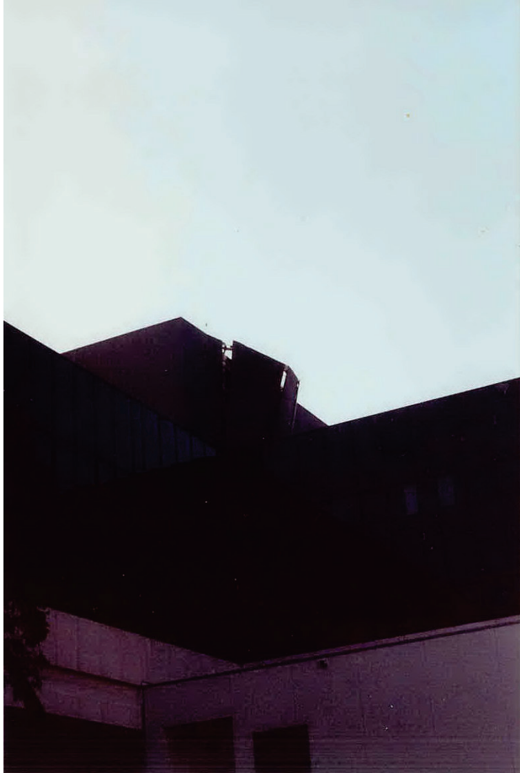
Figure 6.3.1.3-2 Precast panel failure at the top floor of a hospital in the 1994 magnitude-6.7 Northridge Earthquake (Photo courtesy of OSHPD).
