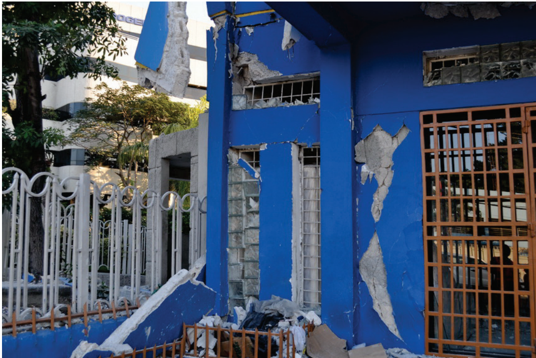
Figure 6.3.1.5-1 Damage to glass block in building with reinforced concrete frame and concrete masonry infill in the magnitude-7 2010 Haiti Earthquake (Photo courtesy of Eduardo Fierro, BFP Engineers). Note some blocks failed at rigid mortar joints and stayed in the frame, others fell out of the frame, and others broke in place. This building also suffered structural damage.
