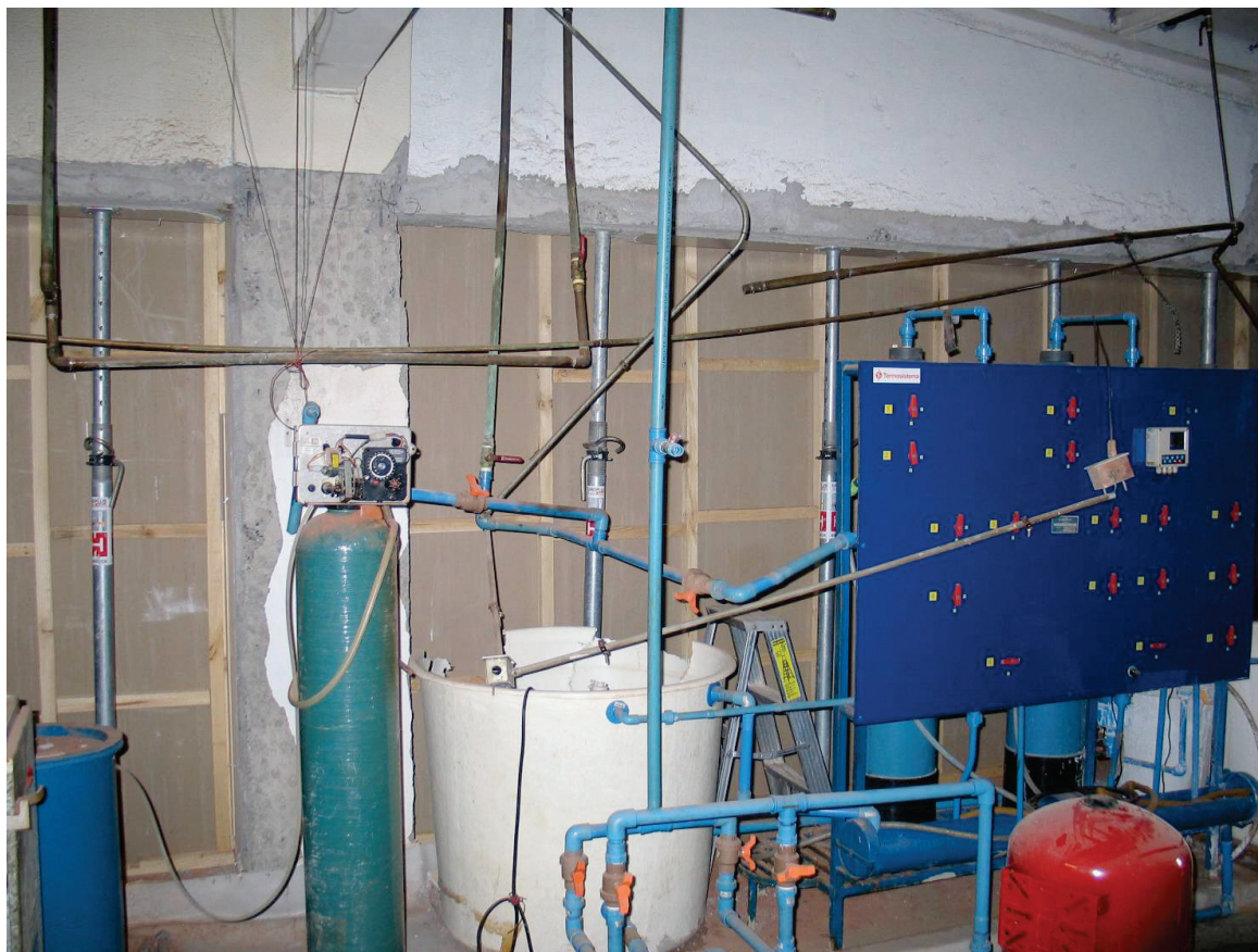
Figure 6.3.2.1-6 An infill masonry wall collapsed onto the distilled water equipment spilling two 150 gallon containers; water leaked past the perimeter edge of the floor slab into the operating room suite below resulting in the closure of 3 of 6 the operating rooms. Replacement gypsum board partition seen in photo. Hospital built in 2005 in Los Angeles, Chile. Damage from the 2010 Chile Earthquake (Photo courtesy of Bill Holmes, Rutherford & Chekene).
