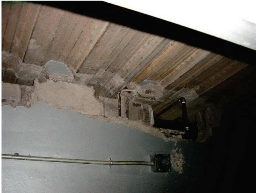
Figure 6.3.2.1-1 Damage along the top of a reinforced concrete masonry unit partition built flush with soffit of metal deck at an industrial facility in the 2001 magnitude-8.4 Peru Earthquake (Photo courtesy of Eduardo Fierro, BFP Engineers).
