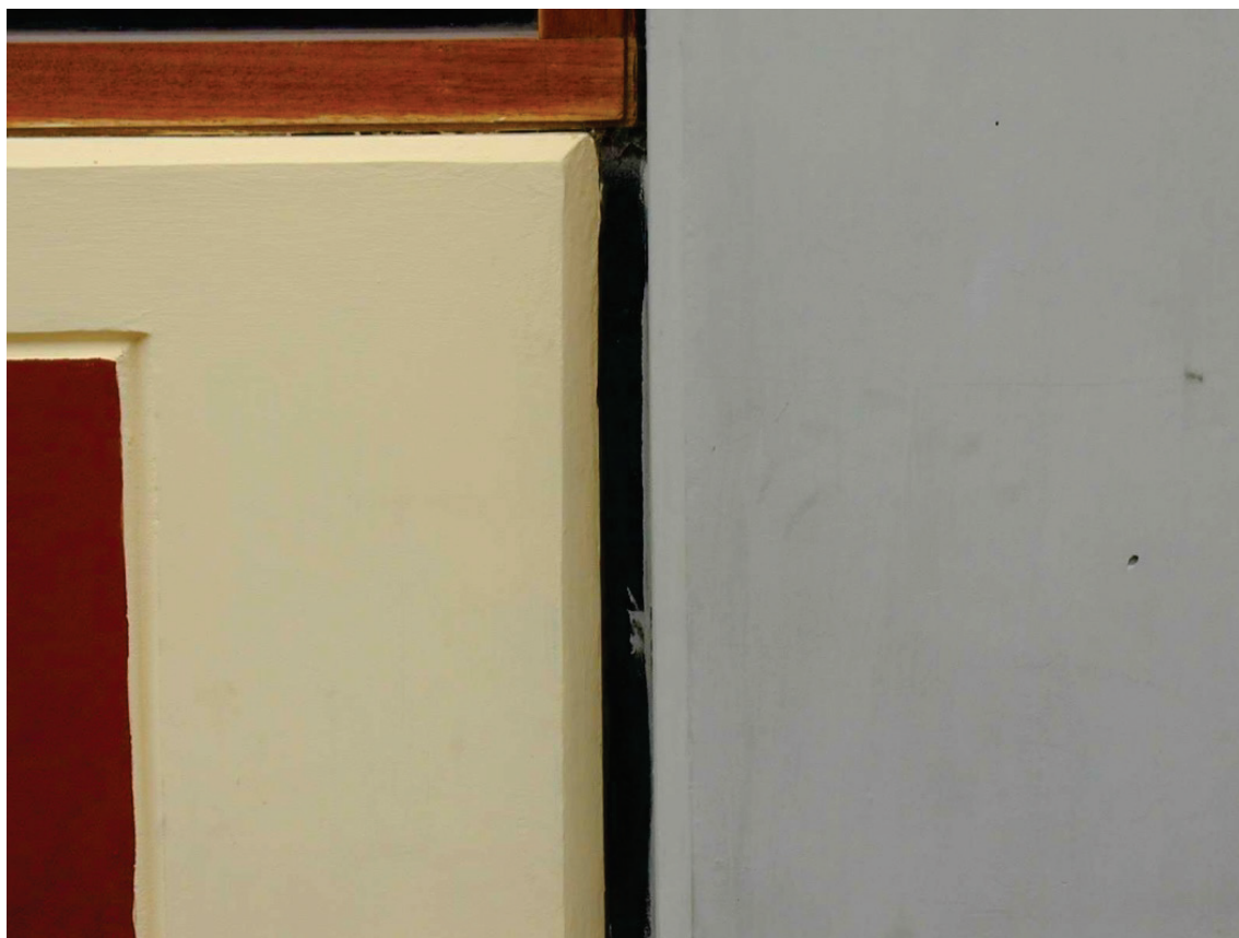
Figure 6.3.2.1-7 Detail of isolation joint to prevent creation of “captive column” condition (Photo courtesy of Eduardo Fierro, BFP Engineers).
