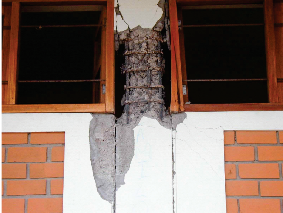
Figure 6.3.2.1-3 Damage to structural column (“captive column”) due to restraint caused by partial height masonry wall in the 2001 Peru Earthquake (Photo courtesy of Eduardo Fierro, BFP Engineers).
