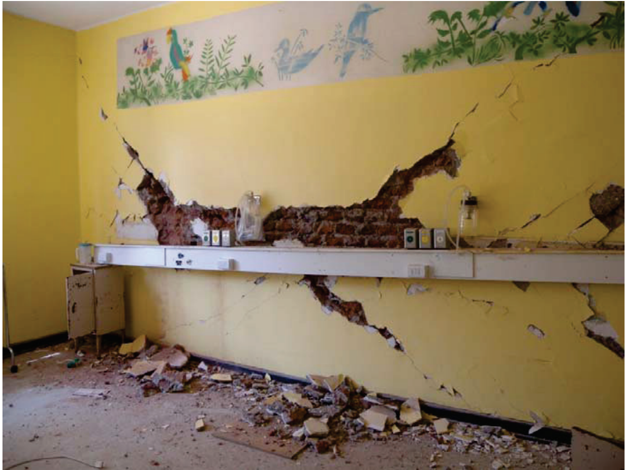
Figure 6.3.2.1-5 Damage to unreinforced brick partitions in patient rooms, and other mostly nonstructural damage, resulted in the evacuation of the Felix Bulnes Hospital in Santiago in the 2010 magnitude-8.8 Chile Earthquake (Photo courtesy of Gilberto Mosqueda, University of Buffalo, SUNY).
