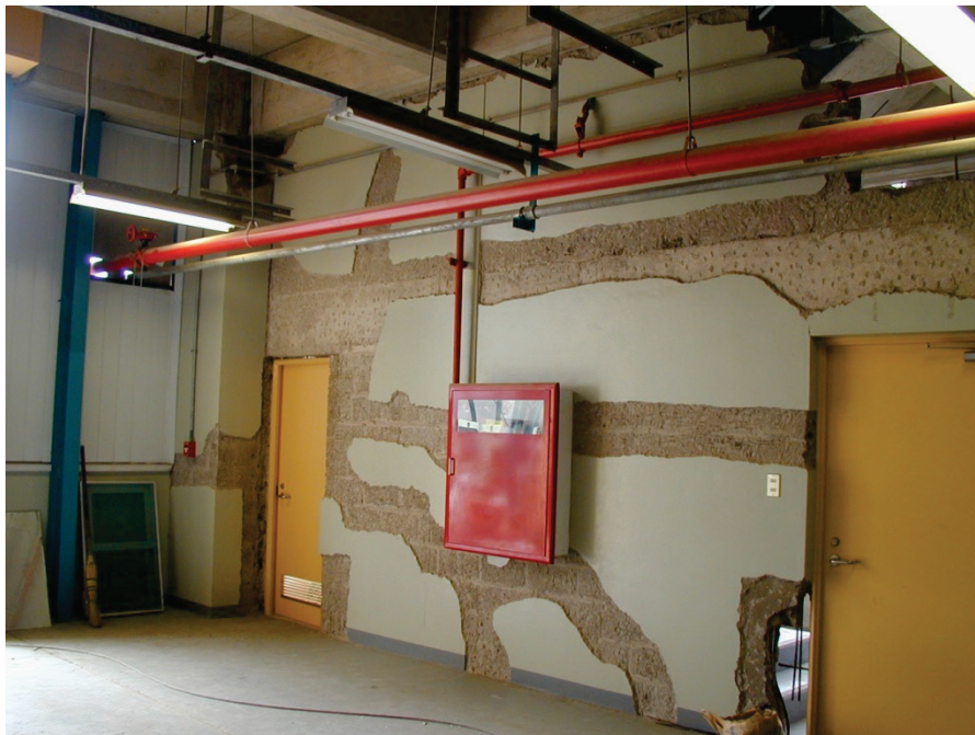
Figure 6.3.2.1-2 Damage to reinforced concrete masonry partition used to support fire protection cabinet and piping in the 2001 Peru Earthquake; loose stucco and masonry were removed prior to photo (Photo courtesy of Eduardo Fierro, BFP Engineers).
