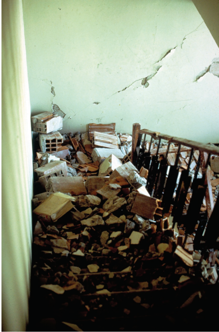
Figure 6.3.2.1-4 View of stairway in the Banco Central Building, Managua, Nicaragua after the 1972 magnitude 6.2 Managua Earthquake. Most of the stairs were covered with debris that resulted from the failure of the hollow tile partitions surrounding the stairs (Photo courtesy of PEER Godden Collection, No. J94).
