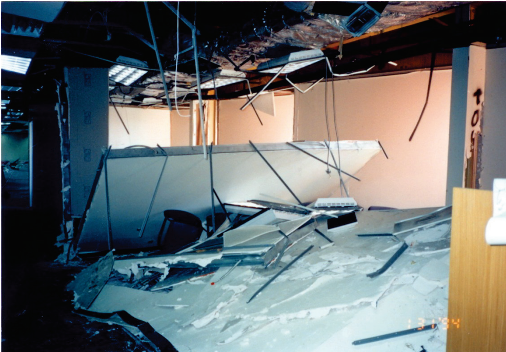
Figure 6.3.2.2-1 Out-of-plane failure of inadequately braced partial height metal stud partitions in the 1994 Northridge Earthquake (Photo courtesy of Wiss, Janney, Elstner Associates).
