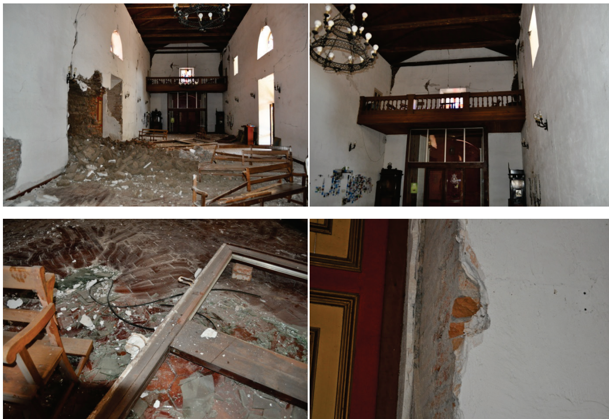
Figure 6.3.2.3-3 Failed wood framed glazing assembly in the 2010 Chile earthquake (Photo courtesy of Eduardo Fierro, BFP Engineers). The wood framing was held in place by metal or rebar brackets embedded in the masonry wall. The adobe wall on the left of the door collapsed and the brackets on the right side pulled out of the brick masonry wall (lower right). The glazing assembly at the rear entrance of the chapel was anchored overhead to the wood balcony framing and was undamaged.
