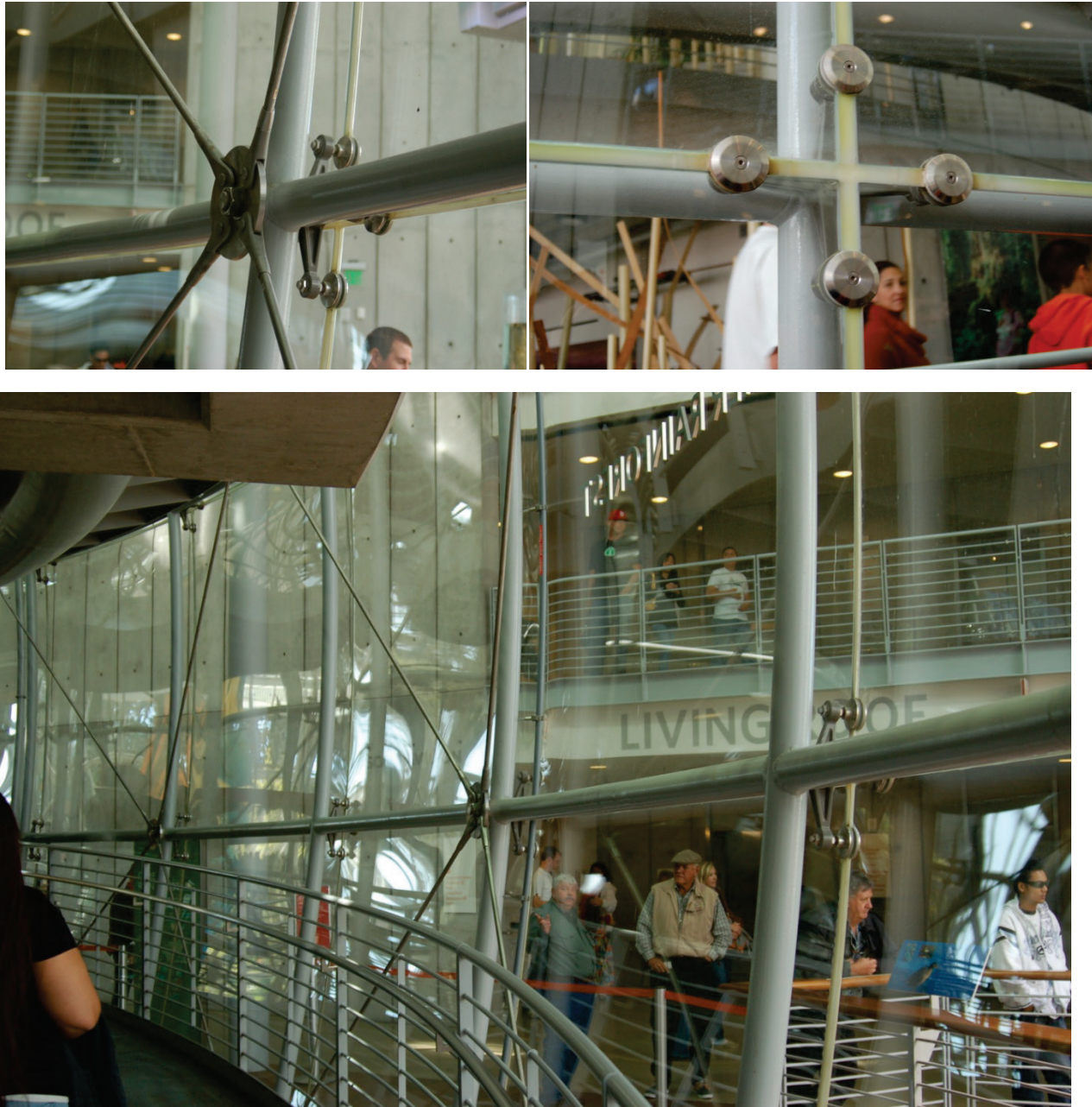
Figure 6.3.2.3-5 Specialized glazing details for glass dome using specialty hardware, such as large sealant joints required to accommodate thermal movement and seismic deformations at the California Academy of Sciences, San Francisco, California (Photos courtesy of Cynthia Perry, BFP Engineers).
