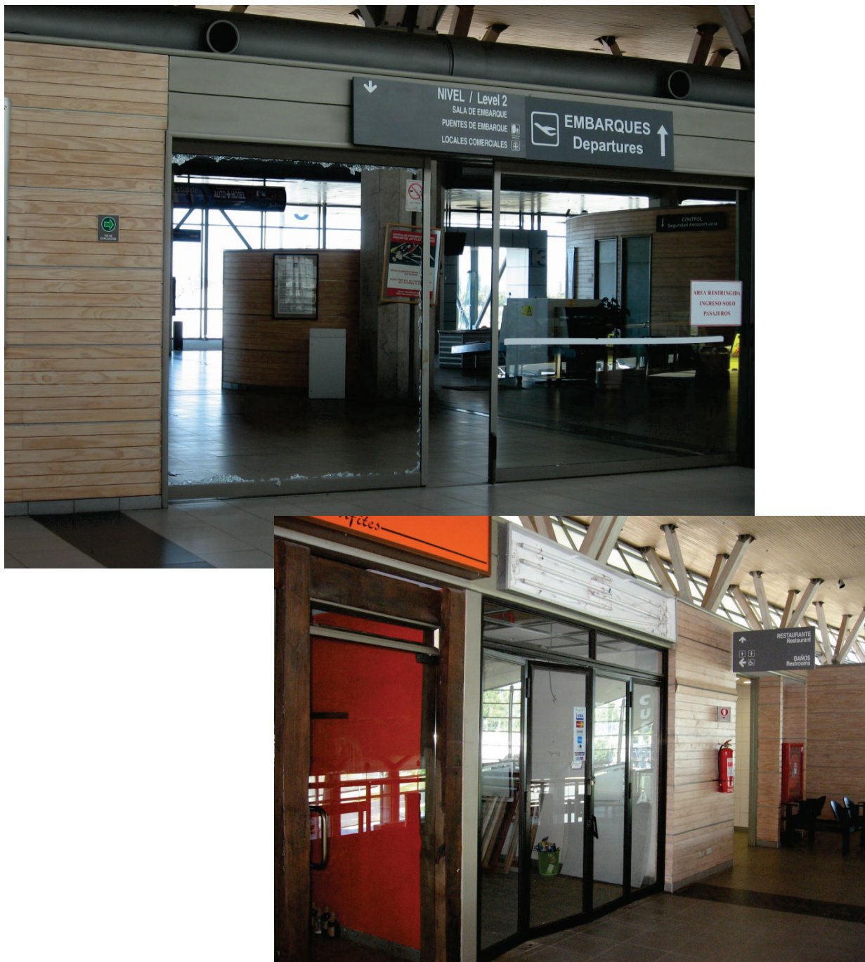
Figure 6.3.2.3-2 Damage to glazed doors at the Concepción airport in the 2010 Chile Earthquake. In the top photo the glazing in the sliding glass door shattered; in the lower photo the glass is intact but the door frames are misaligned (Photos courtesy of Rodrigo Retamales, Rubén Boroschek & Associates).
