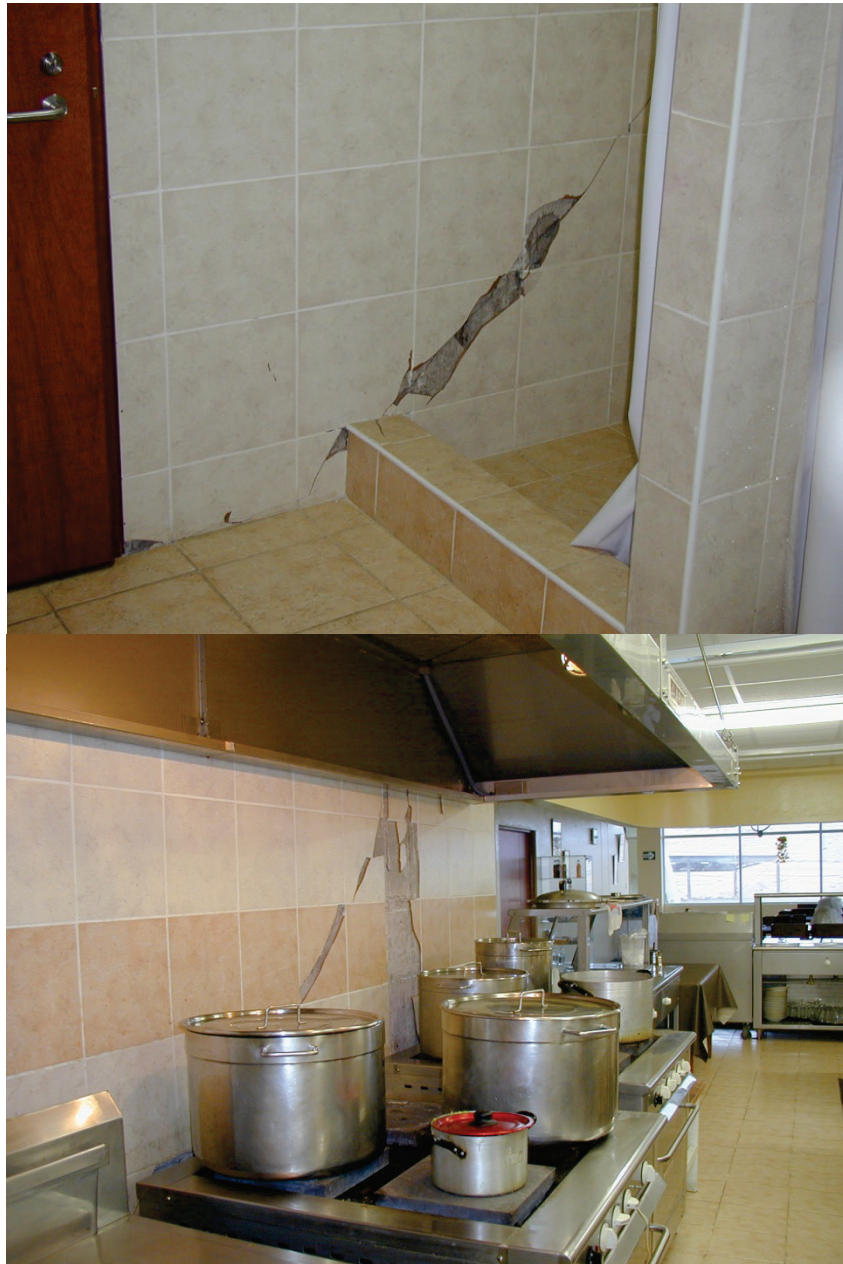
Figure 6.3.3.1-2 Damage to adhered tile veneer in locker room and kitchen at industrial facility in the 2001 Peru Earthquake (Photo courtesy of Eduardo Fierro, BFP Engineers). Tile was adhered to CMU partitions which were built integral with the concrete frame. While only a limited number of tiles were broken, equipment had to be disconnected and many tiles removed to repair cracks in the wall and facilitate the repair of the veneer.
