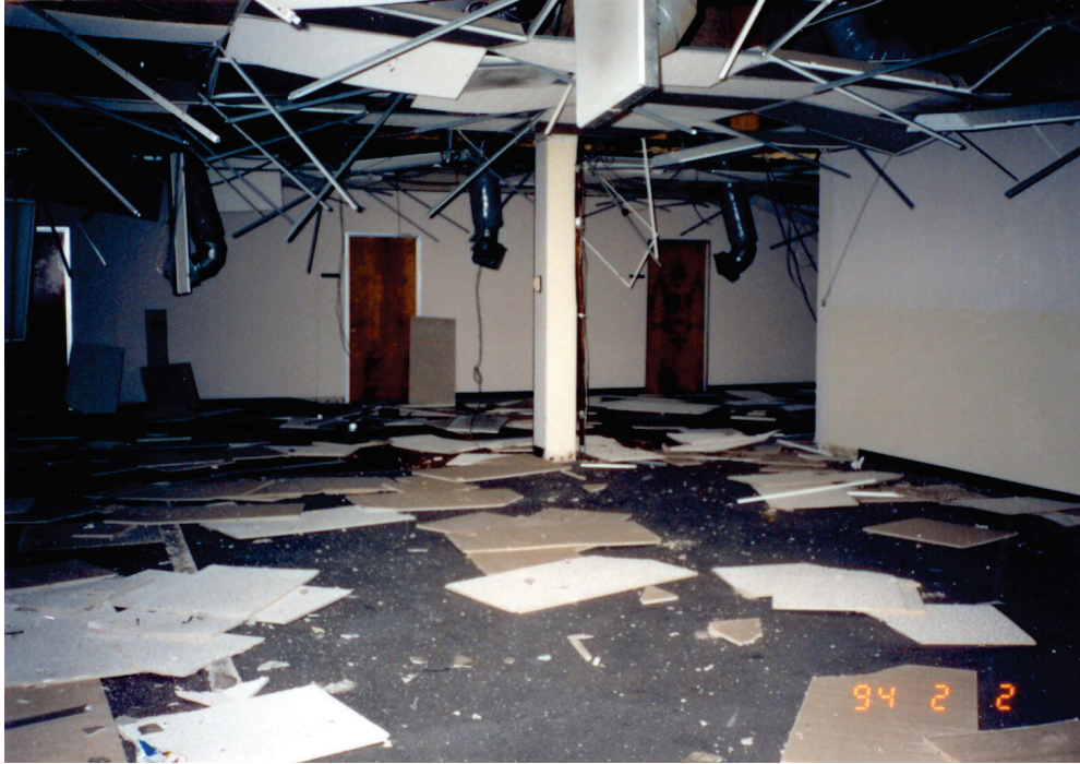
Figure 6.3.4.1-2 Failure of suspended ceiling system including lights and air diffusers in the 1994 Northridge Earthquake (Photo courtesy of Wiss, Janney, Elstner Associates).
