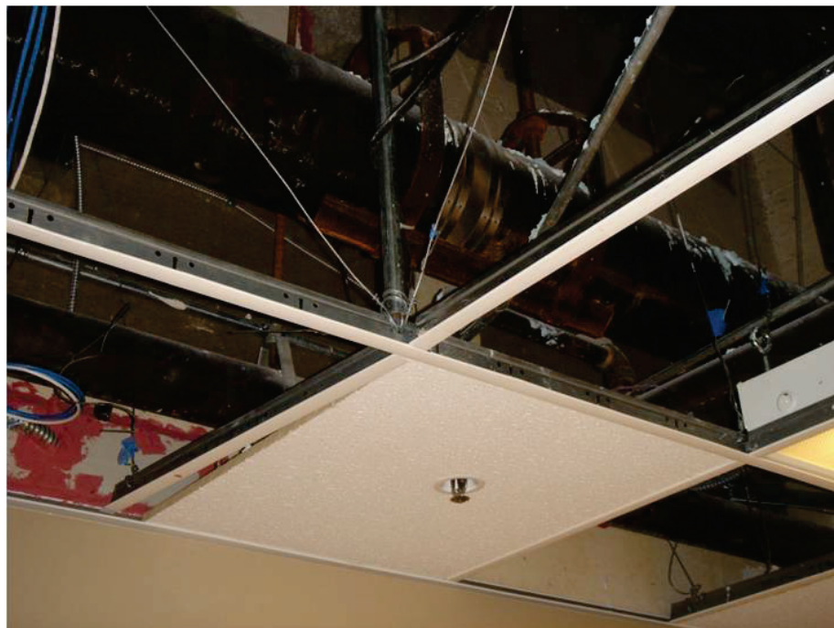
Figure 6.3.4.1-6 Compression struts and diagonal splayed wires are used to limit the movement of suspended acoustic tile ceilings. Per ASTM E580, this type of bracing assembly is required for ceiling areas larger than 1000 sq. ft. in Seismic Design Category D,E, and F (Photo courtesy of Maryann Phipps, Estructure).
