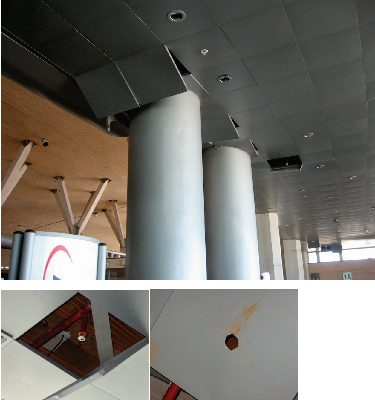
Figure 6.3.4.1-5 Damage to suspended metal panel ceiling system and fire sprinklers at Concepción airport, primarily at far end and around column obstructions in the 2010 Chile Earthquake (Photos courtesy of Rodrigo Retamales, Rubén Boroschek & Associates). The metal panel was strong enough to fail the sprinkler head shown at lower left.
