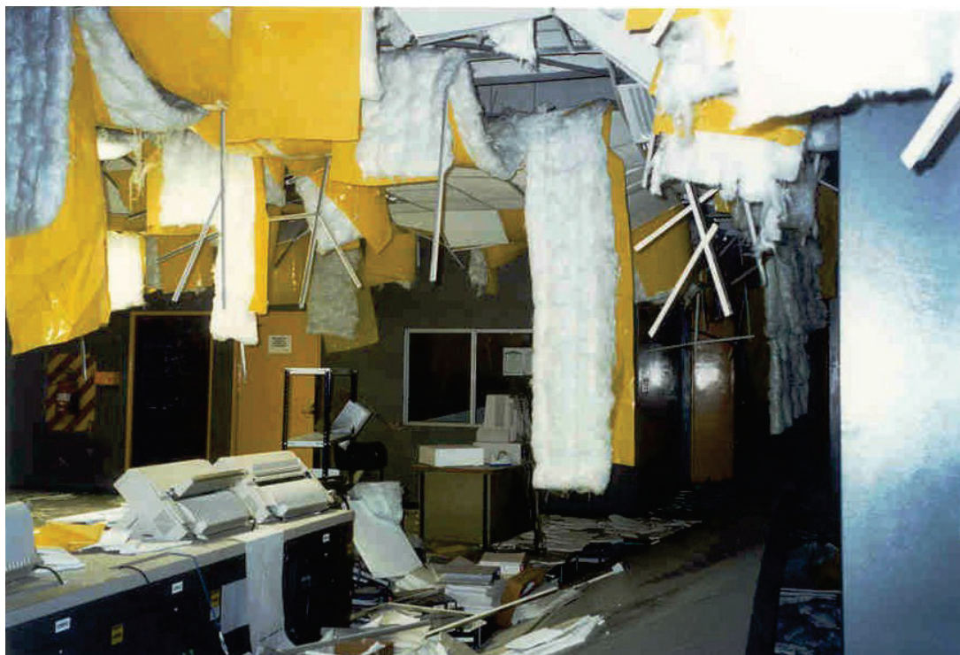
Figure 6.3.4.1-1 Failure of suspended ceiling system including lights, air diffusers, and insulation in control room of an industrial plant in the 2001 magnitude-8.4 Peru Earthquake (Photo courtesy of BFP Engineers).
