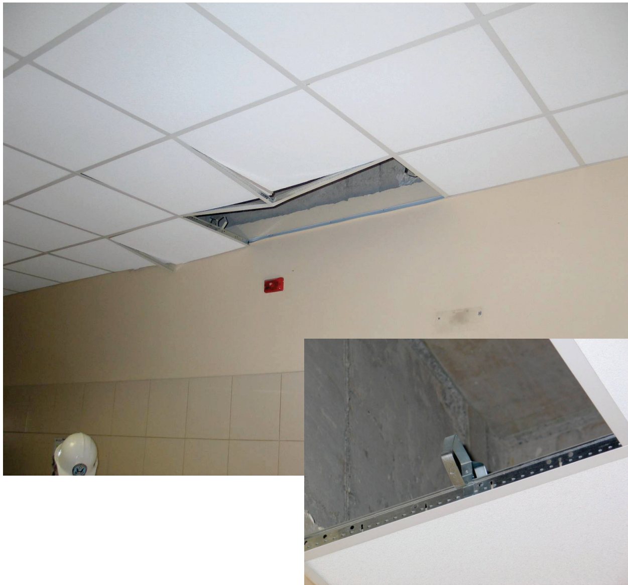
Figure 6.3.4.1-4 Fallen ceiling tiles at Talca Hospital in the 2010 Chile Earthquake, in spite of the use of clips as shown in detail at right. Most ceilings observed in Chile did not have seismic detailing (Photos courtesy of Bill Holmes, Rutherford & Chekene).
