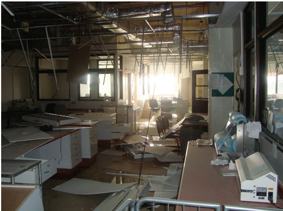
Figure 6.3.4.1-3 Generalized failure of ceiling grid, tiles, lights, and diffusers at the Los Angeles Hospital in the 2010 magnitude-8.8 Chile Earthquake (Photo courtesy of Bill Holmes, Rutherford & Chekene).
