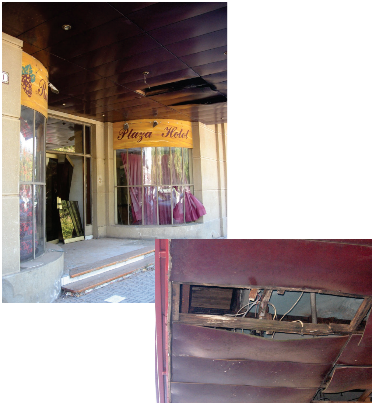
Figure 6.3.4.2-3 Damage to soffit paneling and wood framing at hotel in the 2010 Chile Earthquake; panels and wood framing show signs of prior water damage and deterioration. Note also damage to storefront glazing and glass doors (Photos courtesy of Rodrigo Retamales, Rubén Boroschek & Associates).
