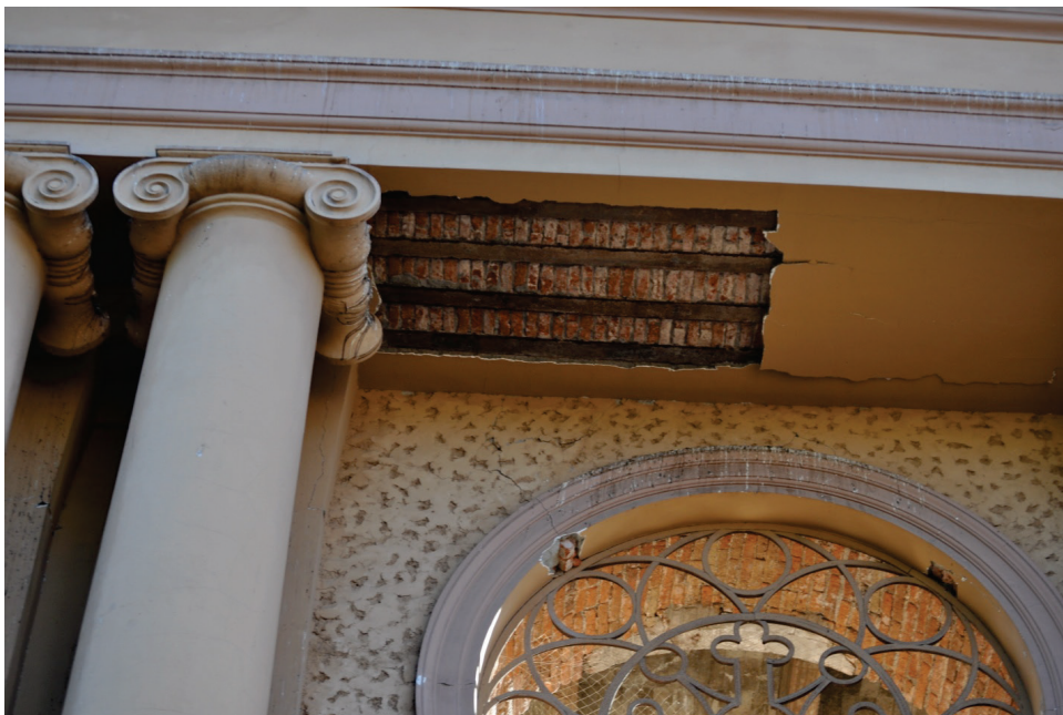
Figure 6.3.4.2-2 Damage to stucco soffit of historic church in the 2010 Chile Earthquake (Photo courtesy of Eduardo Fierro, BFP Engineers). Stucco applied directly to the underside of the slab above without furring; portion at left has fallen, portion at right delaminated.
