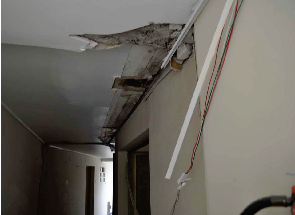
Figure 6.3.4.2-1 Damage to metal lath and plaster ceiling applied to the underside of the concrete slab in 10-story residential building in the 2010 magnitude-8.8 Chile Earthquake (Photo courtesy of Eduardo Fierro, BFP Engineers). The damage occurred due to pounding at the interface between two wings of the structure.
