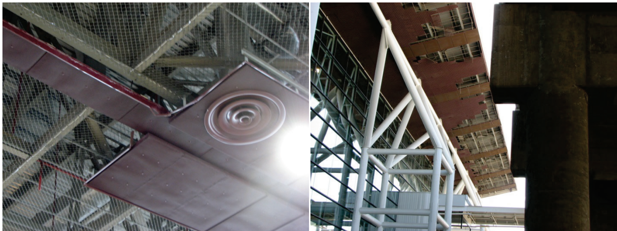
Figure 6.3.4.2-5 Extensive failure of ceiling in the main terminal of the Santiago airport in the 2010 Chile Earthquake. Metal panels with lights and diffusers hung from furring on short metal tabs; these remained in place but detail at lower left shows they also sustained some damage. Furring channels still in place throughout ceiling but majority of lightweight ceiling panels and much of the cross furring came down as shown at lower right photo of exterior soffit with same system (Photos courtesy of Antonio Iruretagoyena, Rubén Boroscchek & Associates).
