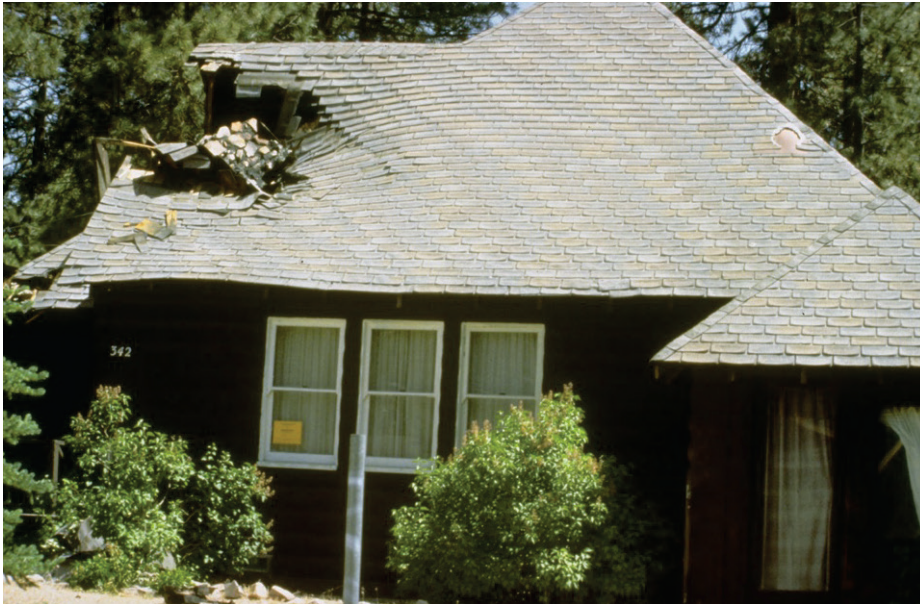
Figure 6.3.7.1-1 Chimney collapsed and fell through the roof; approximately 2,600 chimneys were destroyed in the 1992 Big Bear City, California earthquake (NGDC, 2009).
