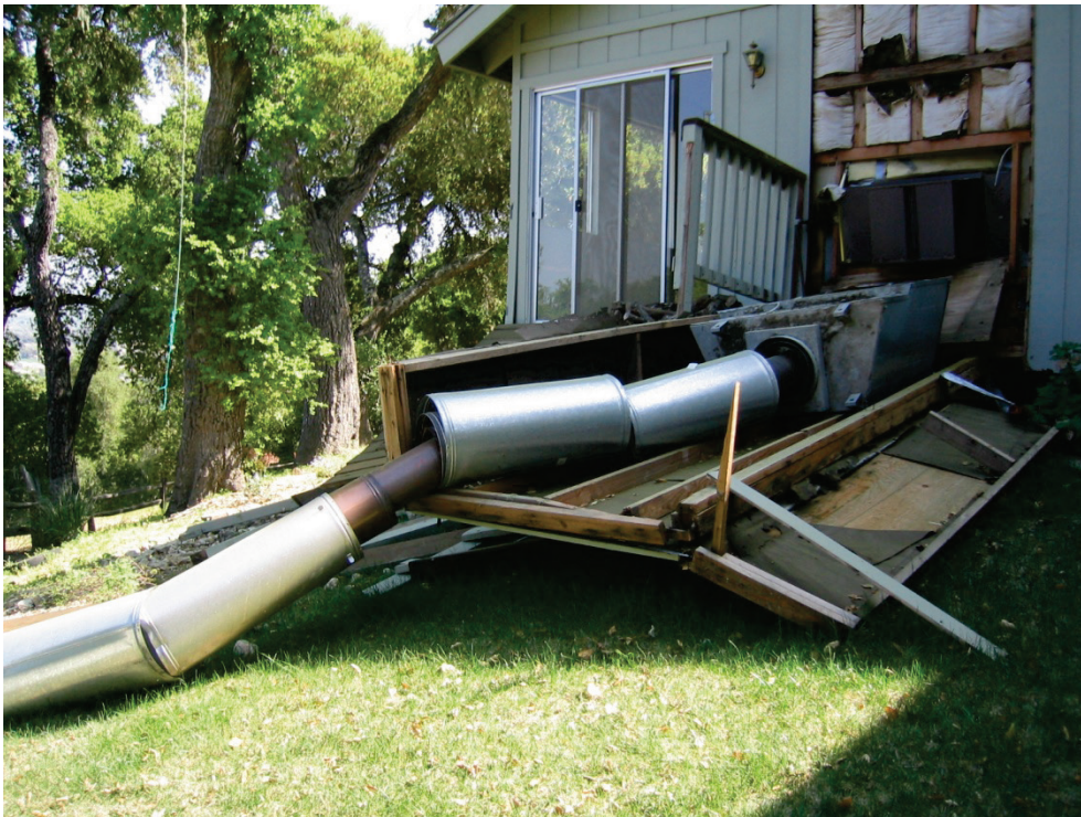
Figure 6.3.7.1-2 Residential metal flue in wood frame chimney that failed in the 2003 magnitude-6.5 San Simeon earthquake. The house fell off its cripple wall, pushing over the chimney (Photo courtesy of Michael Mahoney).
