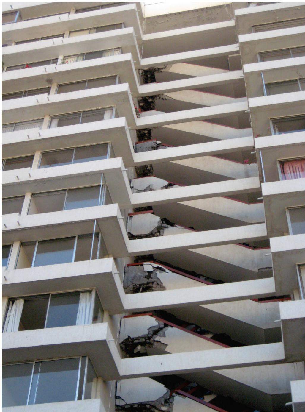
Figure 6.3.8.1-3 Stairs damaged up the full height of this apartment building in Viña del Mar in the 2010 magnitude-8.8 Chile Earthquake (Photo courtesy of Santiago Pujol, Purdue University). The stairs were rigidly attached at adjacent floors and behaved like diagonal braces although they were neither designed nor detailed to function as structural braces.
