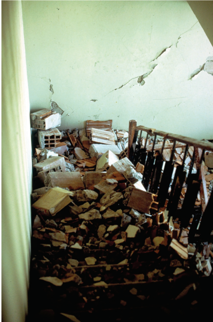
Figure 6.3.8.1-2 View of stairway in the Banco Central Building, Managua, Nicaragua after the 1972 magnitude-6.2 Managua Earthquake. Most of the stairs were covered with debris that resulted from the failure of the hollow tile partitions surrounding the stairs. This photograph highlights the need to not only prevent direct damage to stairway framing and connections, but also to protect against damage to surrounding walls (Photo courtesy of PEER Godden Collection, No. J94).
