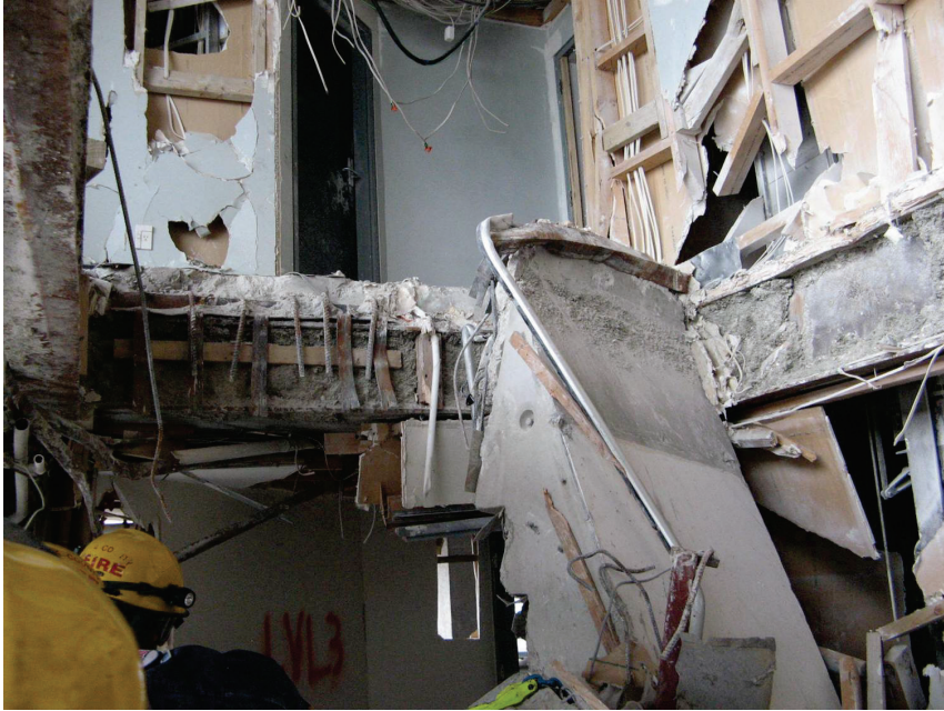
Figure 6.3.8.1-4 Stair support condition at Forsyth-Barr Building in Christchurch, New Zealand. Precast stair runs have completely pulled off supports and collapsed into stairwell (Photo courtesy of Des Bull, Holmes Consulting Group).
