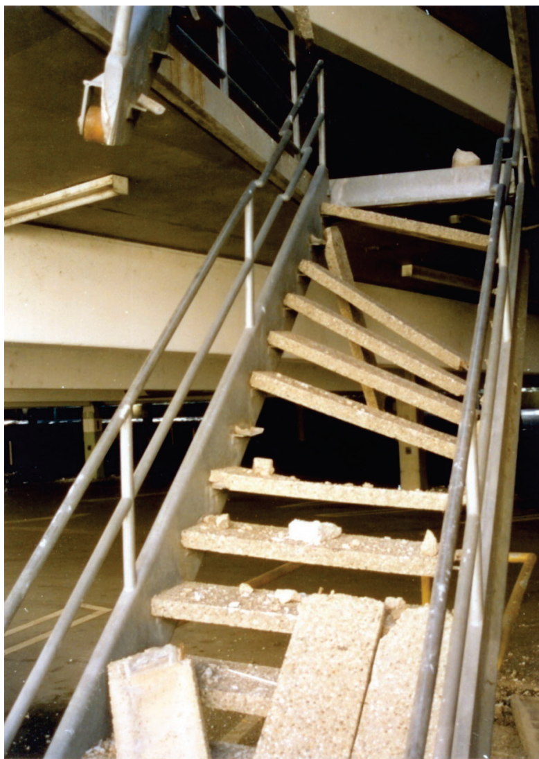
Figure 6.3.8.1-1 Stairway damaged by drift in the 1994 magnitude-6.7 Northridge, California earthquake (Photo courtesy of Wiss, Jenney, Elstner Associates).
