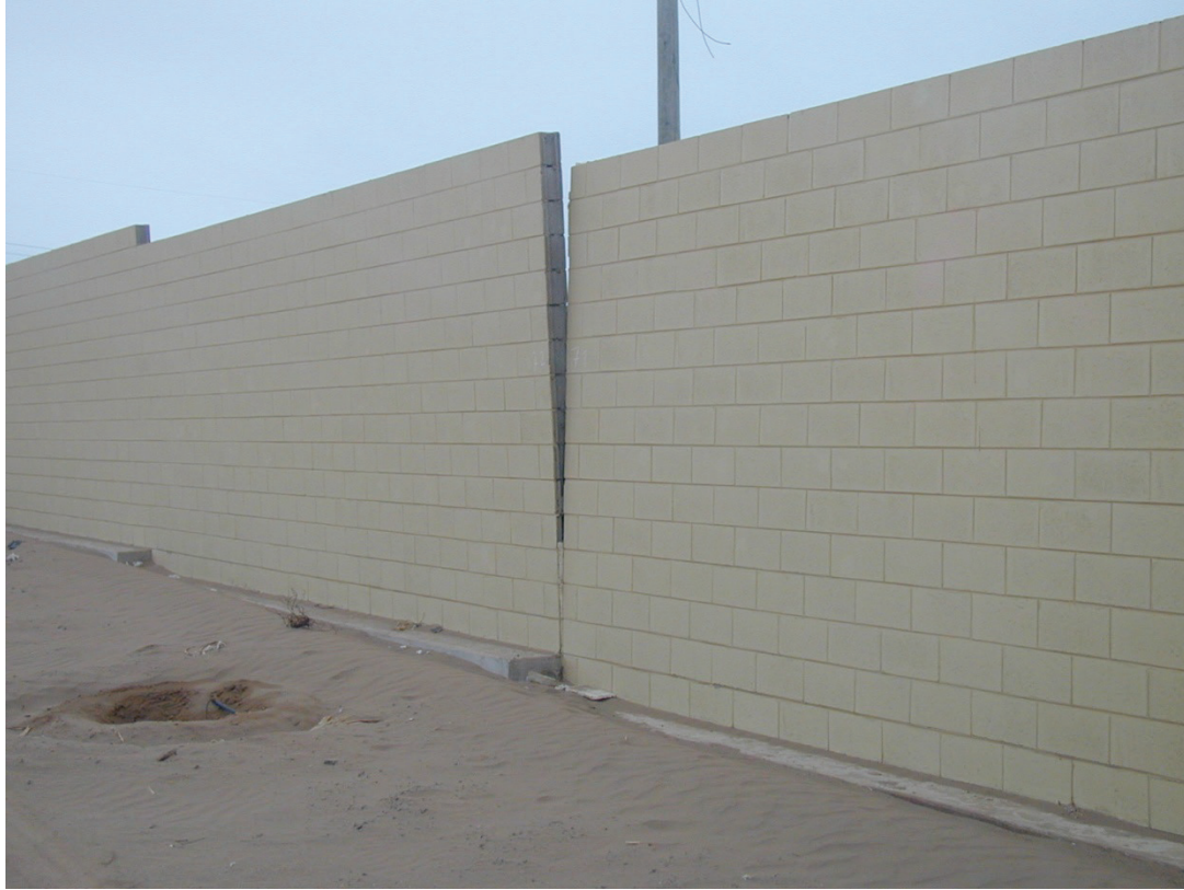
Figure 6.3.9.1-3 Damage to reinforced masonry boundary fence at industrial facility in Southern Peru; out-of-plane movement at construction joint in wall without sufficient reinforcing for the level of shaking experienced at this location in the 2001 magnitude-8.4 Peru Earthquake (Photo courtesy of Eduardo Fierro, BFP Engineers). Additional boundary steel or reinforced concrete boundary columns located either side of construction joints would improve the performance of this type of fence.
