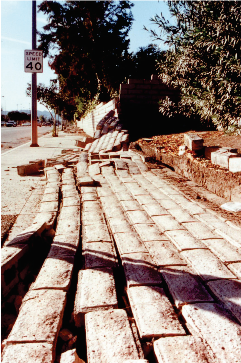
Figure 6.3.9.1-1 Collapse of freestanding CMU walls covering much of the sidewalk in the 1994 magnitude-6.7 Northridge Earthquake (Photo courtesy of Robert Reitherman). The rubble reveals that the wall was unreinforced.
