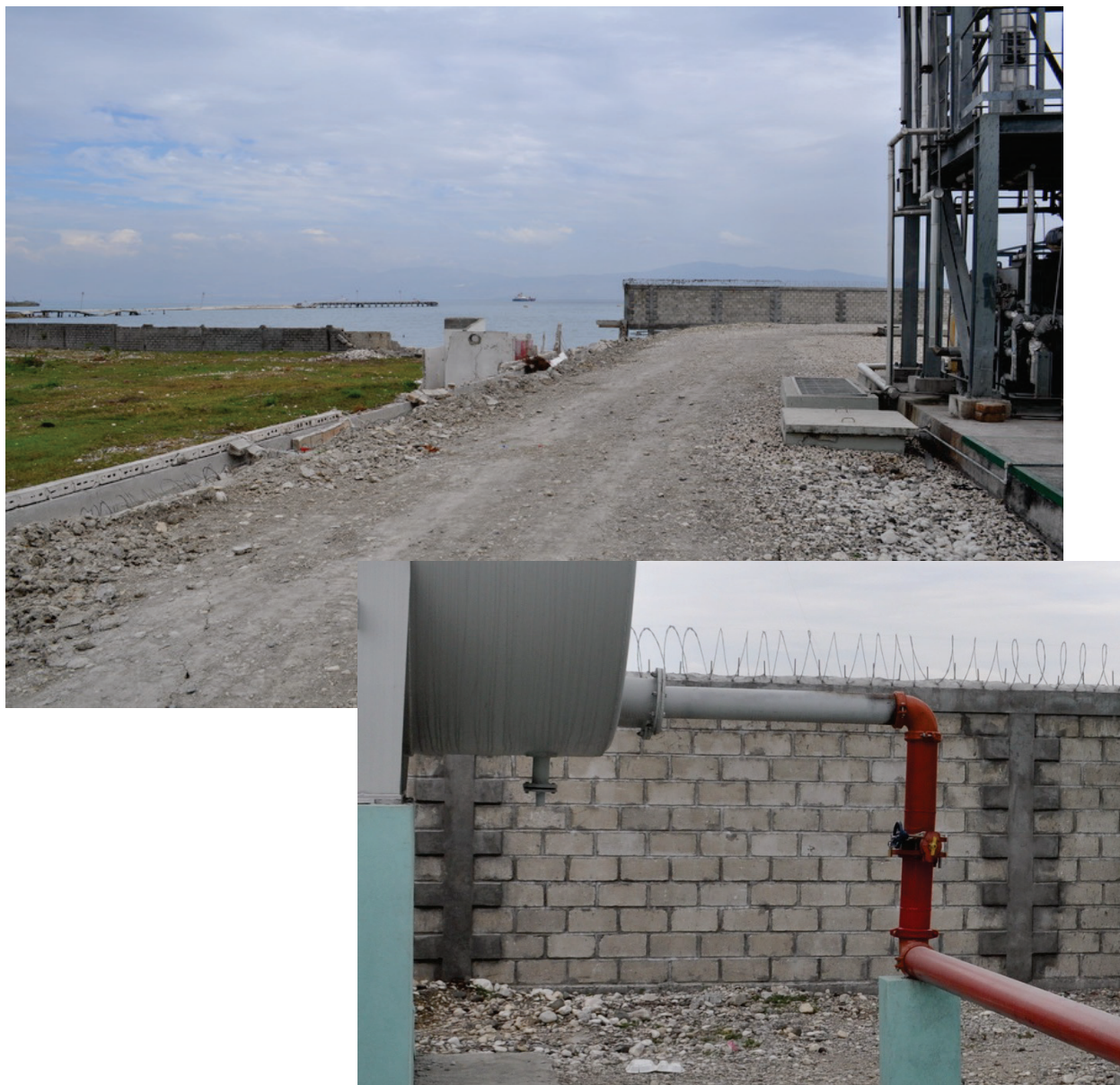
Figure 6.3.9.1-4 Photo at top shows complete collapse of poorly detailed confined masonry fence in foreground; partial collapse of poorly detailed confined masonry fence in distance at left; no damage to well detailed confined masonry fence in distance at right in the 2010 Haiti Earthquake. Close-up view of well-detailed confined masonry fence in bottom photo with concrete columns and bond beam at top (Photos courtesy of Eduardo Fierro, BFP Engineers). Fences in foreground and at right formed the security perimeter at an electric power plant in Port-au-Prince.
