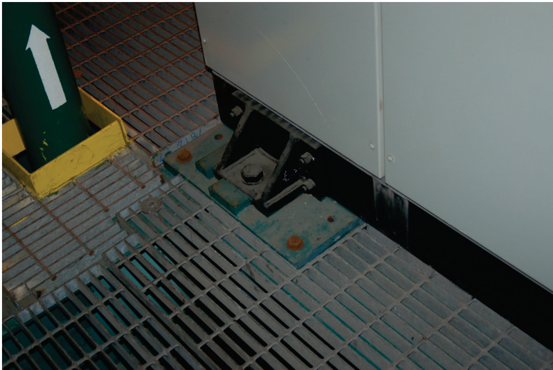
Figure 6.4.1.1-4 Bolted connection to steel skid with added shear lugs (Photo courtesy of Eduardo Fierro, BFP Engineers).
