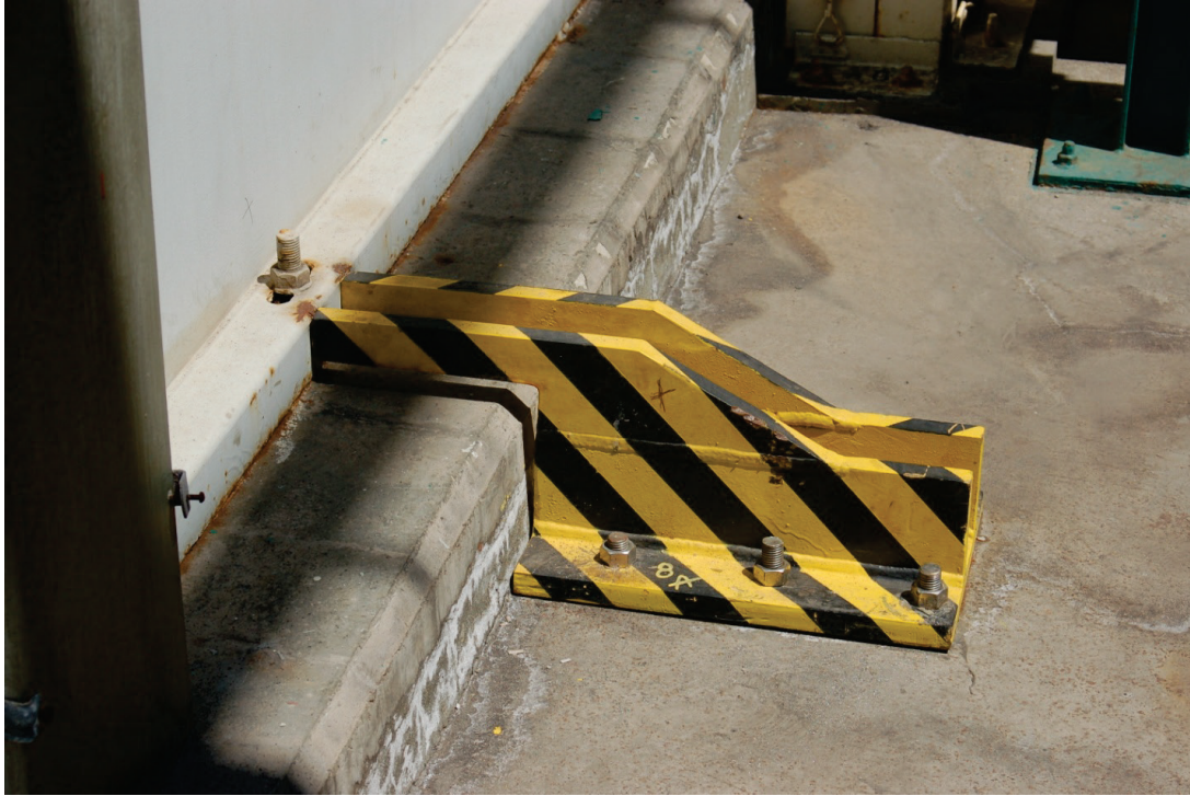
Figure 6.4.1.1-3 Added lateral capacity provided for skid-mounted equipment added following the 2001 Peru Earthquake (Photo courtesy of Eduardo Fierro, BFP Engineers).
