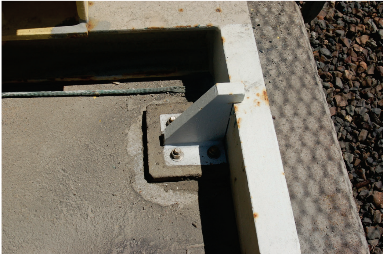
Figure 6.4.1.1-5 Alternate detail for skid mounted equipment (Photo courtesy of Eduardo Fierro, BFP Engineers).
