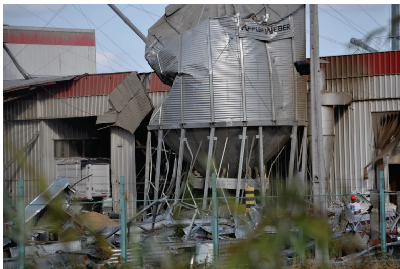
Figure 6.4.1.2-2 Damage to silos, conveyors and equipment at a grain operation in the 2010 magnitude-8.8 Chile Earthquake (Photos courtesy of Eduardo Fierro, BFP Engineers).
