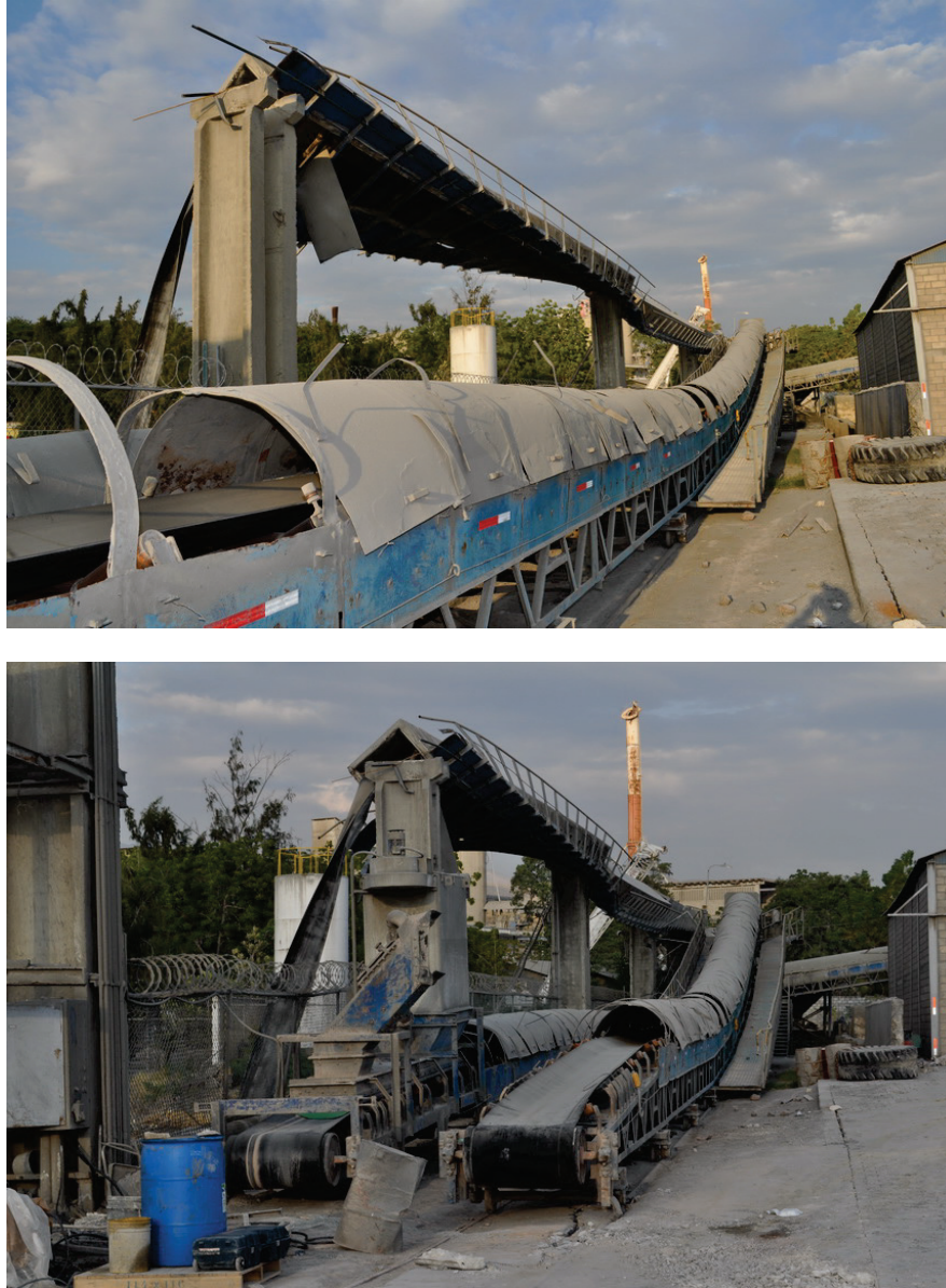
Figure 6.4.1.2-1 Damage to conveyors and equipment at a cement plant in the 2010 magnitude-7 Haiti Earthquake (Photos courtesy of Eduardo Fierro, BFP Engineers).
