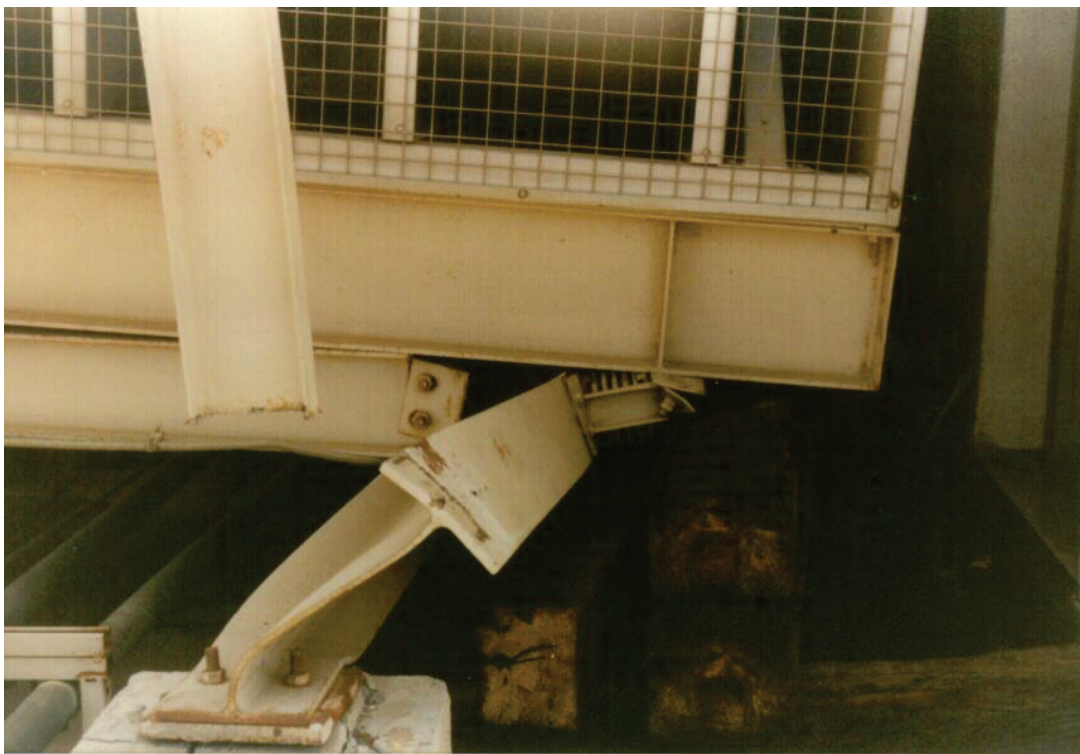
Figure 6.4.1.3-3 Failure of an entire support assembly including vibration isolators (Photo courtesy of Mason Industries).
