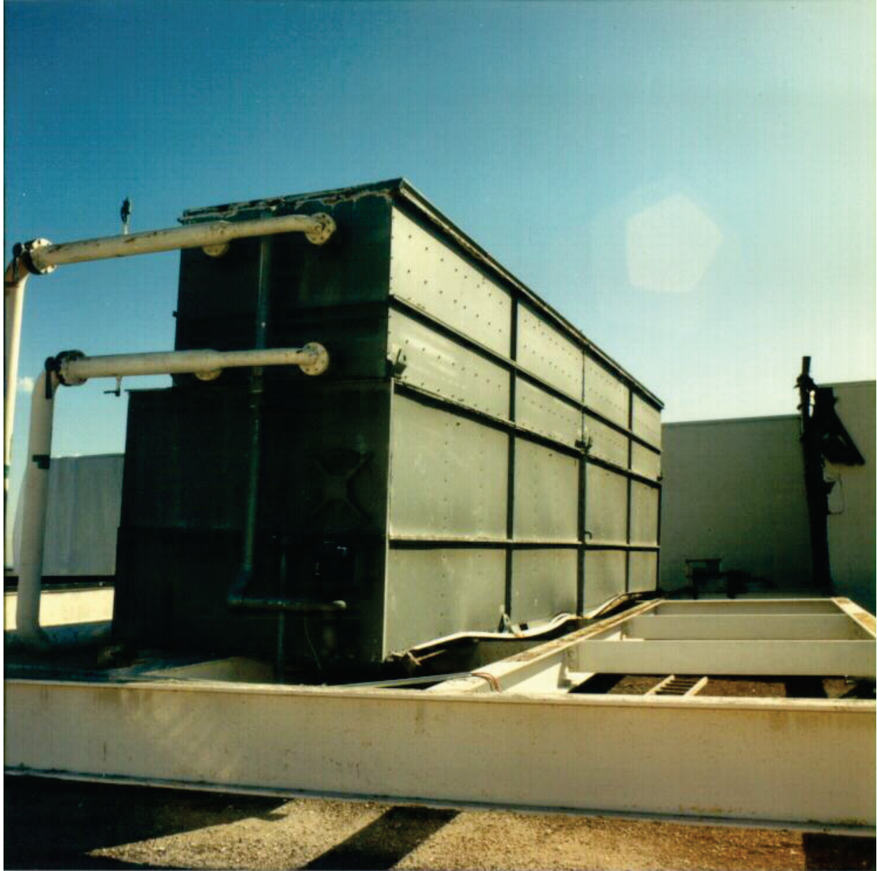
Figure 6.4.1.3-4 Rooftop equipment on isolators collapsed onto skid (Photo courtesy of Mason Industries).
