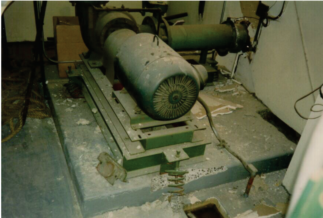
Figure 6.4.1.3-2 Failure of pump mounted on three vibration isolators and damage at wall penetration (Photo courtesy of Mason Industries).
