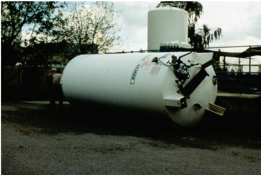
Figure 6.4.2.1-2 A vertical tank at hospital overturned due to inadequate anchorage in the 1994 Northridge Earthquake (Photo courtesy of OSHPD).
