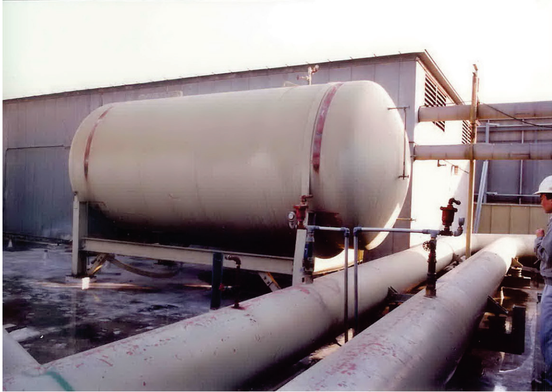
Figure 6.4.2.1-3 Horizontal tank strapped to structural support frame on hospital roof; one strap failed and tank slid six inches in the 1994 Northridge Earthquake (Photo courtesy of OSHPD).
