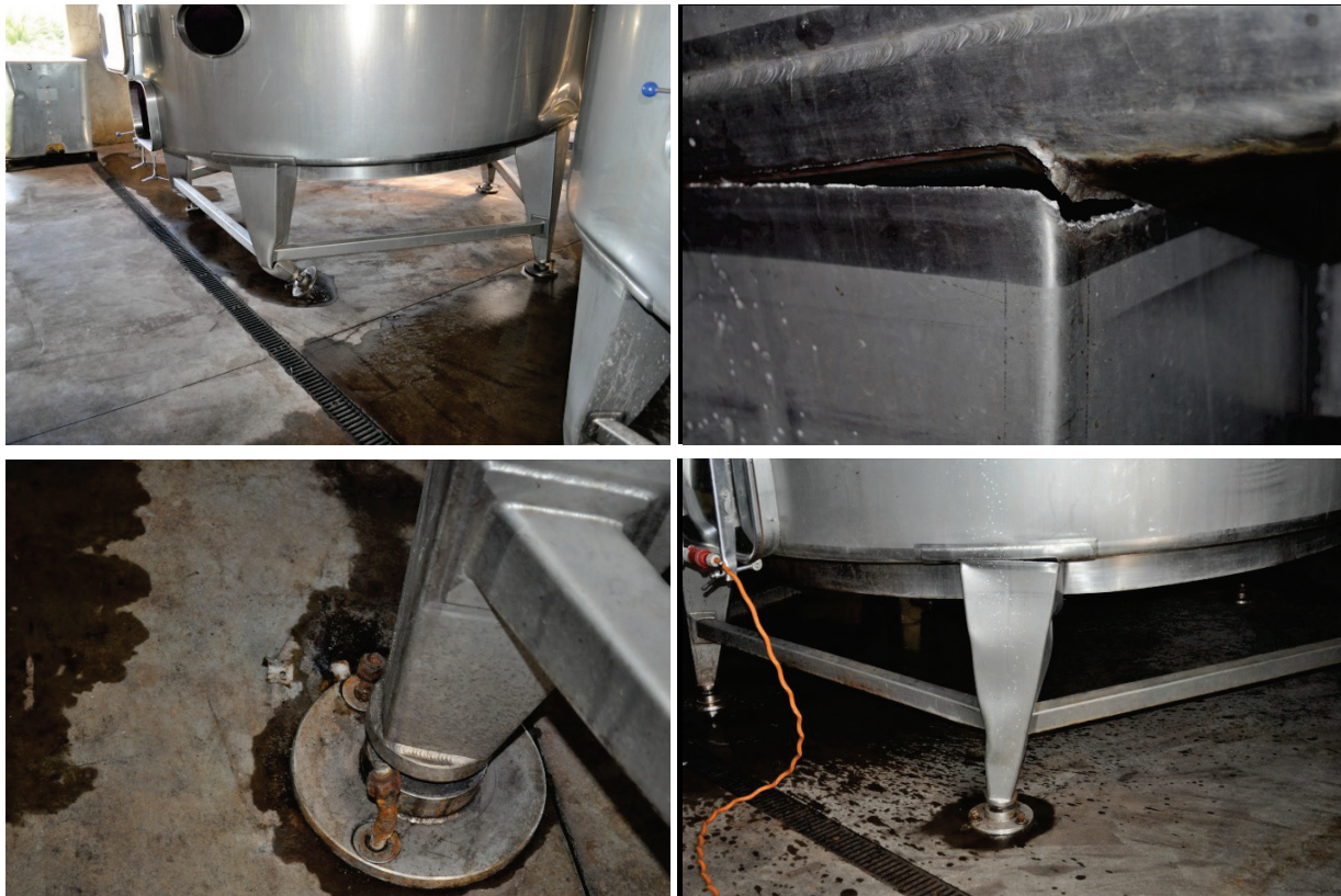
Figure 6.4.2.1-4 Wineries suffered extensive damage in the 2010 magnitude-8.8 Chile Earthquake with many barrels of wine spilled. This winery had damage to anchored tanks; tank anchorage failed, legs buckled, welds tore, anchor bolts pulled up, etc. The tank legs all have leveling bolts at the bottom, creating a weak zone between the bottom of the leg and the anchor plate. Similar unanchored tanks in this facility shifted position but were undamaged (Photos courtesy of Eduardo Fierro, BFP Engineers).
