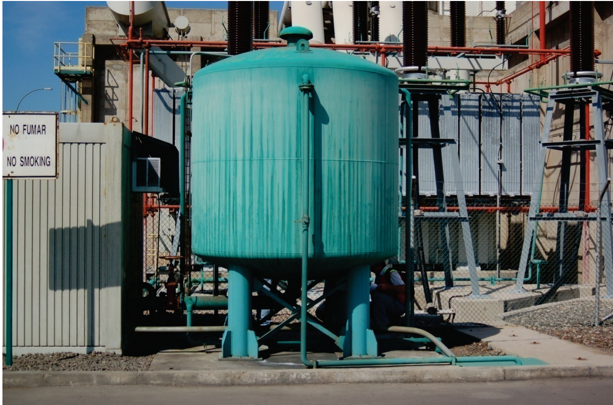
Figure 6.4.2.1-7 Gusset plates and cross bracing added at base of vertical tank on four legs following the 2001 magnitude-8.4 Peru Earthquake (Photo courtesy of Eduardo Fierro, BFP Engineers).
