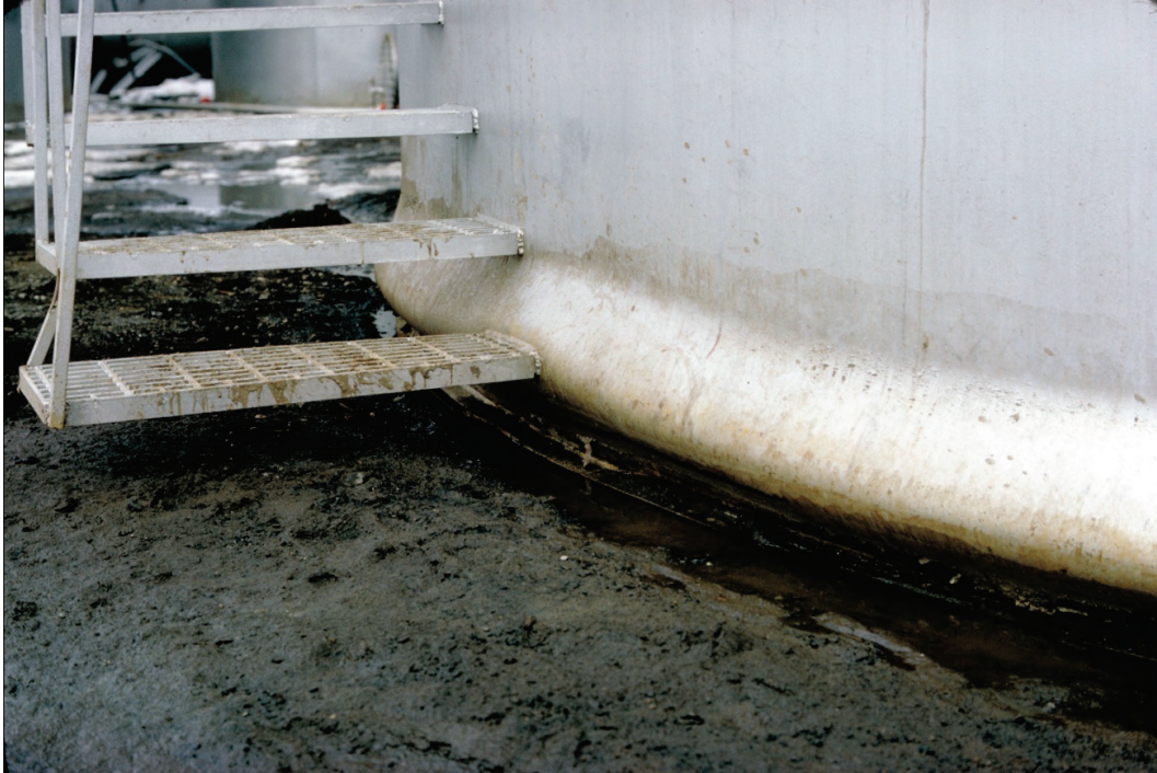
Figure 6.4.2.2-2 Tank with “elephant’s foot” buckle at the base in the 1964 magnitude-9.2 Anchorage, Alaska earthquake (Photo courtesy of PEER, Steinbrugge Collection, No. S2508)
