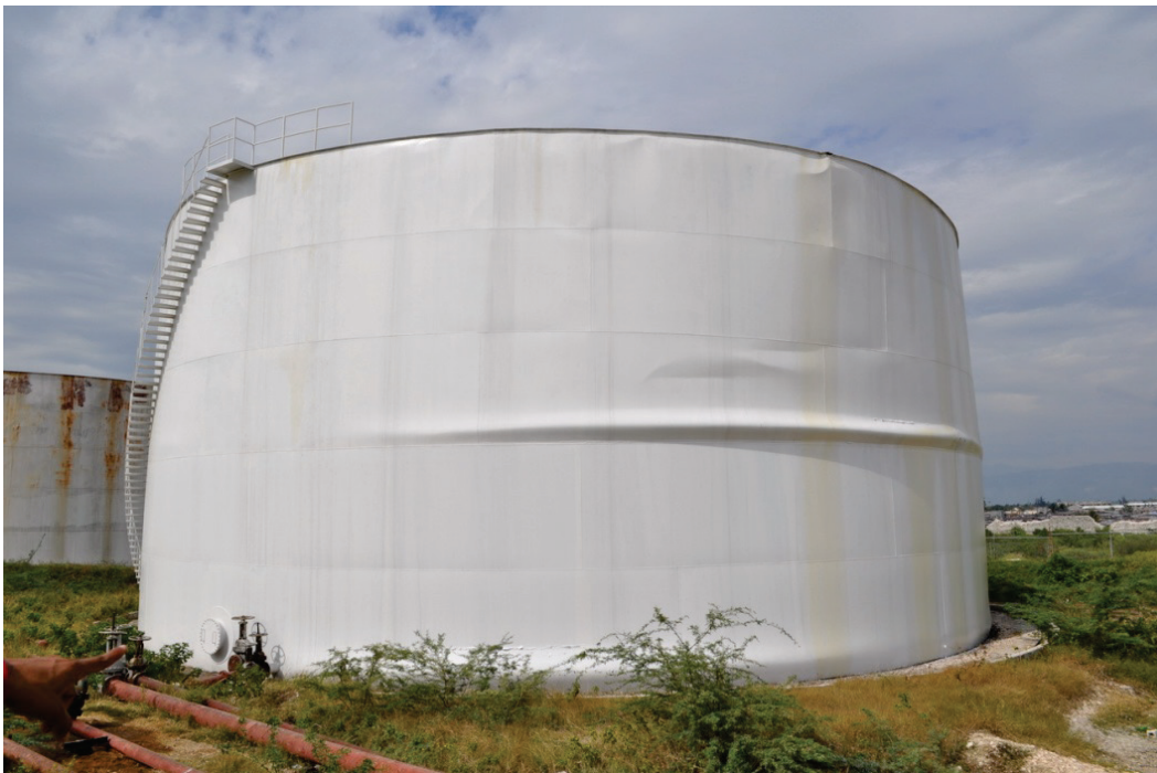
Figure 6.4.2.2-3 Tank with “elephant’s foot” and “elephant knee” in Port-au-Prince in the 2010 magnitude-7 Haiti Earthquake (Photo courtesy of Eduardo Fierro, BFP Engineers).
