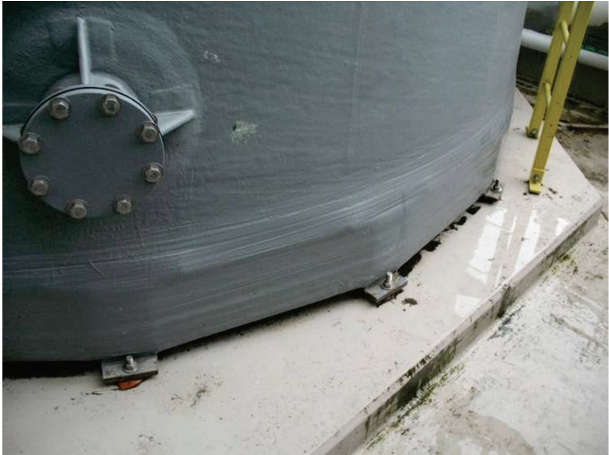
Figure 6.4.2.2-6 Anchors at base of fiberglass reinforced plastic tank (Photo courtesy of Jeffrey Soulages, Intel).
