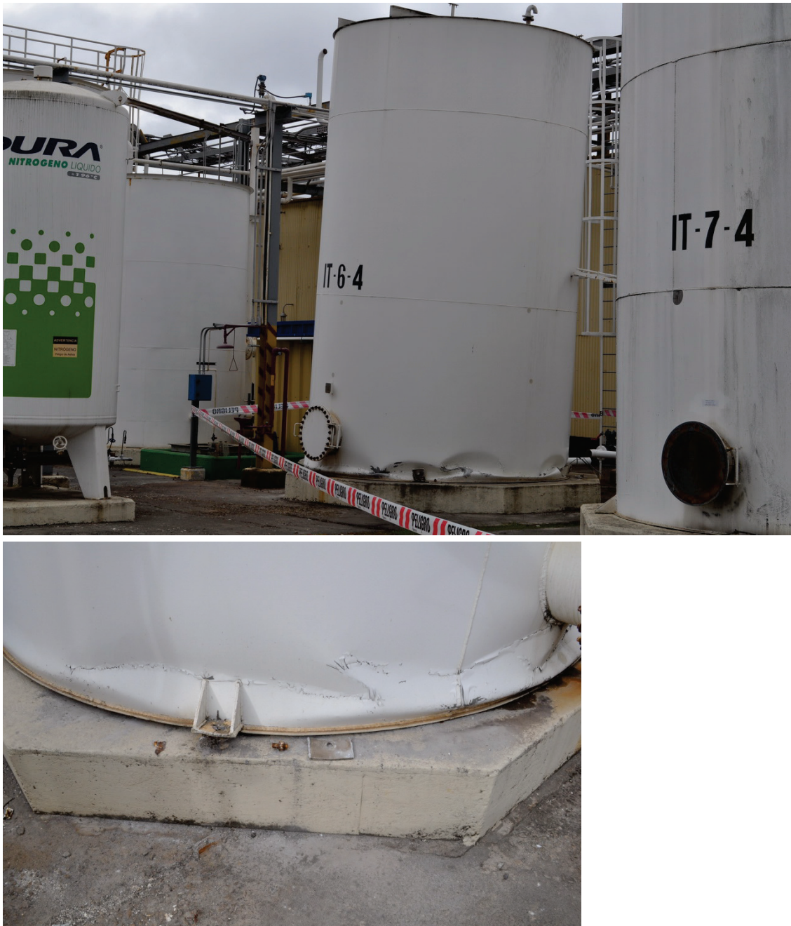
Figure 6.4.2.2-4 Anchored tank damaged at base when anchorage failed; tank slid and ruptured attached piping in 2010 magnitude-8.8 Chile Earthquake (Photo courtesy of Eduardo Fierro, BFP Engineers).
