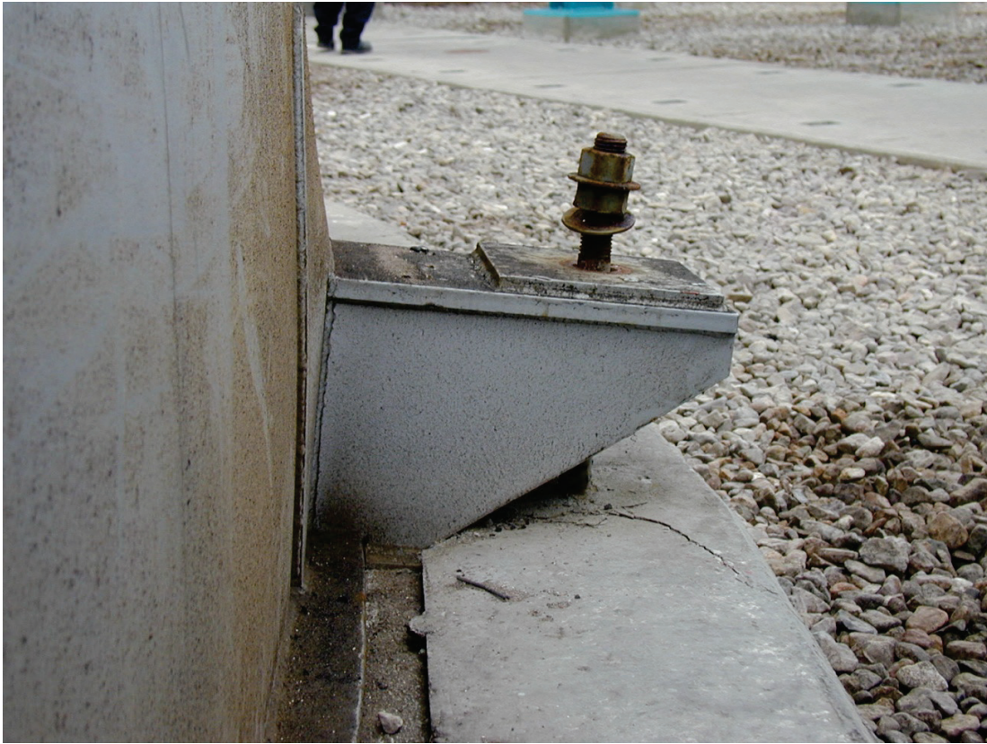
Figure 6.4.2.2-1 Damage to ductile connection at base of a 5000 cubic meter diesel fuel tank in the 2001 magnitude-8.4 Peru Earthquake. All eight connections were damaged; damage included bolt elongation, deformation of tank wall, and cracked concrete pad (Photo courtesy of Eduardo Fierro, BFP Engineers).
