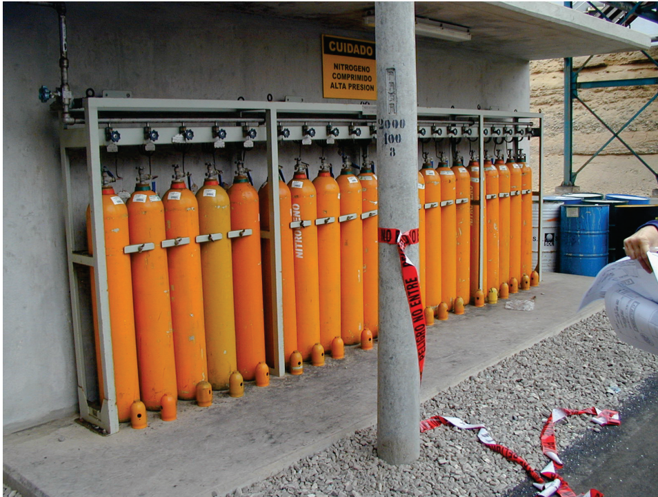
Figure 6.4.2.3-2 Gas cylinder anchorage with attached gas lines undamaged in the 2001 magnitude-8.4 Peru Earthquake (Photo courtesy of Eduardo Fierro, BFP Engineers).
