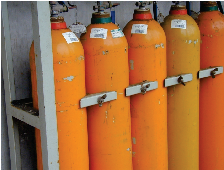
Figure 6.4.2.3-3 Detail of undamaged gas cylinder installation (Photo courtesy of Eduardo Fierro, BFP Engineers).
