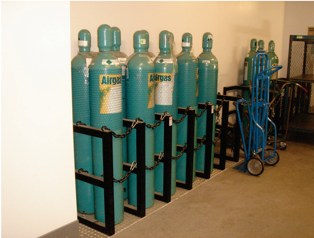
Figure 6.4.2.3-7 Detail of enclosures for airgas tanks in a hospital; chains attached with quick release hooks (Photo courtesy of Maryann Phipps, Estructure).
