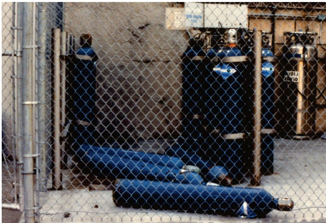
Figure 6.4.2.3-1 Unanchored tanks inside fenced enclosure in the 1994 magnitude-6.7 Northridge Earthquake (Photo courtesy of OSHPD).
