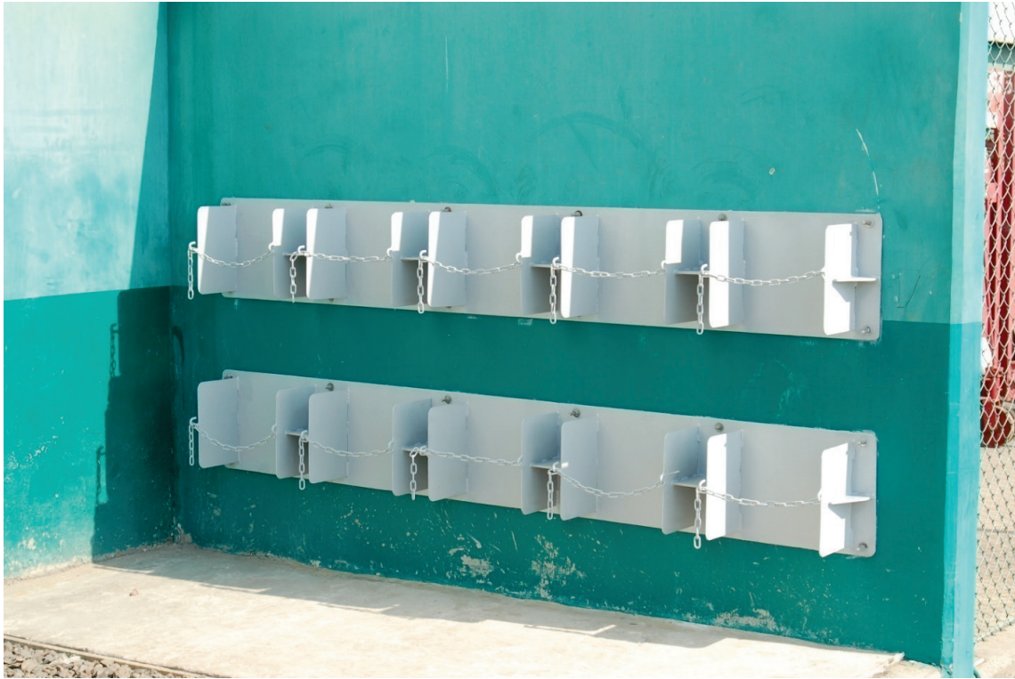
Figure 6.4.2.3-4 Wall-mounted cylinder restraints upgraded with stiffener plates following the 2001 Peru Earthquake (Photo courtesy of Eduardo Fierro, BFP Engineers).
