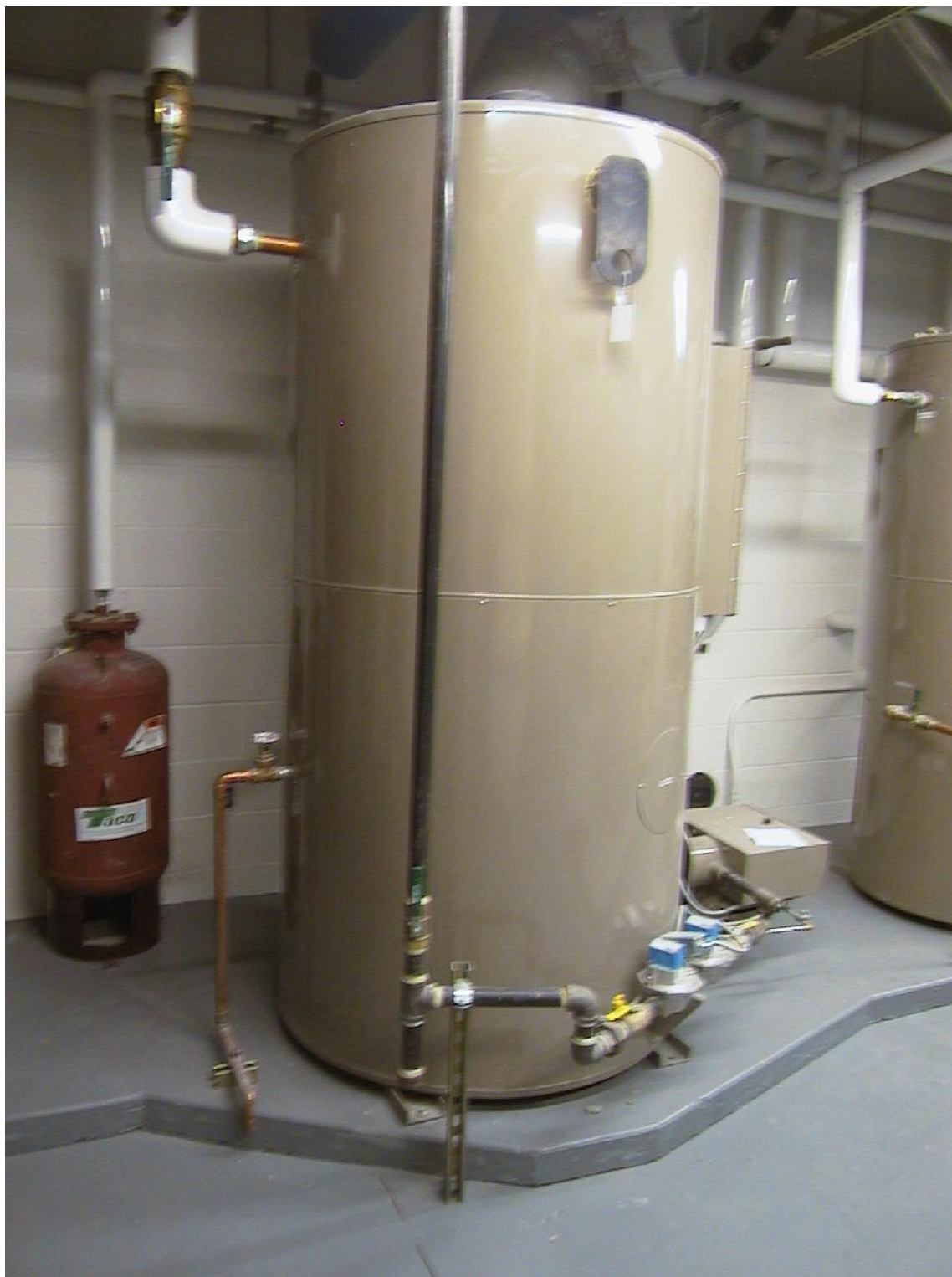
Figure 6.4.2.4-5 Base-mounted water heater located in a school; equipment supplied with metal base for mounting (Photo courtesy of EQE for the Salt Lake City School District).
