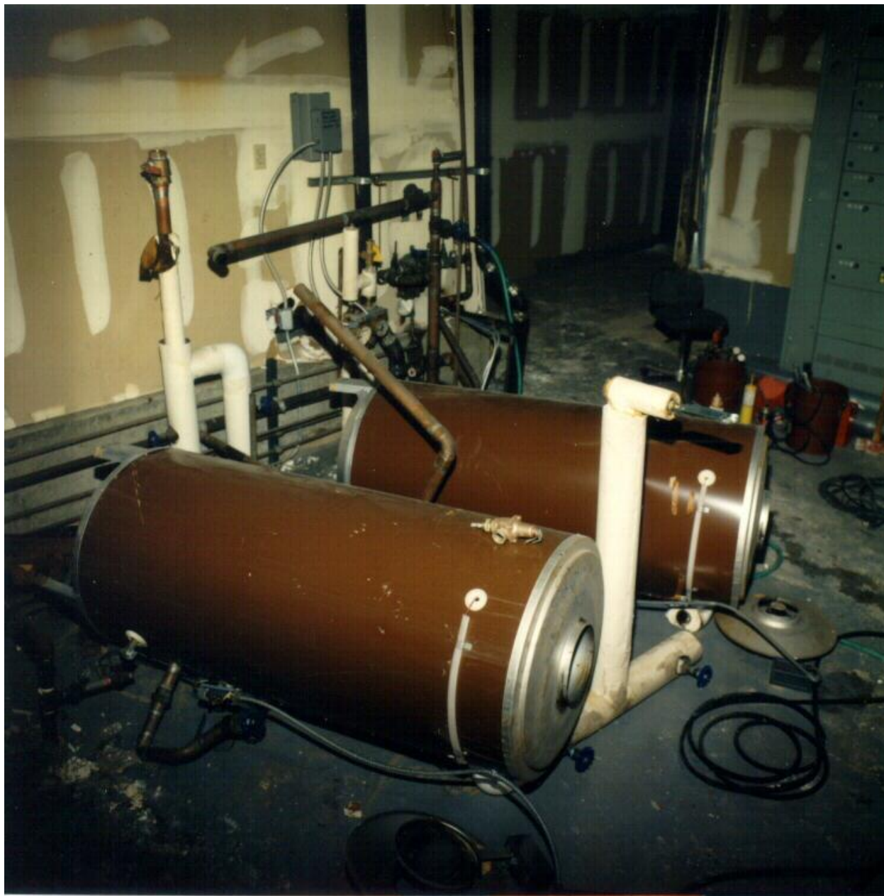
Figure 6.4.2.4-1 Unanchored water heaters overturned (Photo courtesy of Mason Industries).
