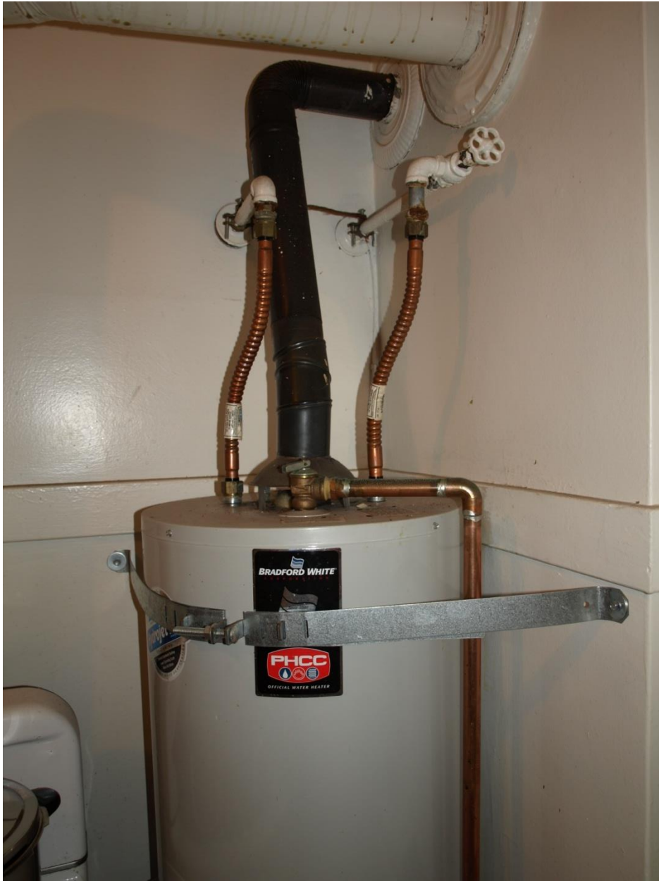
Figure 6.4.2.4-4 Corner installation using a commercially available strap; note flex copper tubing for water hook up (Photo courtesy of Cynthia Perry, BFP Engineers).
