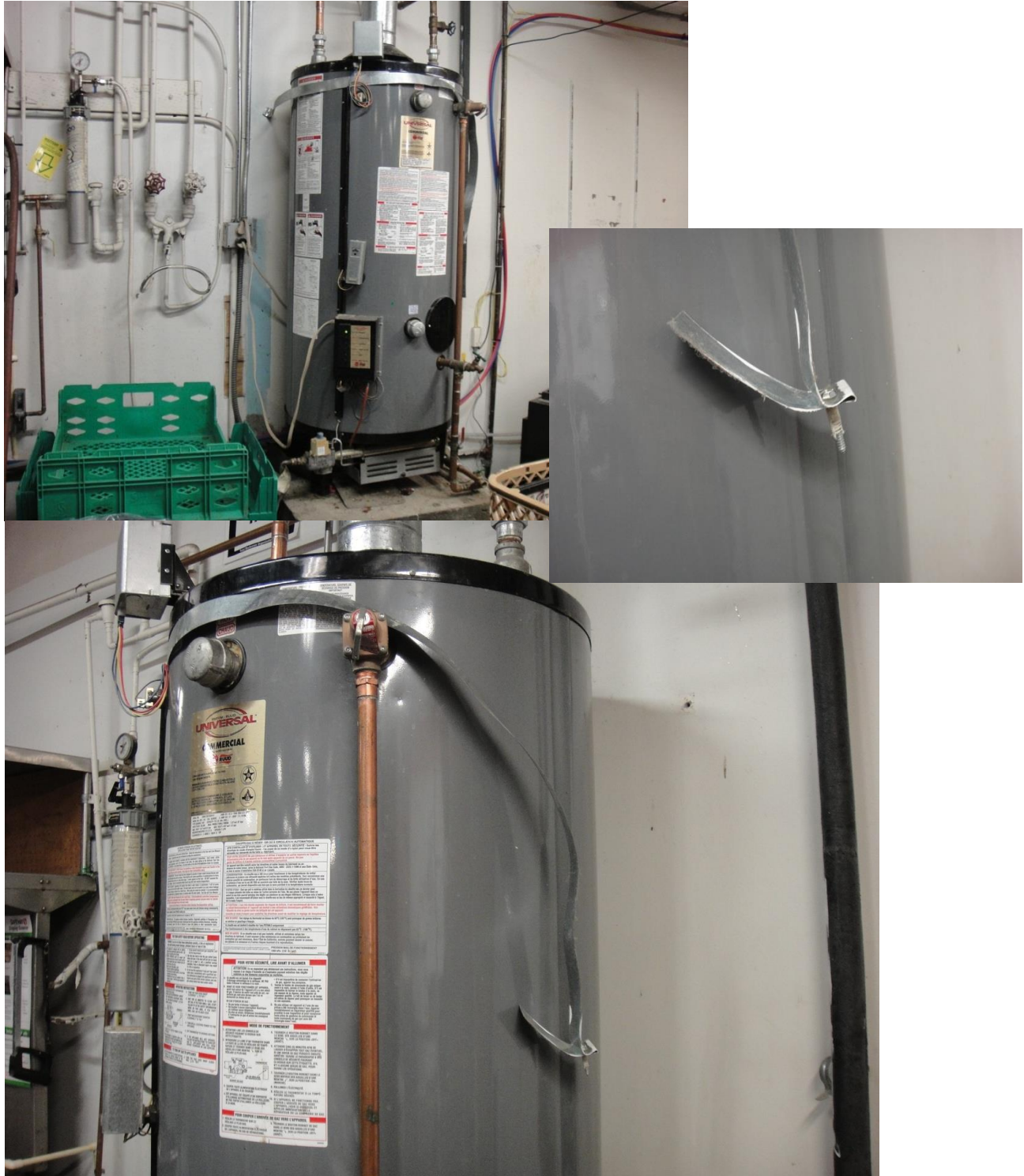
Figure 6.4.2.4-3 Damaged water heater in the 2010 magnitude-6.5 Eureka Earthquake. The water heater strap pulled out from the supporting concrete wall as a result of inadequate anchorage. The tank moved sufficiently to break interconnected water lines which were rigidly connected to the tank.
