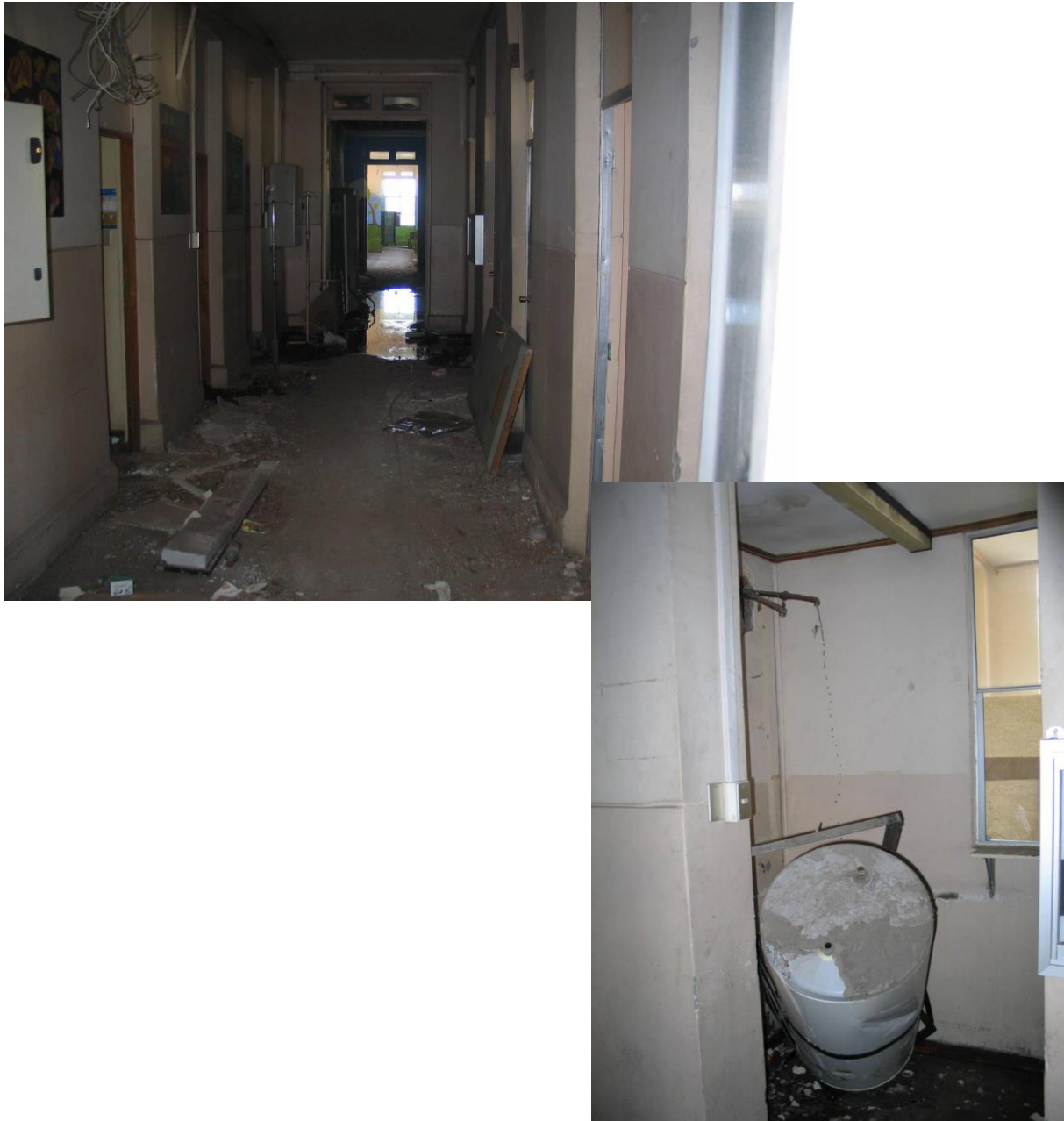
Figure 6.4.2.4-2 Water damage at the Talca Hospital in the 2010 magnitude-8.8 Chile Earthquake; water leaking from tank at right. This building was closed due to nonstructural damage, dominated by water damage (Photos courtesy of Bill Holmes, Rutherford & Chekene).
