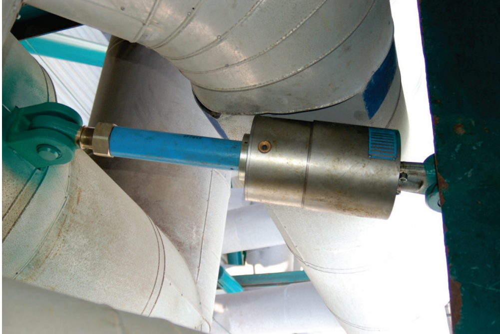
Figure 6.4.3.1-8 Viscous damper used as restraint on large insulated pipe (Photo courtesy of Eduardo Fierro, BFP Engineers).
