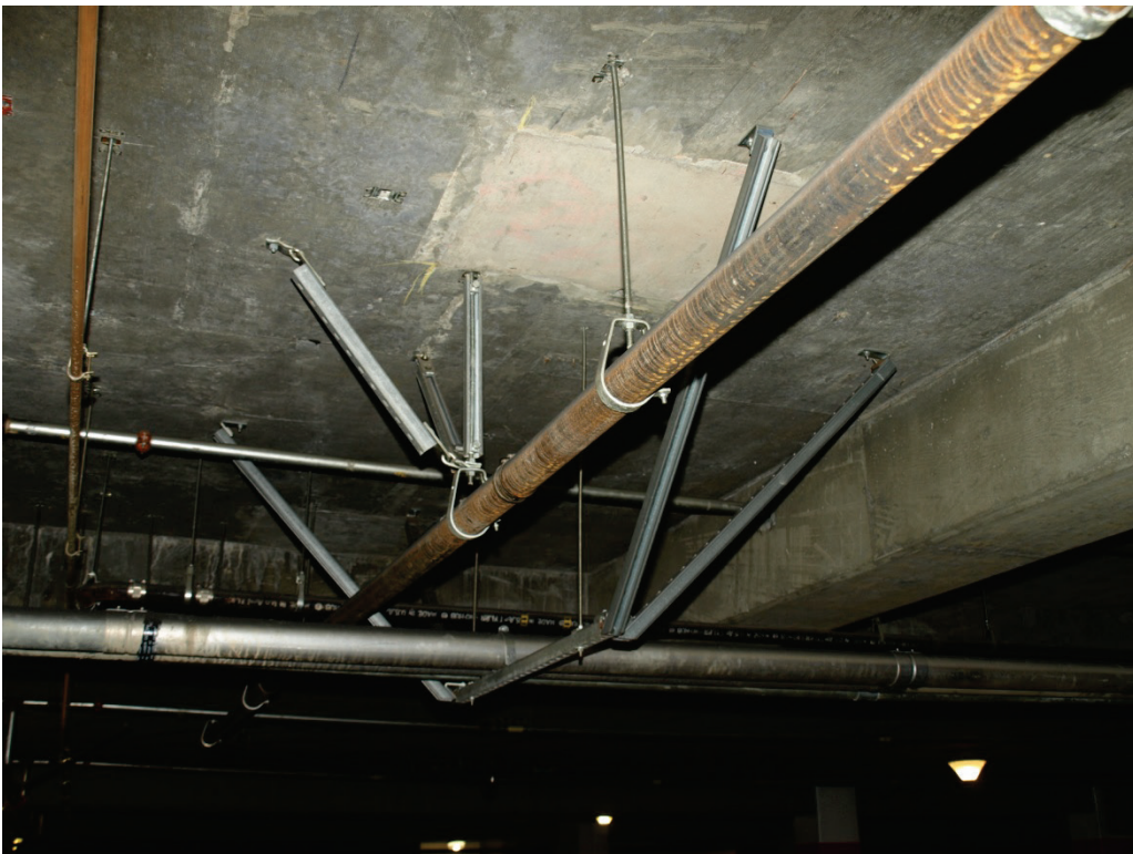
Figure 6.4.3.1-7 Transverse bracing with J-hanger and strut at the restraining bolt. Note that longitudinal brace shown is ineffective because the J-hanger can slip along the length of the pipe; a pipe clamp or equivalent is required for a longitudinal brace (Photo courtesy of Cynthia Perry, BFP Engineers).
