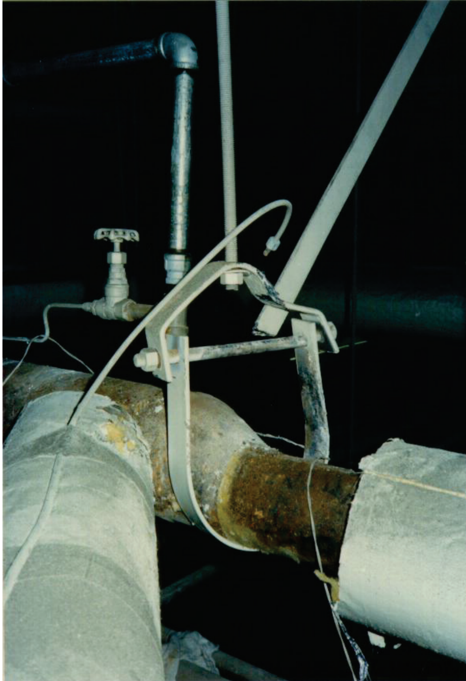
Figure 6.4.3.1-3 Pipe brace failed at connection in 1994 Northridge Earthquake; insulation removed prior to photo (Photo courtesy of Mason Industries).
