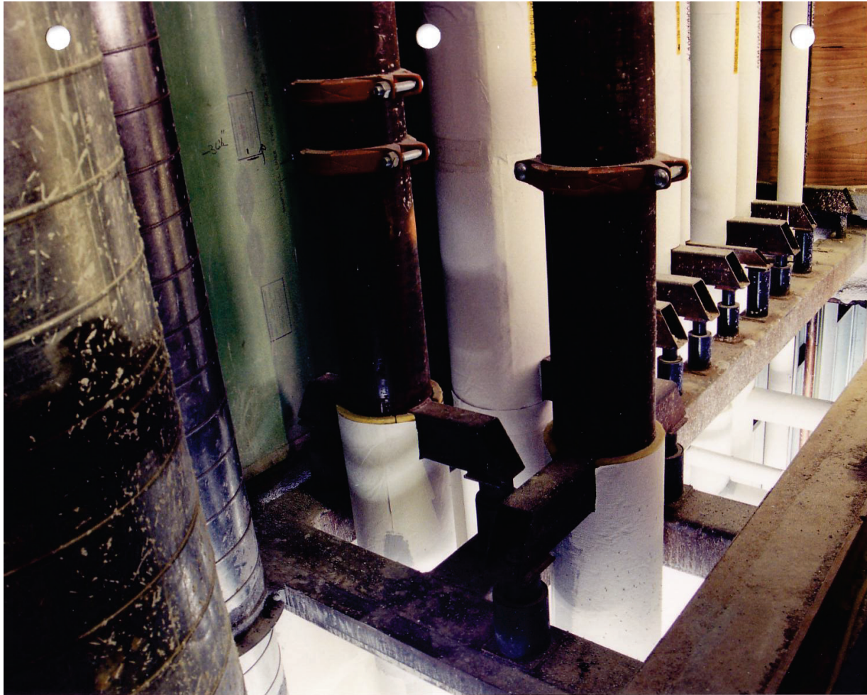
Figure 6.4.3.4-2 Riser supports provide lateral restraint with vertical sliding guides that allow thermal movement; restraint hardware consisting of tube sections is welded to either side of pipe (Photo courtesy of Mason Industries).
