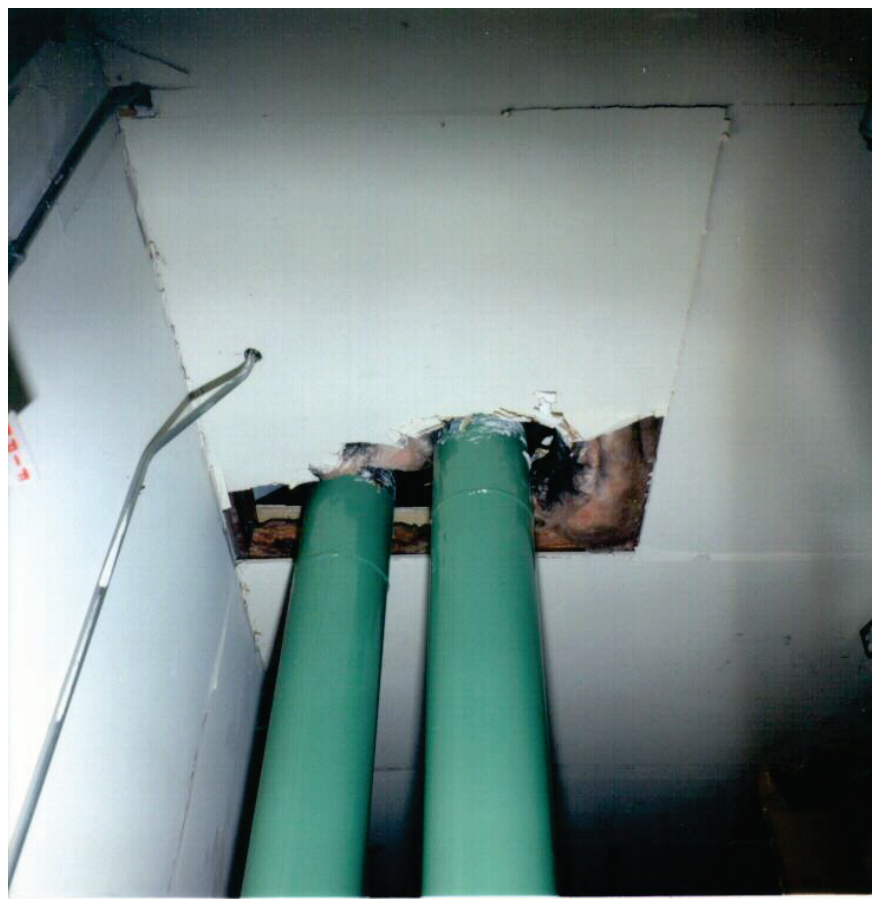
Figure 6.4.3.4-1 Movement of unbraced risers damaged ceiling finishes and insulation in the 1994 magnitude-6.7 Northridge Earthquake (Photo courtesy of Mason Industries).
