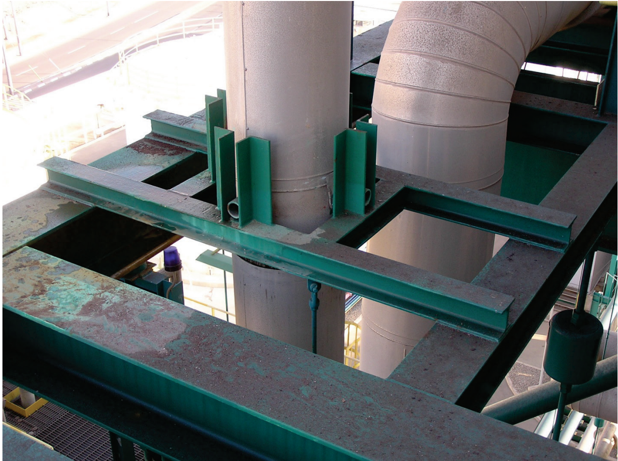
Figure 6.4.3.4-4 Insulated boiler pipe risers with welded lugs (small pipe sections) which travel vertically in guides providing lateral seismic restraint (Photo courtesy of Eduardo Fierro, BFP Engineers).
