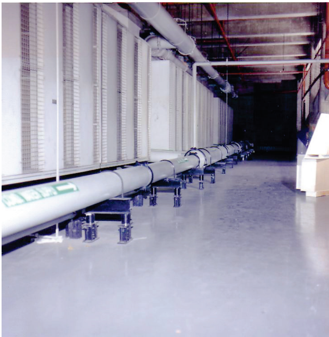
Figure 6.4.3.5-3 Floor-mounted supports for insulated pipe with vibration isolation (Photo courtesy of Mason Industries).
