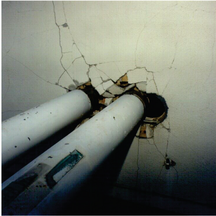
Figure 6.4.3.5-2 Damage to piping, stud wall and finishes due to movement of poorly restrained floor-mounted piping in the 1994 magnitude-6.7 Northridge Earthquake (Photo courtesy of Mason Industries).
