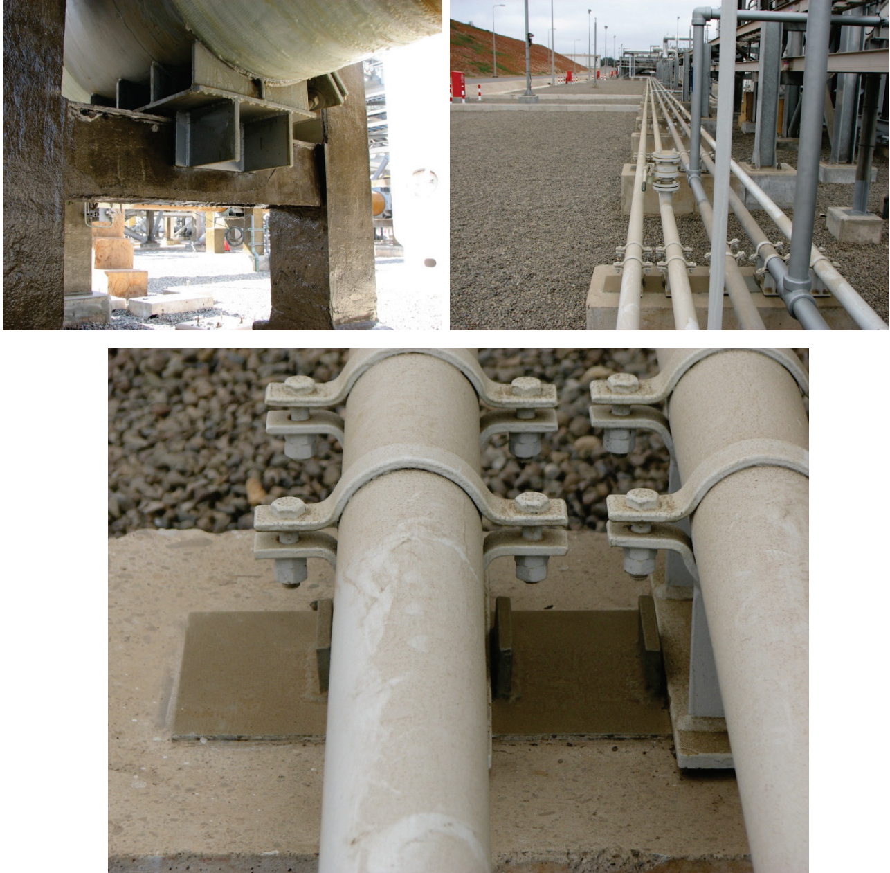
Figure 6.4.3.5-5 Floor-mounted supports for industrial piping in Chile; piping undamaged in the 2010 Chile Earthquake. The Chilean Industrial Code (Norma Chilena 2369) requires that shear forces be resisted by shear keys as shown; lower photo is detail of piping at upper right (Photos courtesy of Antonio Iruetagoiena, Rubén Boroschek & Associates).
