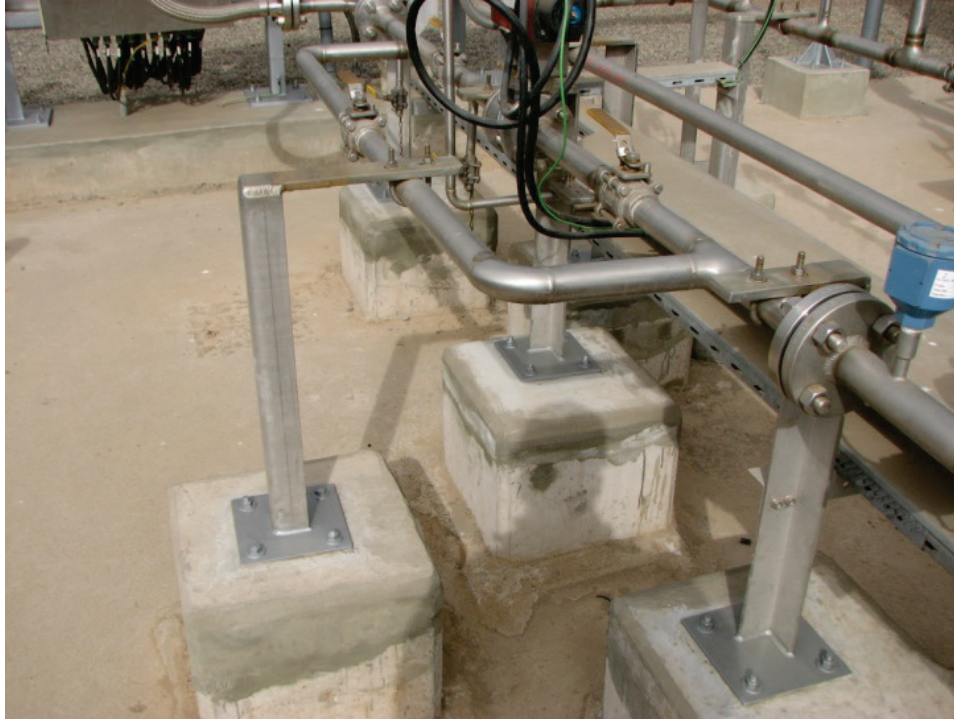
Figure 6.4.3.5-4 Floor/ground-mounted supports for industrial piping in Chile; piping undamaged in the 2010 magnitude-8.8 Chile Earthquake. Pipe supports include concrete pedestal, base plate, and built-up welded support stand. (Photos courtesy of Antonio Iruretagoyena, Rubén Boroschek & Associates).
