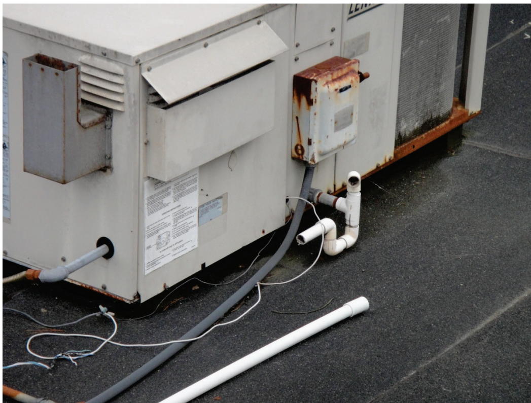
Figure 6.4.3.6-3 Unrestrained roof-mounted piping broke at the connection to the equipment in the 2010 Eureka Earthquake. Piping mounted on wood sleepers should typically be restrained to the roof, not free to slide (Photo courtesy of Maryann Phipps, Estructure).
