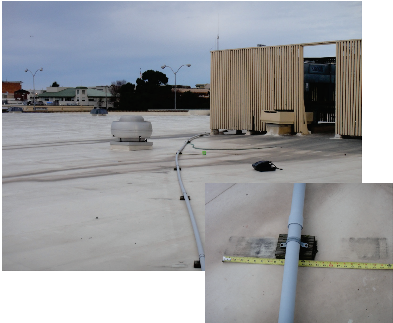
Figure 6.4.3.6-2 Unrestrained wood sleepers on roof-mounted piping slid a foot in either direction in 2010 magnitude-6.5 Eureka Earthquake (Photos courtesy of Maryann Phipps, Estructure).
