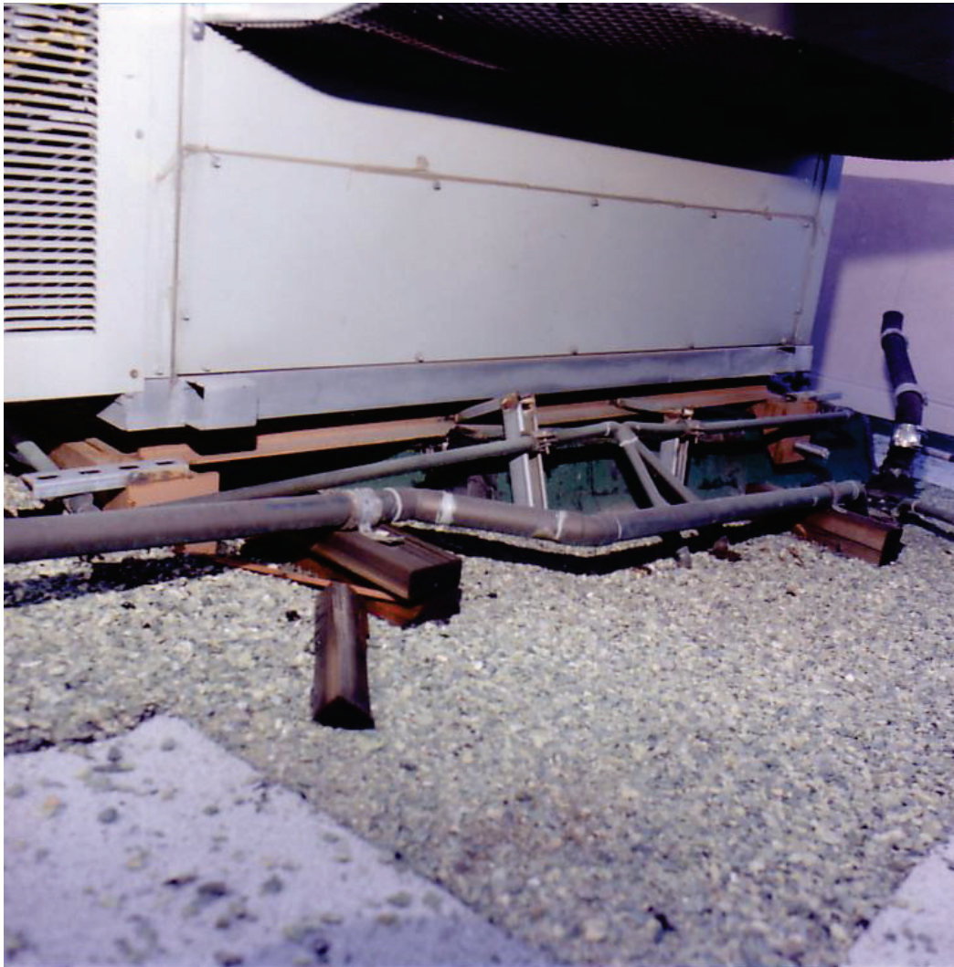
Figure 6.4.3.6-1 Damaged supports and piping on roof-mounted HVAC unit in the 1994 magnitude-6.7 Northridge Earthquake (Photo courtesy of Mason Industries). Both the roof-mounted wood sleepers and strut supports failed.
