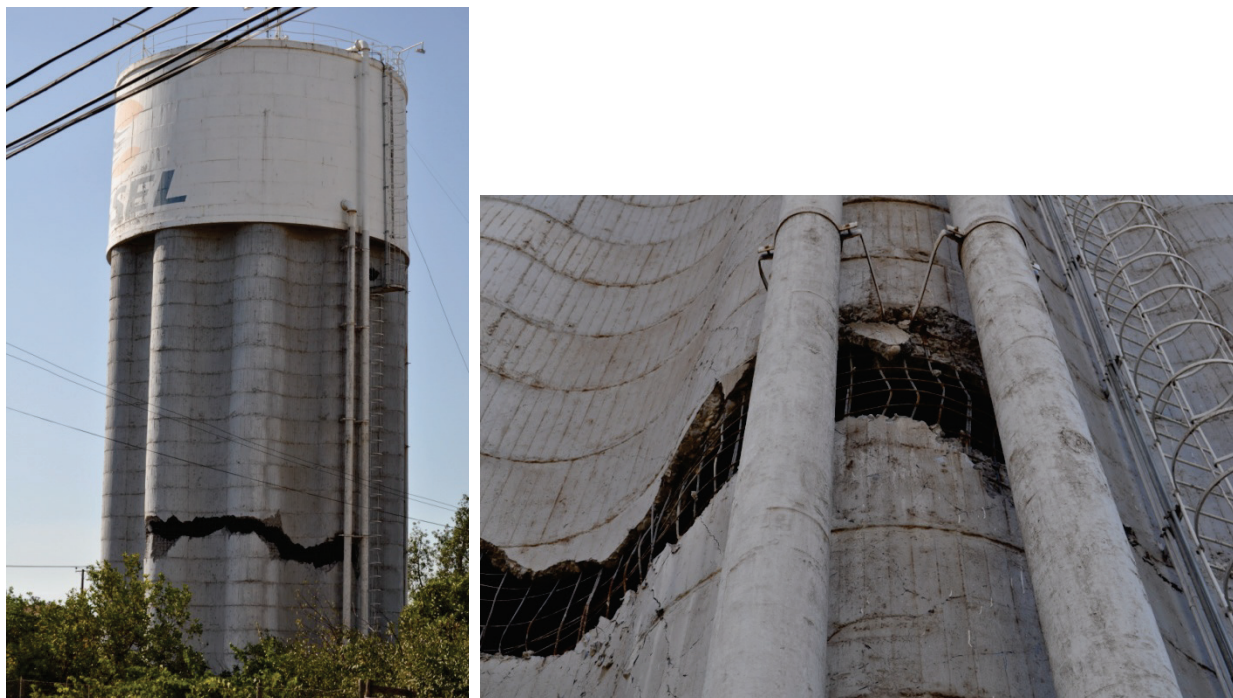
Figure 6.4.3.7-2 Pipe supports attached to wall of damaged silo (Photo courtesy of Eduardo Fierro, BFP Engineers). In spite of structural damage to silo, cast-in-place pipe supports were still intact and the piping did not fall.
