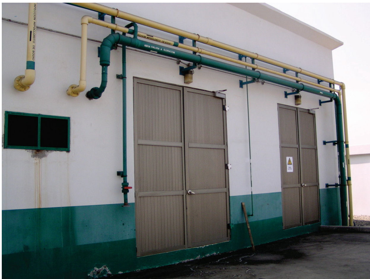
Figure 6.4.3.7-1 Wall-mounted supports for horizontal and vertical pipe runs with exterior exposure. Photo shows minor damage at wall penetration of green pipe and minor movement at some U-bolts, but restraints generally performed well (Photo courtesy of Eduardo Fierro, BFP Engineers). Note that lateral restraint near an elbow can be used to provide longitudinal restraint for a perpendicular pipe run.
