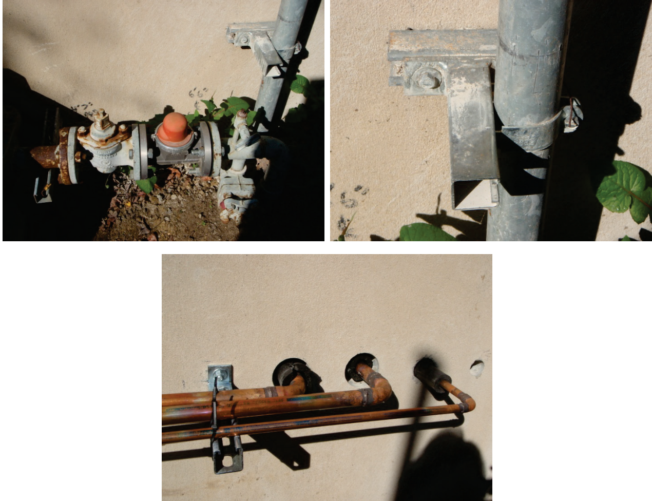
Figure 6.4.3.7-3 Wall-mounted pipe restraint examples using standard strut shapes and connectors (Photo courtesy of Cynthia Perry, BFP Engineers). Bottom view still under construction; pipes temporarily attached with plastic ties.
