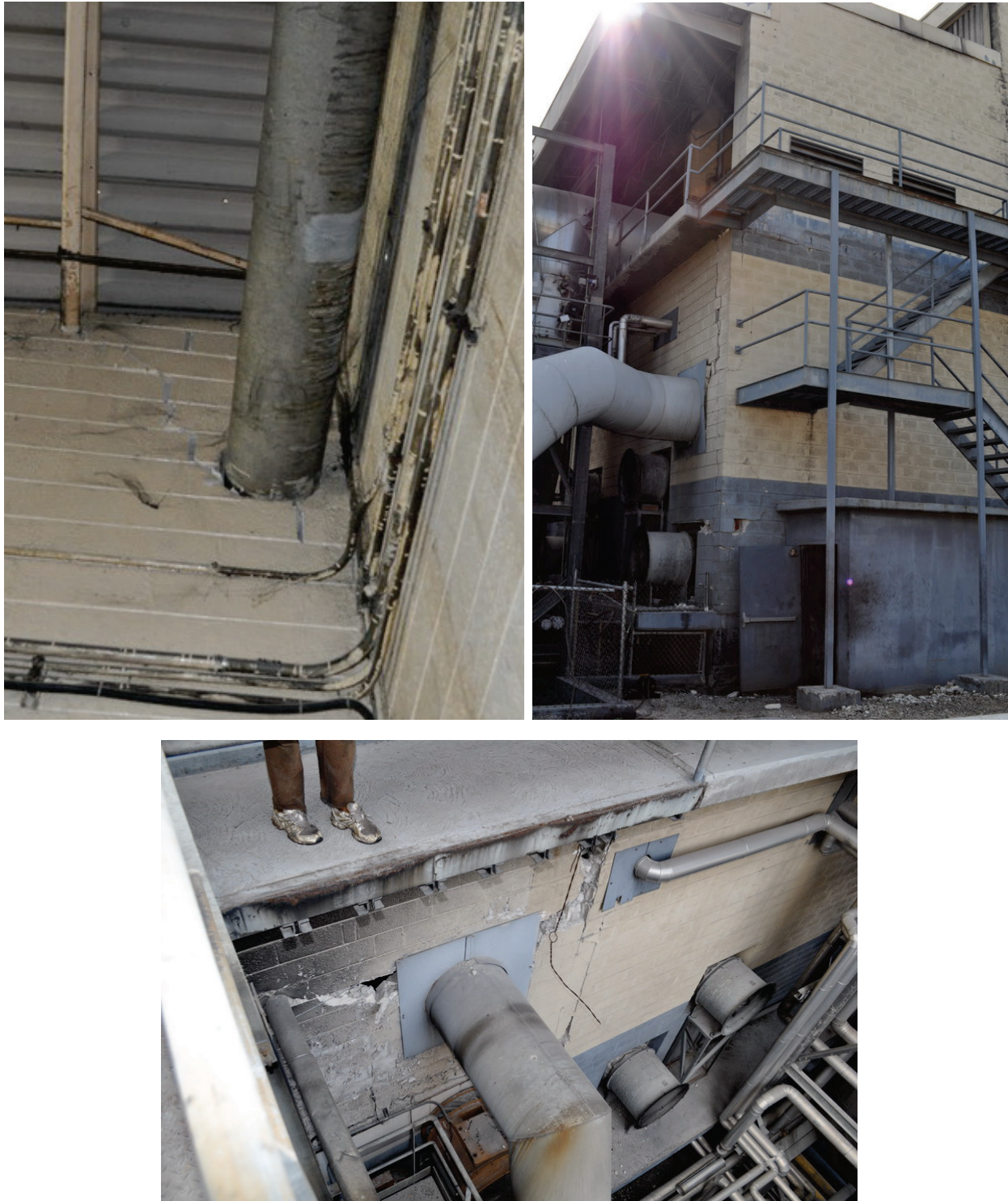
Figure 6.4.3.8-3 Wall penetrations for piping and ducts contributed to damage to unreinforced masonry walls at an industrial facility in the 2010 magnitude-7 Haiti Earthquake (Photos courtesy of Eduardo Fierro, BFP Engineers). The piping and ducts were not damaged but the walls cracked and will need to be repaired.
