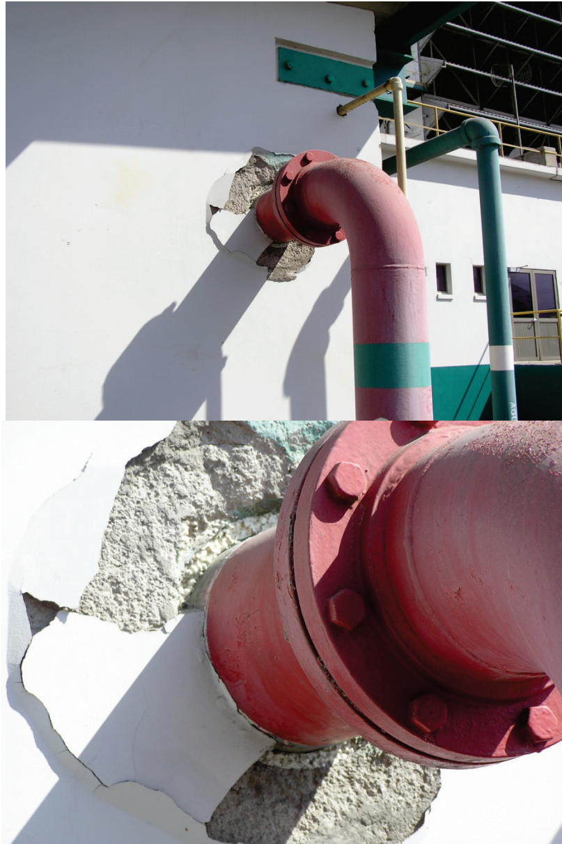
Figure 6.4.3.8-2 Exterior stucco damage at wall penetration for fire protection piping in the 2001 magnitude-8.4 Peru Earthquake (Photos courtesy of Eduardo Fierro, : BFP Engineers).
