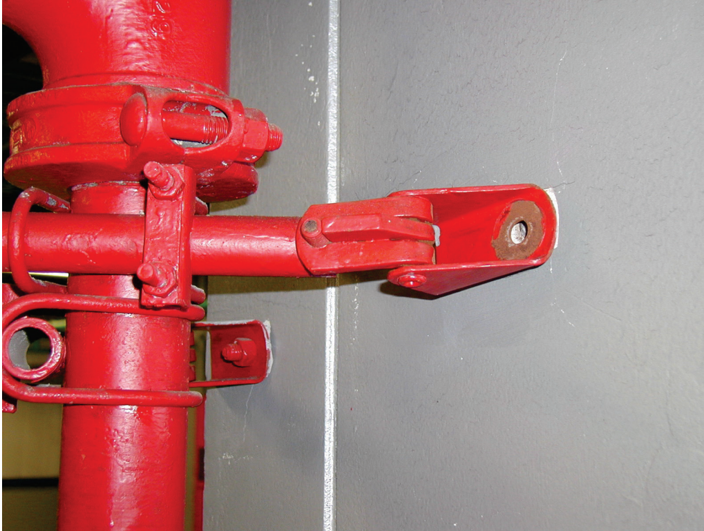
Figure 6.4.4.1-2 Wall-mounted pipe restraint failed due to inadequate connection to structural framing in the 2001 magnitude-8.4 Peru Earthquake (Photo courtesy of Eduardo Fierro, BFP Engineers).
