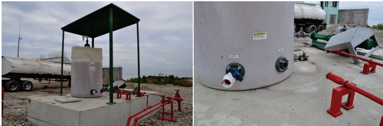
Figure 6.4.4.1-5 Unanchored holding tank slid on concrete pad, breaking fire protection piping and disabling the fire protection system in the 2010 Haiti Earthquake. In this case, the piping was well anchored but the tank was unrestrained (Photo courtesy of Eduardo Fierro, BFP Engineers).
