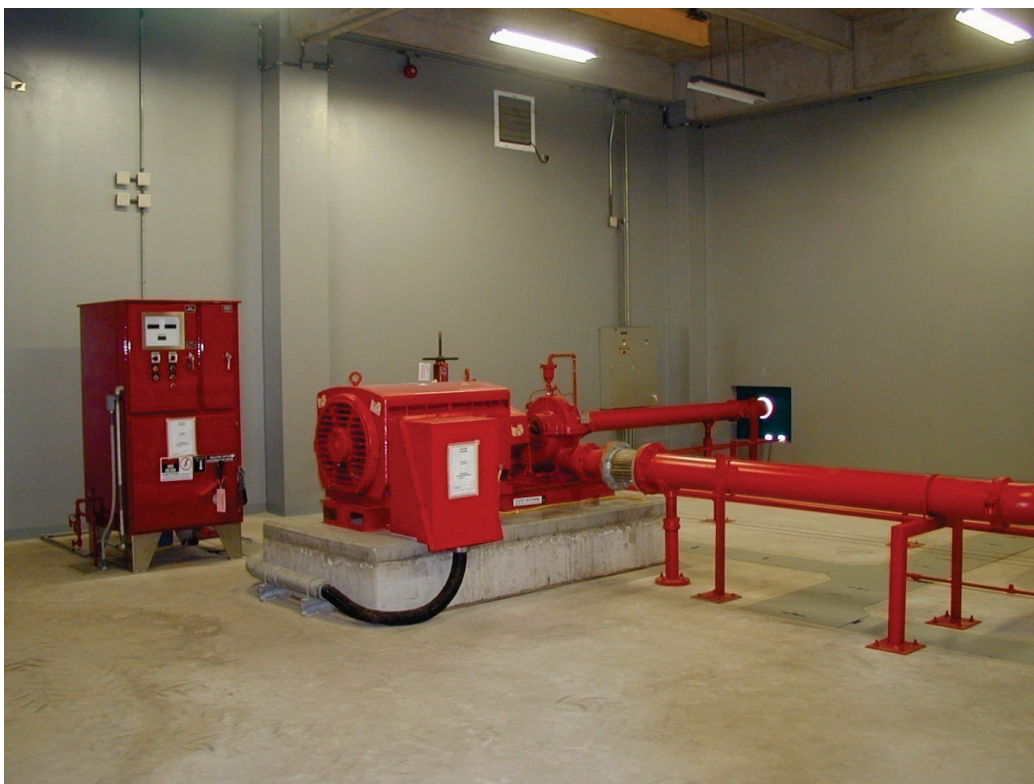
Figure 6.4.4.1-8 There was no damage to the fire suppression equipment in this control room in the 2001 Peru Earthquake because the pump and the control panel were well anchored and the piping had flexible connections with adequate sized wall penetration and no overhead falling hazards (Photo courtesy of Eduardo Fierro, BFP Engineers).
