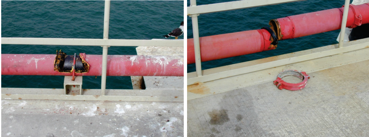
Figure 6.4.4.1-6 Damage to industrial fire protection piping located on jetty in 2001 Peru Earthquake. Longitudinal slip at U-bolt shown at left; this U-bolt still intact but other U-bolts broke and fell off the jetty. Failure of joint coupling and crushing of pipe shown at right (Photo courtesy Eduardo Fierro, BFP Engineers).
