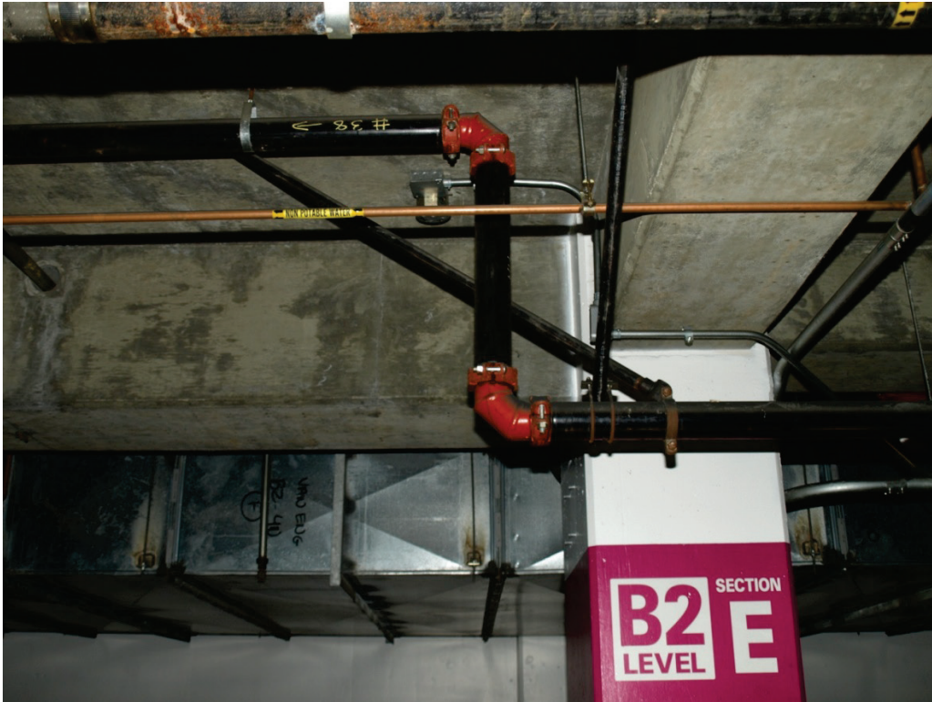
Figure 6.4.4.1-9 Transverse and longitudinal restraints on fire protection distribution line (Photo courtesy of Cynthia Perry, BFP Engineers).
