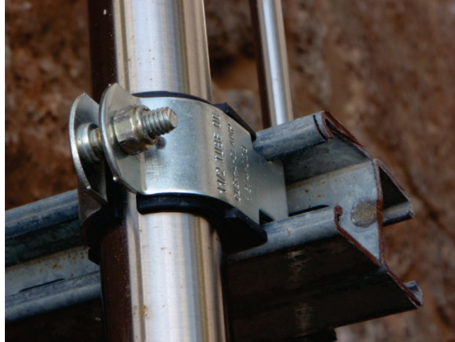
Figure 6.4.5.1-7 Process nitrogen piping outside engineering building on the UC Berkeley campus; strut clamp has rubber fittings to protect the stainless steel piping (Photos courtesy of Cynthia Perry, BFP Engineers).
