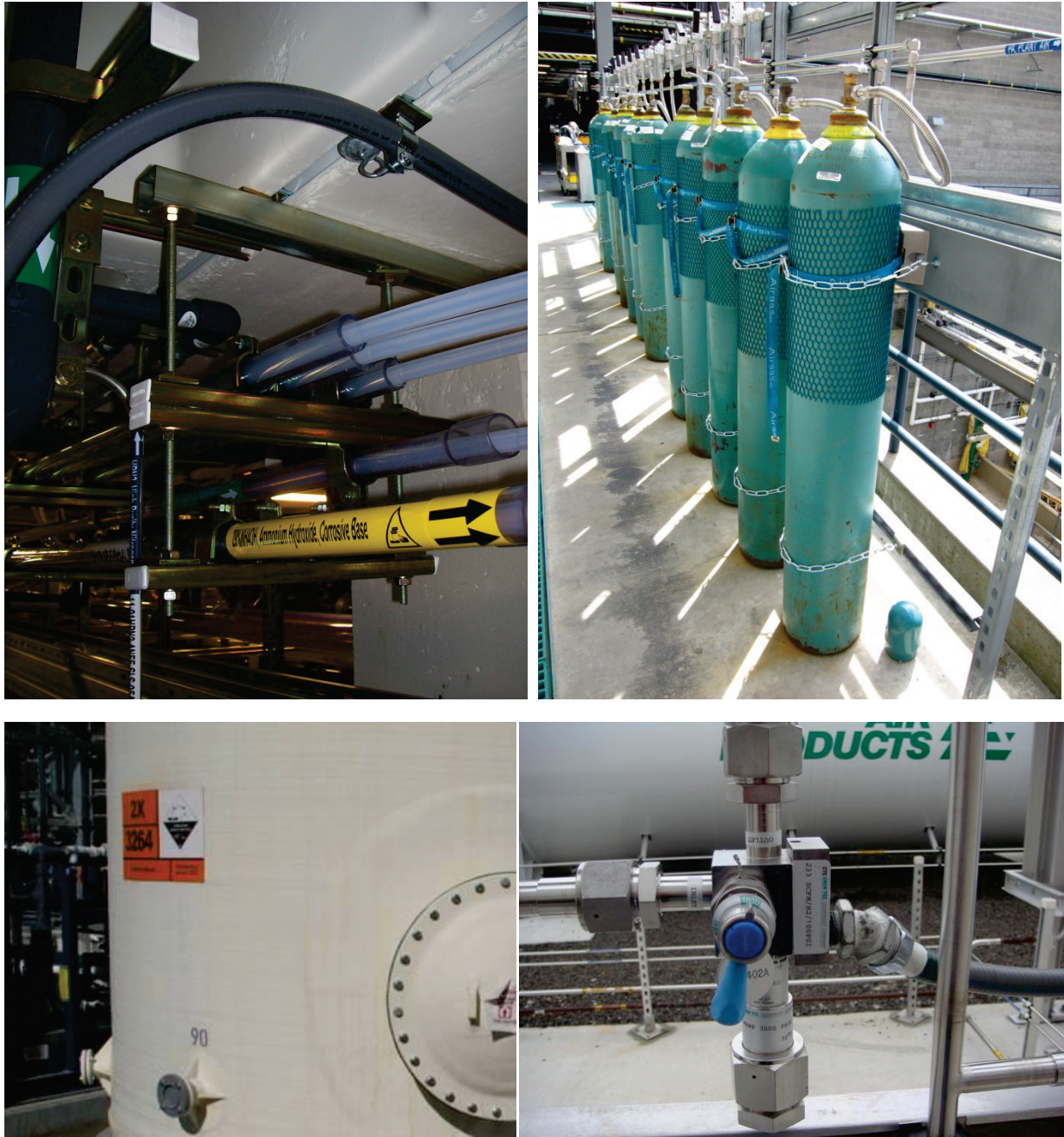
Figure 6.4.5.1-6 Clockwise from top: a) Sleeved pipe connections where seismic anchorage consists of cushioned pipe clamp attached around outer sleeve and inner pipe not restrained longitudinally. b) Airgas canisters chained and strapped to supports, fitted with flexible hose, stainless steel piping (note blue label), and a row of valves. c) Label on tank shows example of European ADR danger labeling scheme. d) Excess flow valve for large gas tank (Photos courtesy of Jeffrey Soulages, Intel Corporation).
