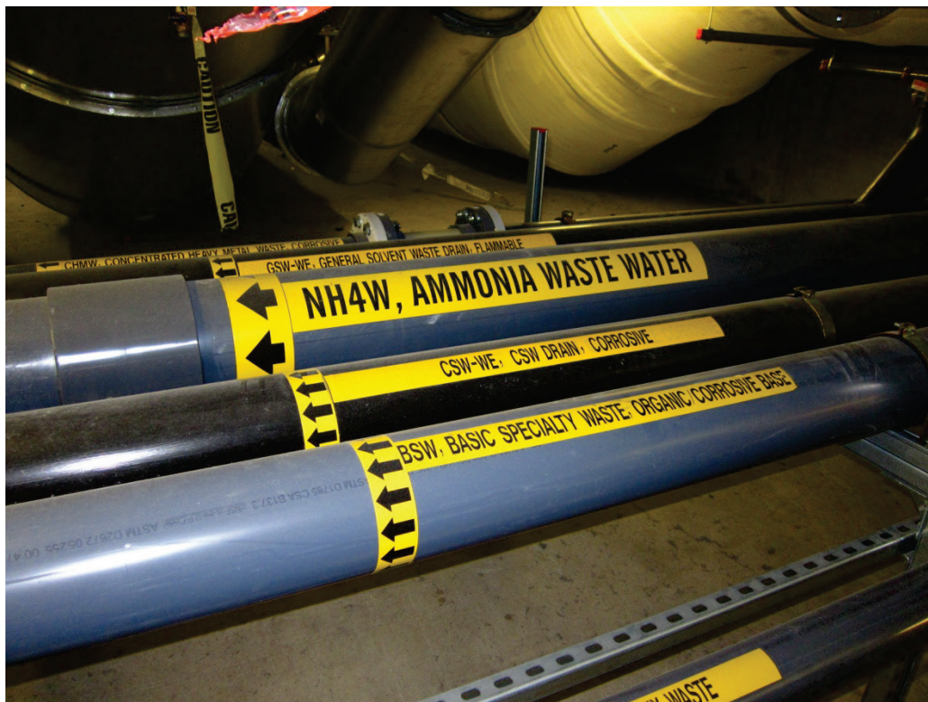
Figure 6.4.5.1-5 Two examples of double walled piping used for secondary containment of hazardous fluids. Preassembled double walled pipe with centering devices or spacers separating the inner and outer pipe is available commercially, but as shown here, the outer pipe was installed and leak tested prior to pulling the inner pipe through. Note the yellow color coded labels indicate reactive materials; flow direction also marked prominently (Photos courtesy of Jeffrey Soulages, Intel Corporation).
