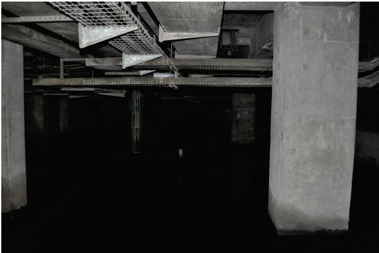
Figure 6.4.5.1-2 Basement level at power plant in Port-au-Prince flooded with oil and water in the 2010 magnitude-7 Haiti Earthquake creating hazardous conditions for inspection and clean-up (Photos courtesy of Eduardo Fierro, BFP Engineers).
