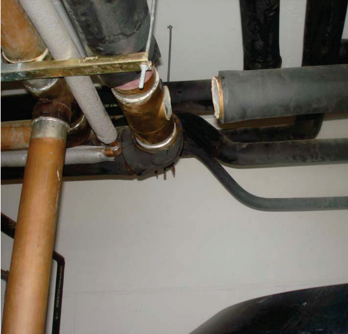
Figure 6.4.5.2-2 Broken copper piping for hot water supply in residential building in the 2010 Chile Earthquake. Trapeze shown not laterally braced but hangers appear to be less than 12" in length and may not have required lateral restraints per ASCE 7-10 (Photo courtesy of Gokhan Pekcan).
