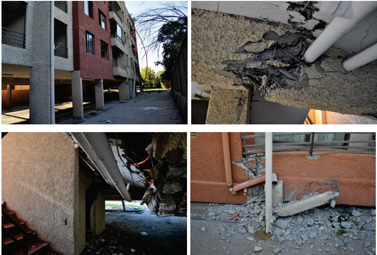
Figure 6.4.5.2-3 Photos displaying resilience of piping systems; this building suffered a partial structural collapse along one side in the 2010 Chile Earthquake. The only broken pipe (shown at lower right) was along the collapsed side; the other piping had broken pipe supports in some locations but the joints remained largely intact, even with these very large deformations (Photos courtesy of Eduardo Fierro, BFP Engineers).
