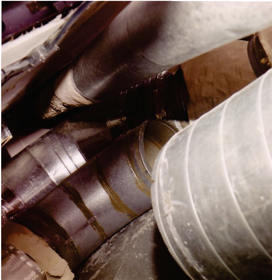
Figure 6.4.6.1-1 Unbraced ducts separated at bend in the 1994 magnitude-6.7 Northridge Earthquake (Photo courtesy of Mason Industries).
