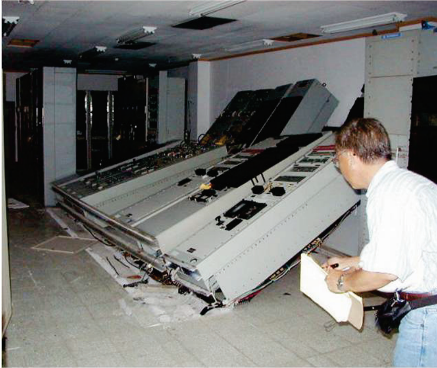
Figure 6.4.7.1-1 Overturned equipment in the 1985 magnitude-8 Mexico Earthquake, note absence of anchorage of equipment base to floor (Photo courtesy of Degenkolb Engineers).
