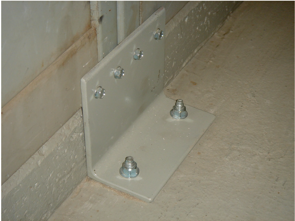
Figure 6.4.7.1-10 Detail of cabinet base anchorage (Photo courtesy of Maryann Phipps, Estructure).
