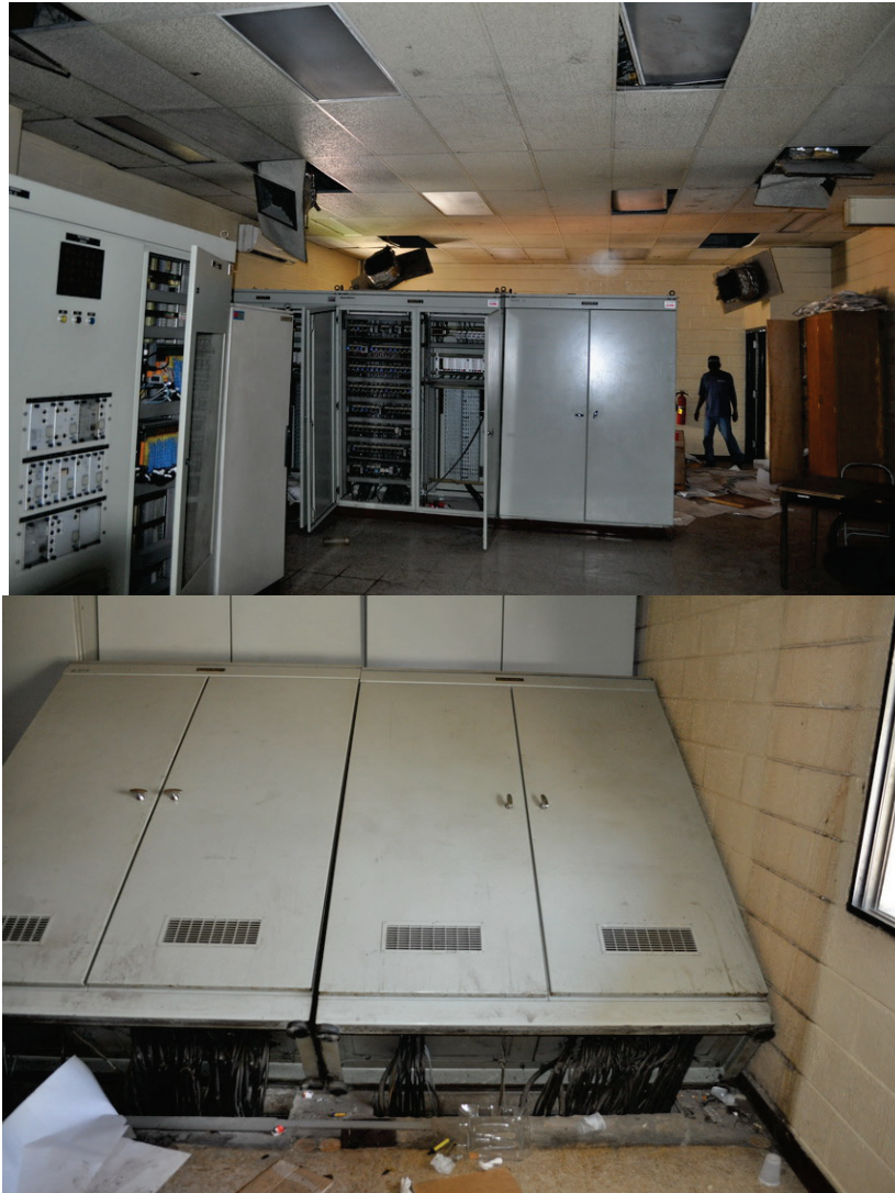
Figure 6.4.7.1-3 Damage to unanchored electrical cabinets at power plant in Port-au-Prince in the 2010 magnitude-7 Haiti Earthquake (Photos courtesy of Eduardo Fierro, BFP Engineers).
