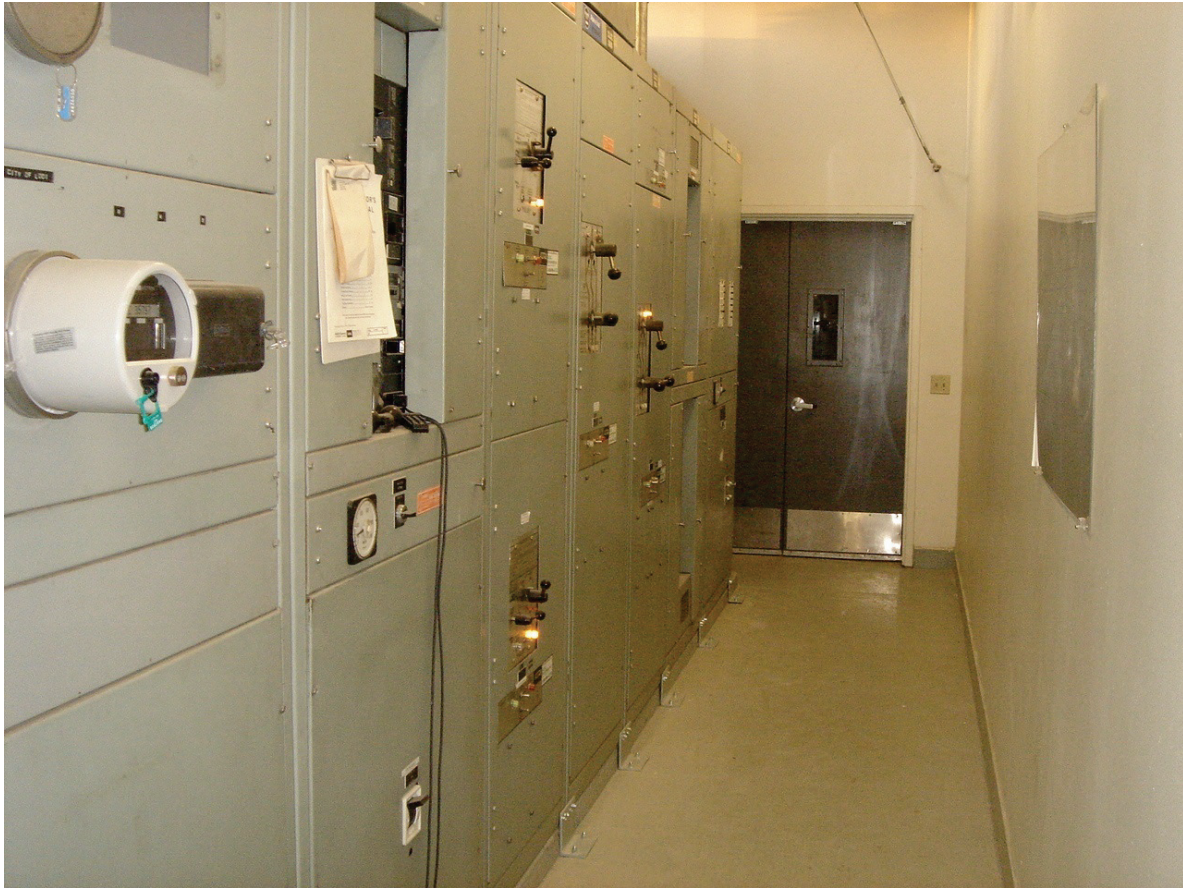
Figure 6.4.7.1-9 Anchorage for electrical cabinets. Anchorage to wall at top of cabinets is also present but not visible (Photo courtesy of Maryann Phipps, Estructure).
