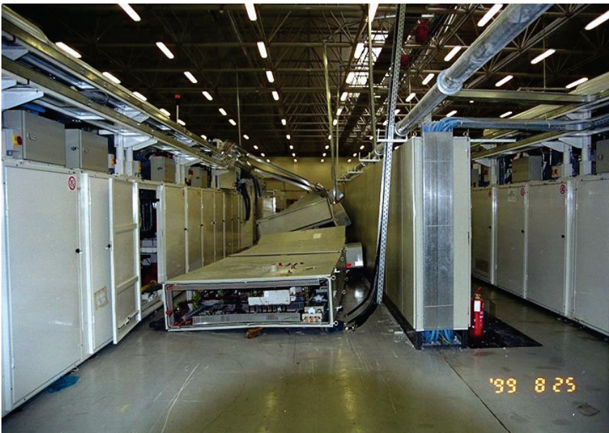
Figure 6.4.7.1-2 Unanchored electrical cabinets overturned in a paper products plant during the 1999 magnitude-7.4 Izmit, Turkey earthquake (Photo courtesy of NISEE Izmit Collection, No. IZT-682, photograph by Halil Sezen).
