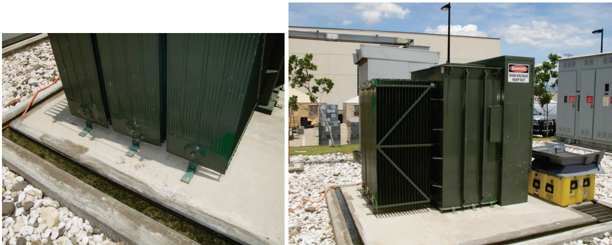
Figure 6.4.7.3-5 Outdoor liquid type electrical power transformer which converts incoming medium voltage to 480 volt utilization voltage for critical facility. Note use of manufacturer supplied diagonal elements on cooling fin assembly to minimize dynamic loading on liquid filled fin assembly which contains numerous welded connections. Post earthquake photo from the 2010 M 7.0 Haiti Earthquake (photos courtesy of Philip J. Caldwell).
