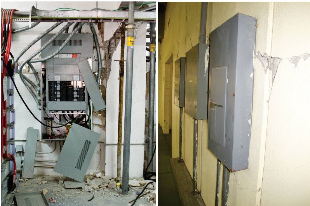
Figure 6.4.7.3-8 Example of rugged equipment. Post earthquake photos of two different essential facilities which sustained significant structural damage during the 2010 M 7.0 Haiti Earthquake. Wall mounted electrical power distribution panels were undamaged and remained functional even though the walls they were mounted to were severely damaged during the earthquake (photos courtesy of Philip J. Caldwell).
