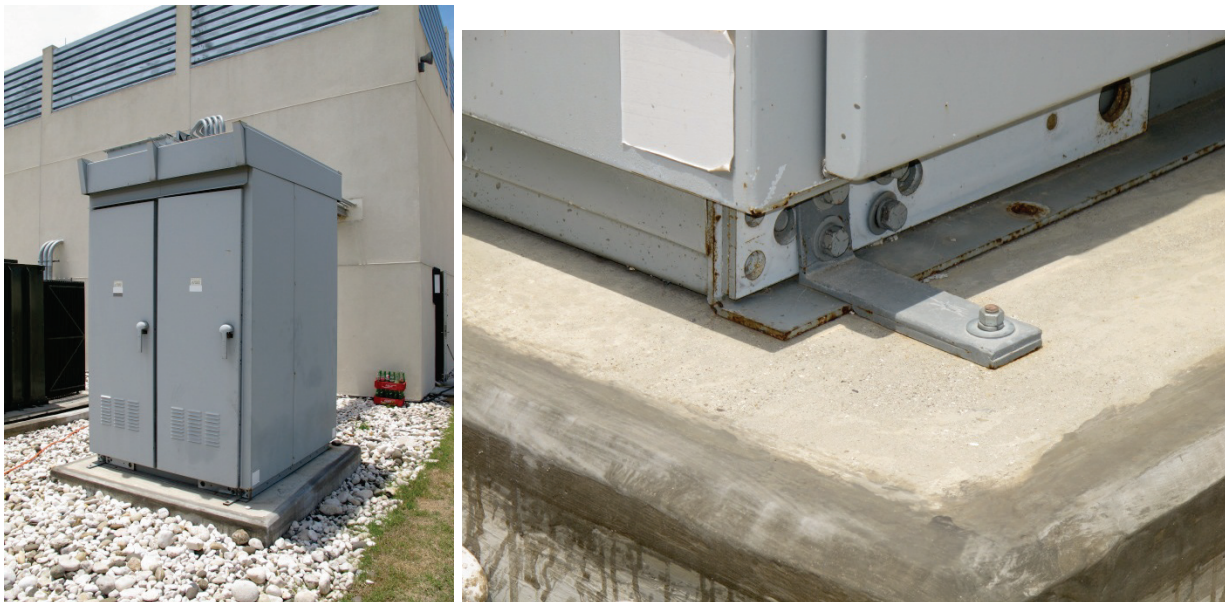
Figure 6.4.7.3-4 Outdoor low voltage switchgear supplying incoming utility power to critical facility. Note equipment frame seismic anchorage load path is bolted at both equipment frame and pad with a continuous rigid load path. Post earthquake photo from the 2010 M 7.0 Haiti earthquake. (photos courtesy of Philip J. Caldwell)
