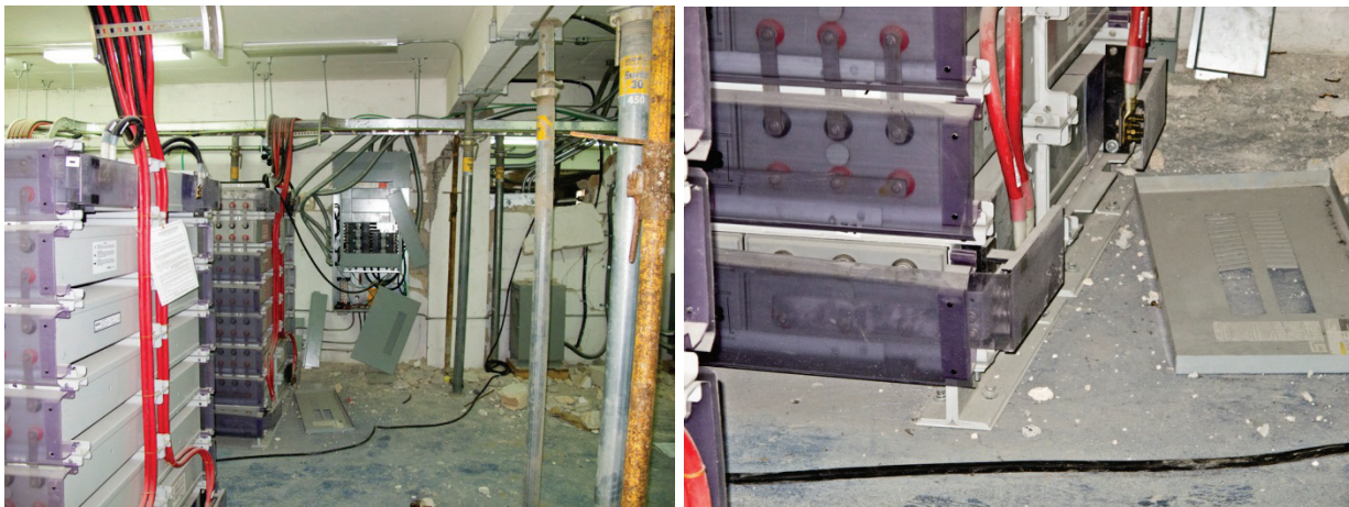
Figure 6.4.7.3-6 Battery room for central network cell phone carrier after 2010 M 7.0 Haiti Earthquake. Three-story building which contained the UPS (uninterruptable power supply) and battery room was newly constructed and suffered near collapse structural damage which required structural demolition and replacement. Note that high mass batteries with integral structural system was rigidly anchored and sustained no damage or loss of operation despite building structural system displacing enough to shear support columns. Cellular carrier representative advised that the central network support functionality was maintained during Earthquake (photos courtesy of Philip J. Caldwell).
