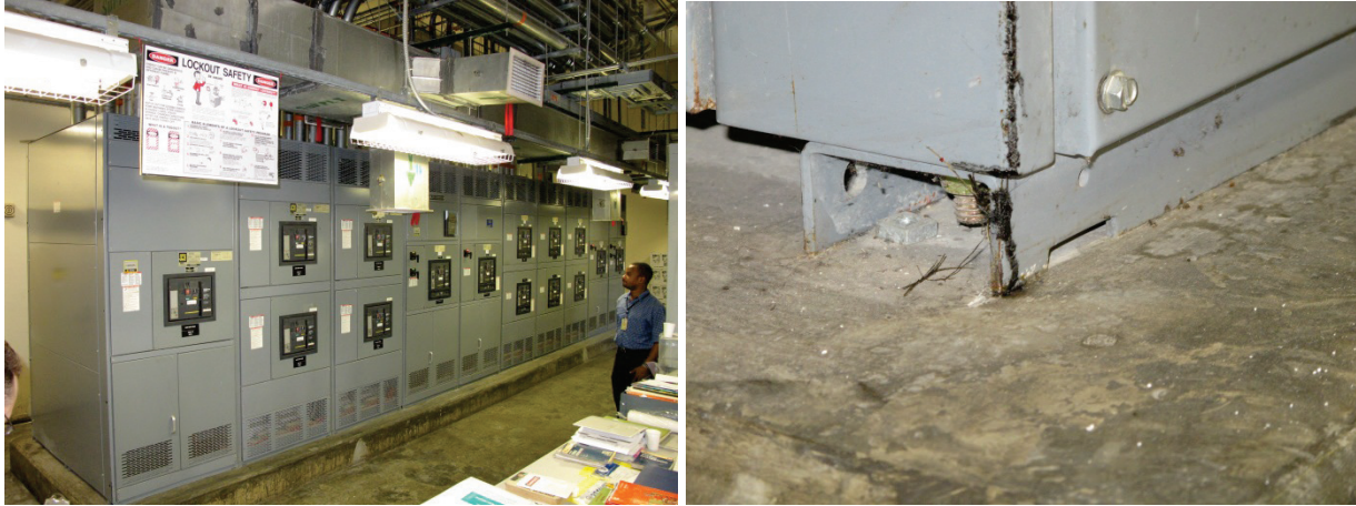
Figure 6.4.7.3-9 Incoming power switchgear for critical facility anchored through base undamaged by the 2010 Haiti M 7.0 Earthquake. Visual inspection of equipment base channels did not reveal any structural damage or equipment displacement on concrete equipment pad. Similar equipment located nearby which did not have a rigid seismic restraint with a continuous load path shifted on its pad (photos courtesy of Philip J. Caldwell).
