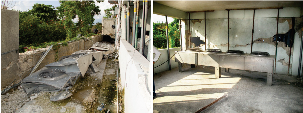
Figure 6.4.7.3-7 Heat rejection mechanical units which provide cooling for servers in cellular carrier central network facility (left photo). Collapsing security wall during the 2010 M 7.0 Haiti Earthquake crushed these units and resulted cyclical total failure of the cellular network as the servers hit temperature limits, shut down, rebooted and heated up again. System stability was restored by replacing the damaged units with temporary ones (right photo). Example of how the reliability of a critical facility essential system is both dependent upon adequate seismic restraints and a location which is free of structural and nonstructural falling hazards (photos courtesy of Philip J. Caldwell).
