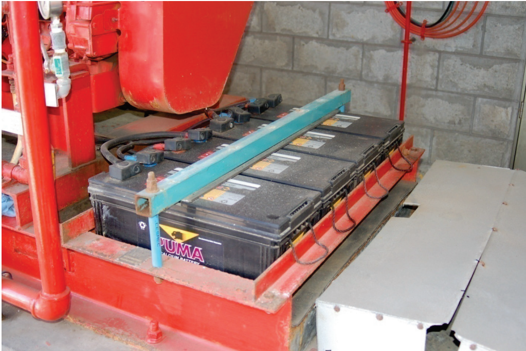
Figure 6.4.7.4-3 Batteries anchored with equipment skid (Photo courtesy of Eduardo Fierro, BFP Engineers).
