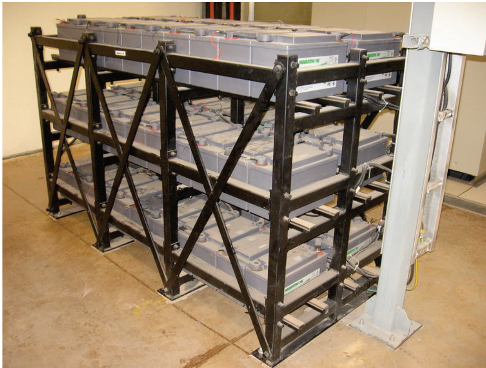
Figure 6.4.7.4-4 Battery rack that performed well in the 2010 magnitude-8.8 Chile Earthquake (Photo courtesy of Rodrigo Retamales, Rubén Boroschek & Associates).
