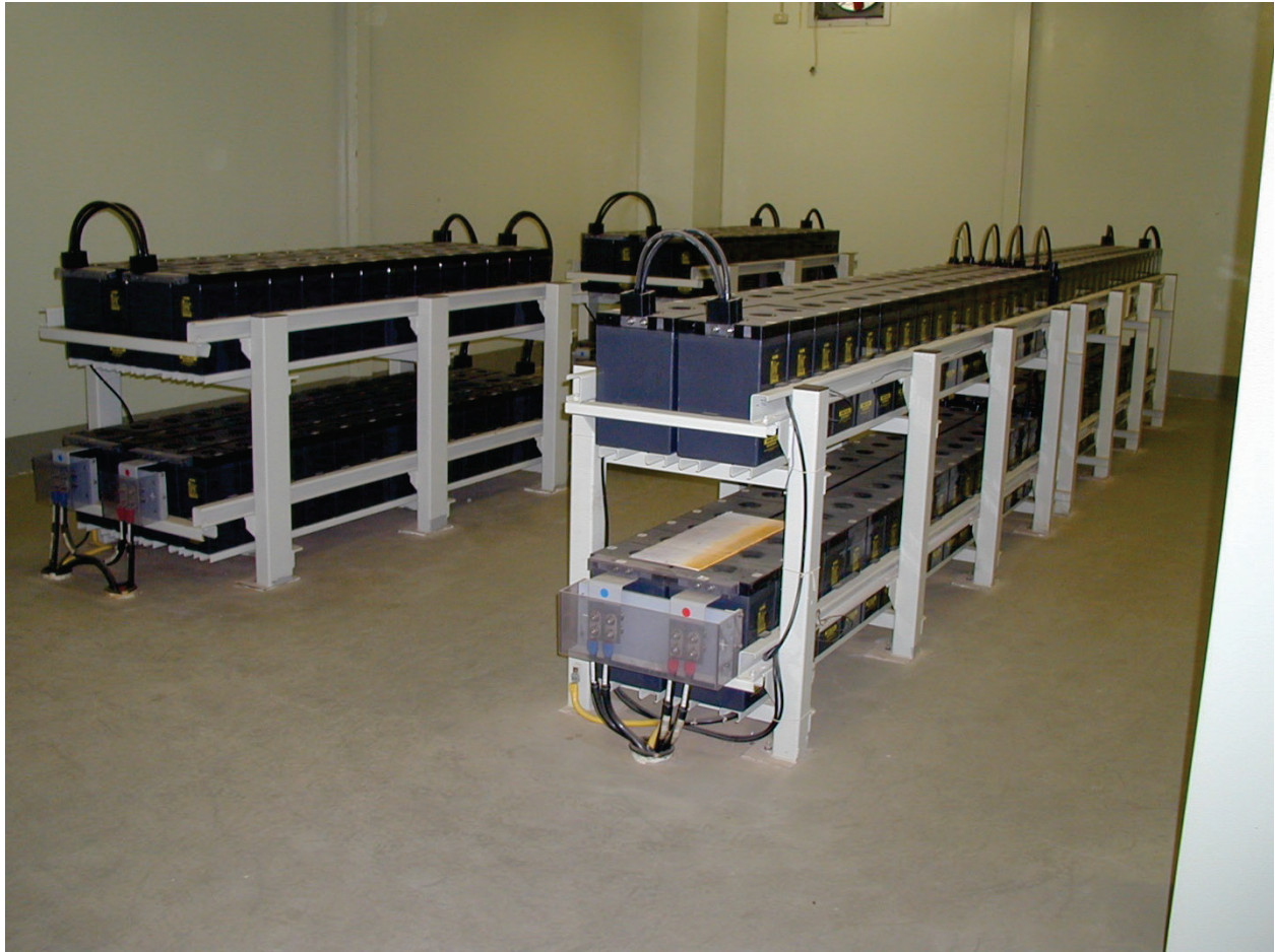
Figure 6.4.7.4-2 Anchored battery racks (Photo courtesy of Eduardo Fierro, BFP Engineers).
