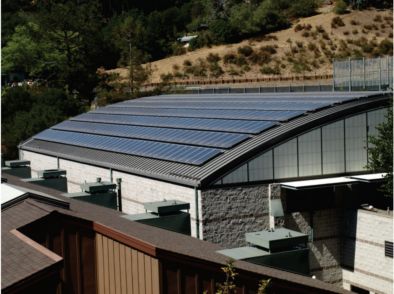
Figure 6.4.7.5-4 Flush mount photovoltaic system on barrel shaped roof of gymnasium at Head-Royce School, Oakland, California (Photo courtesy of Cynthia Perry, BFP Engineers).
