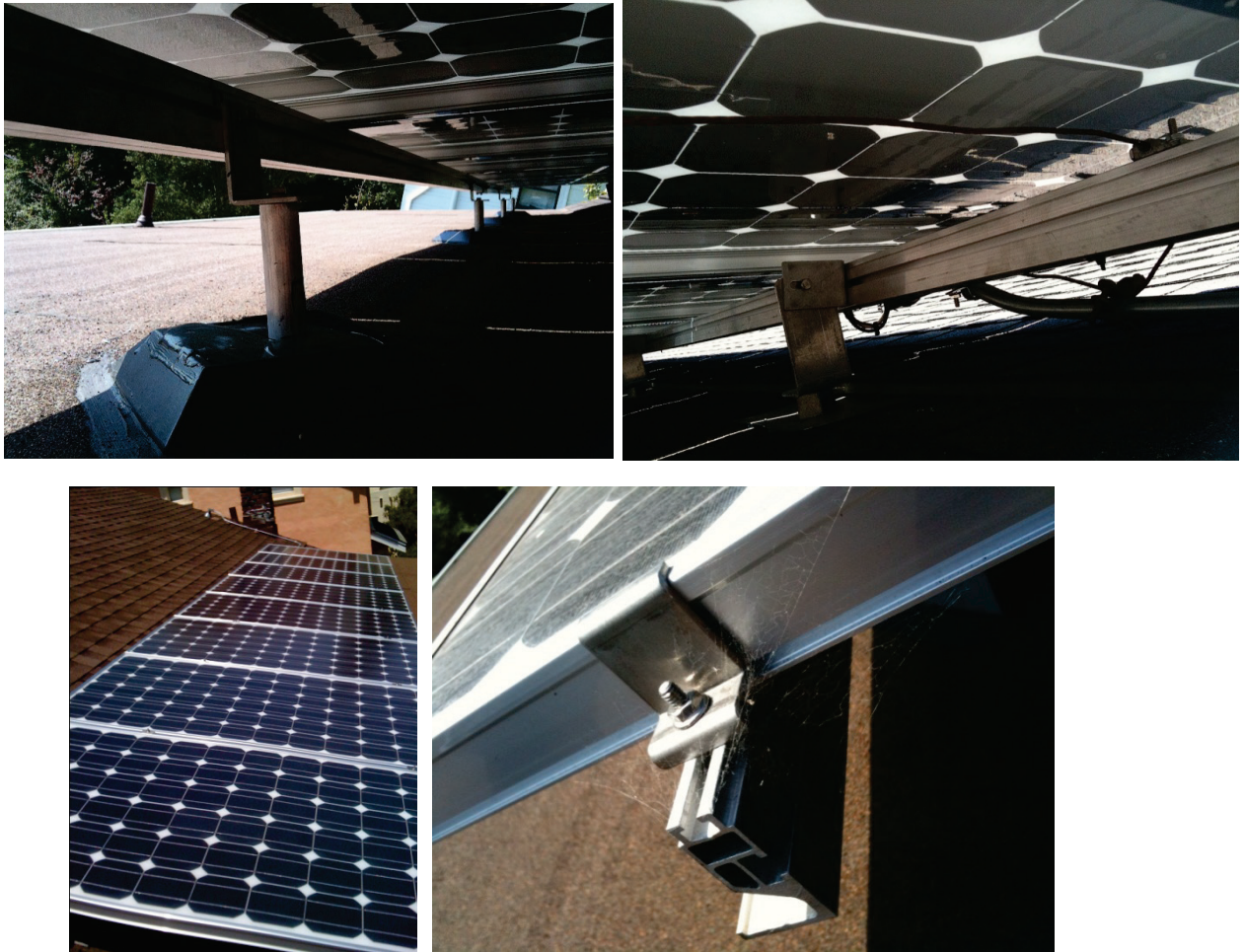
Figure 6.4.7.5-3 Residential photovoltaic system in Berkeley, California mounted over the transition between two different roof slopes (Photos courtesy of Heber Santos). Short standoff used on tar and gravel flat portion (upper left); aluminum flashing and mounting bracket used on sloped portion with composition tile roofing (upper right). The profile of one type of proprietary mounting track is seen at lower left.
