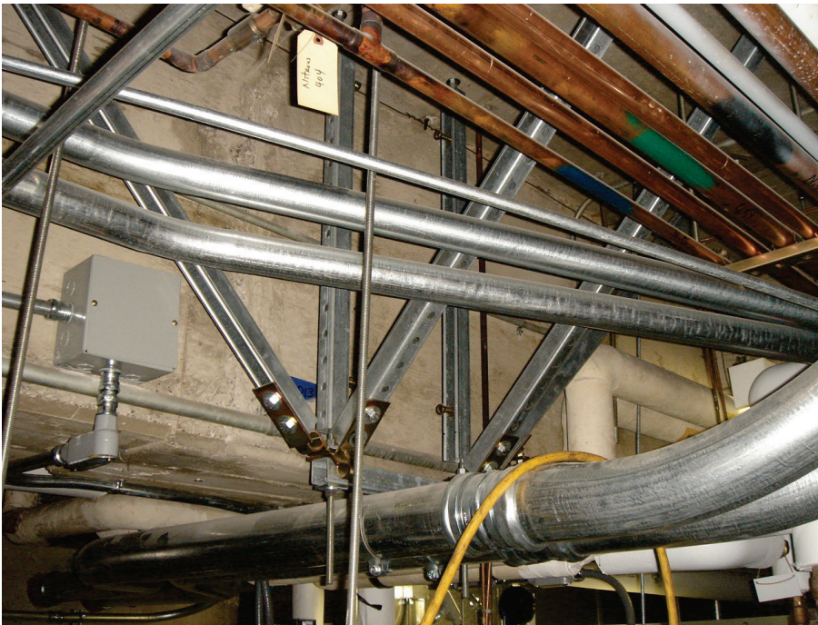
Figure 6.4.8.1-3 Rigid strut bracing for trapeze supporting electrical conduit; conduit attached to trapeze with conduit clamp that provides lateral and longitudinal restraint (Photo courtesy of Maryann Phipps, Estructure).
