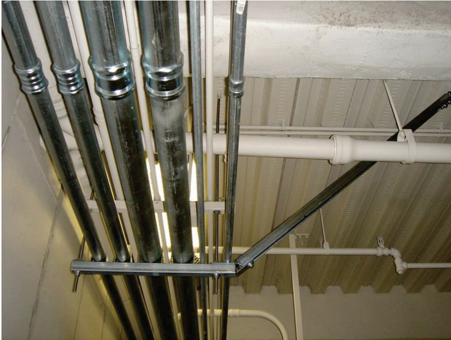
Figure 6.4.8.1-2 Rigid strut bracing provides restraint against earthquake forces perpendicular to the piping. Similar bracing is required in the direction parallel to the conduit (Photo courtesy of Maryann Phipps, Estructure).
