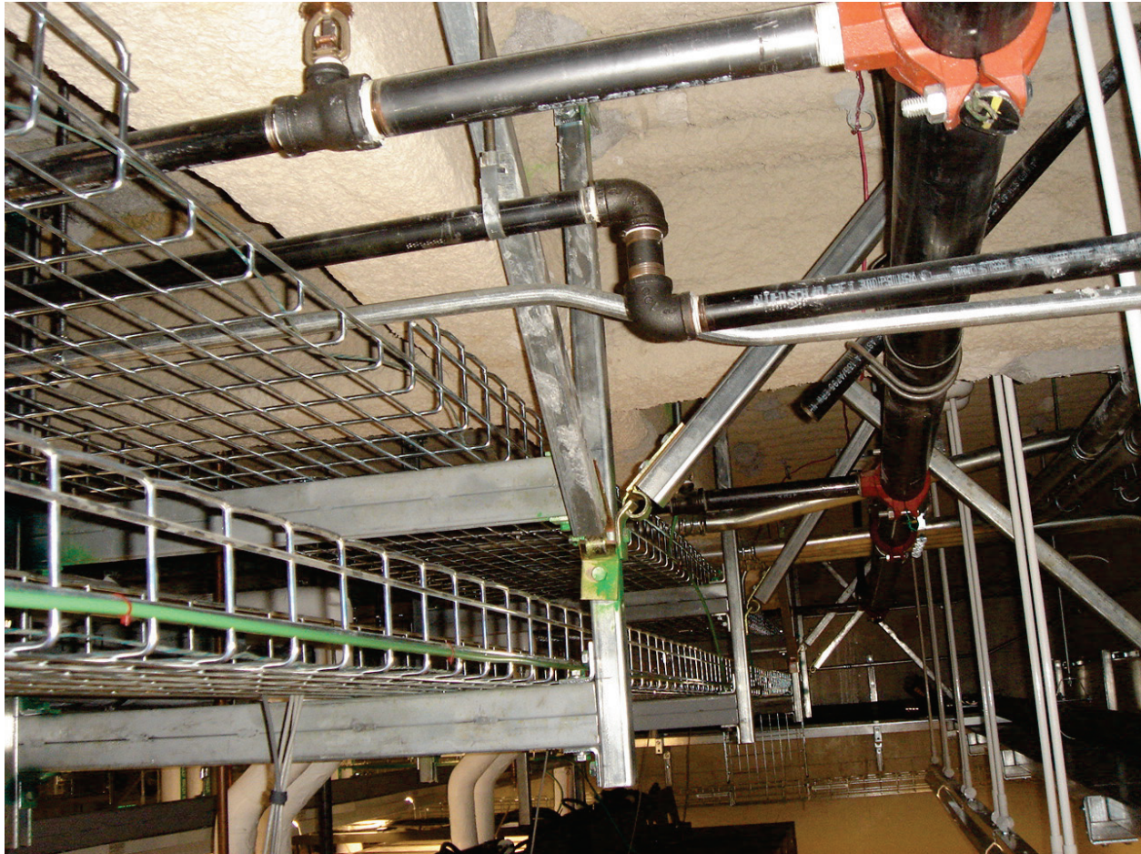
Figure 6.4.8.1-4 Lateral and longitudinal rigid strut bracing for trapeze supporting electrical raceways (Photo courtesy of Maryann Phipps, Estructure).
