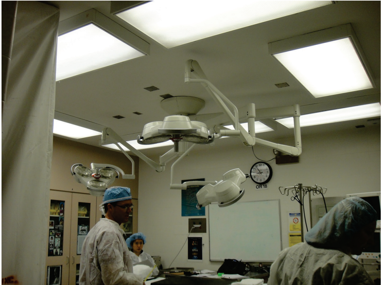
Figure 6.4.9.4-2 Engineered support and bracing are required for heavy operating room lights. The arms, joints, lenses and bulbs must be capable of resisting seismic forces. Hospital fixtures require certification. Photo also shows surface mounted fluorescent fixtures in a suspended gypsum board ceiling; each of these requires independent safety wires to the structure above; see Section 6.4.9.2 (Photo courtesy of Maryann Phipps, Estructure).
