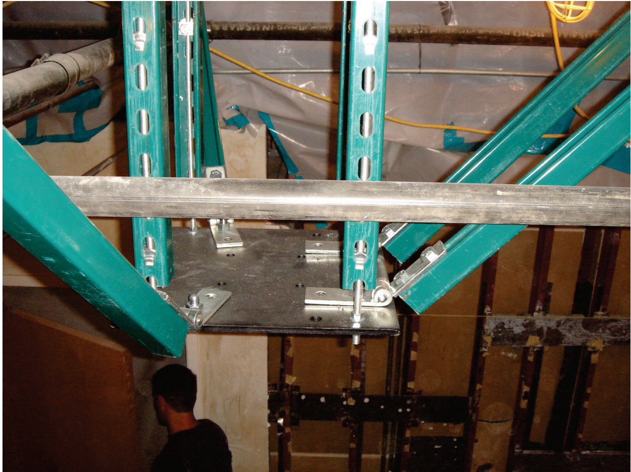
Figure 6.4.9.4-3 Engineered support and bracing for operating room lights located in California hospital. Steel plate has predrilled holes to receive fixture attachments (Photo courtesy of Maryann Phipps, Estructure).
