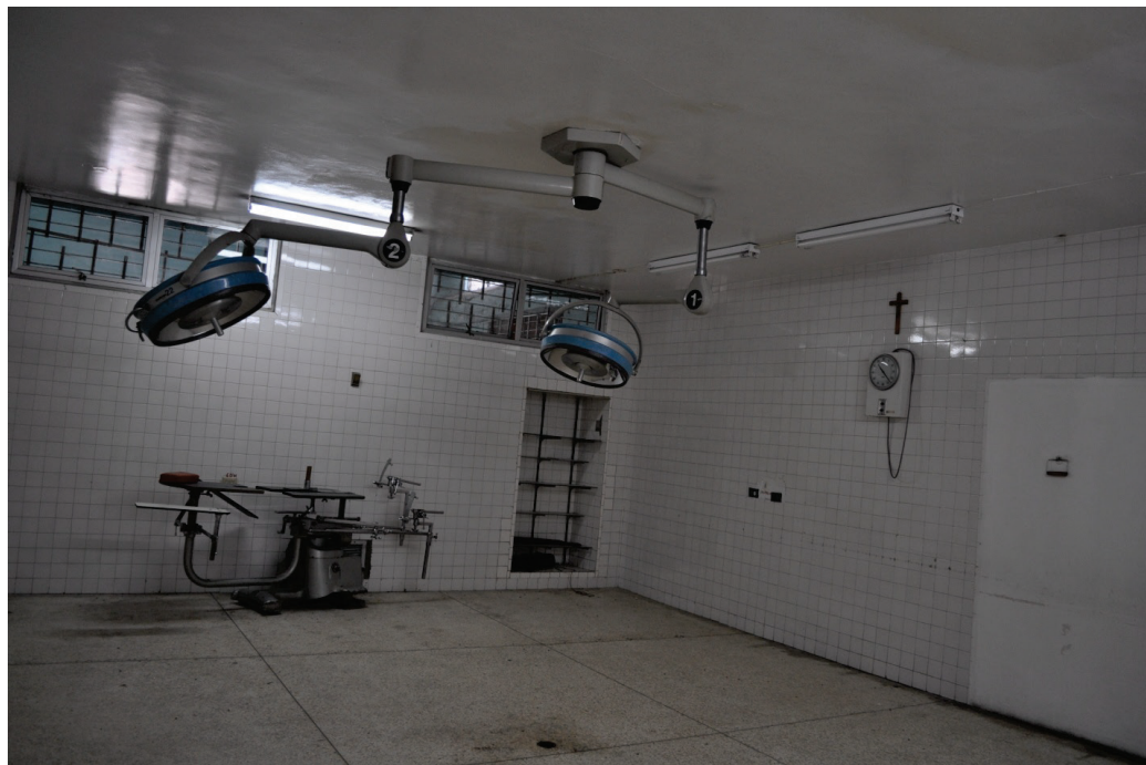
Figure 6.4.9.4-1 Operating room lights undamaged although hospital evacuated due to collapse of adjacent wing in the 2010 magnitude-7 Haiti Earthquake. Fixture anchored to underside of concrete slab (Photo courtesy of Ayhan Irfanoglu, Purdue University).
