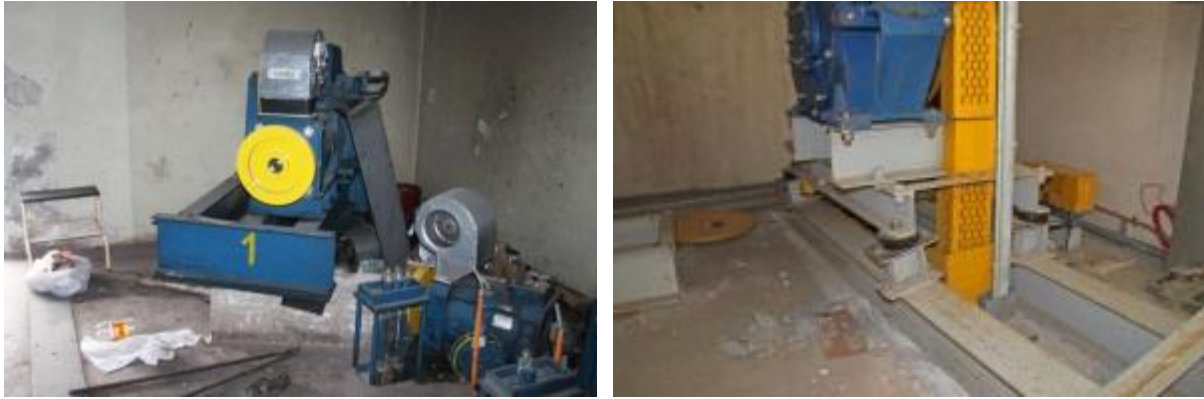
Figure 6.4.10.2-4 Examples of damage to elevator machines produced by inadequate anchorage to the structure (Photos courtesy of Eduardo Miranda, Stanford University).
