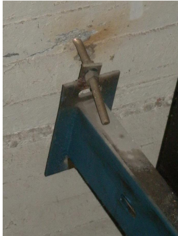
Figure 6.4.10.2-8 Damage to guide rail support brackets in the 2010 Chile Earthquake (Photo courtesy of Gilberto Mosqueda, SUNY Buffalo).
