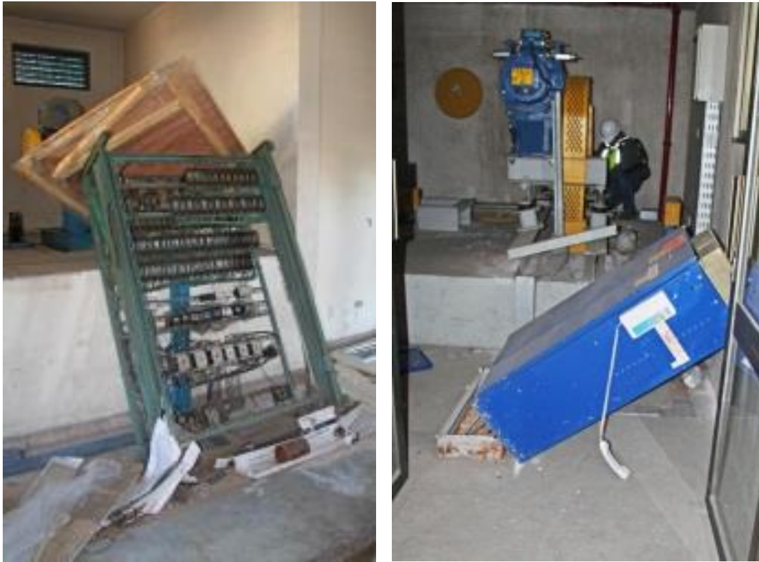
Figure 6.4.10.2-6 Overturned control panels in the 2010 Chile earthquake (Photos courtesy of Eduardo Miranda, Stanford University).
