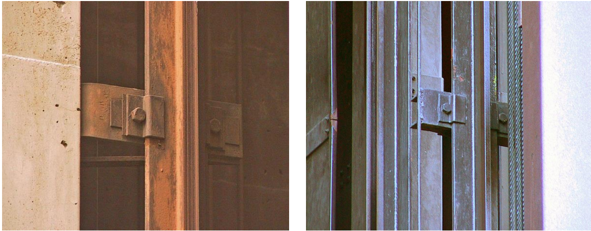
Figure 6.4.10.2-2 Examples of brackets and clips attaching the elevator guide rails to the structure (Photo courtesy of Eduardo Miranda, Stanford University).
