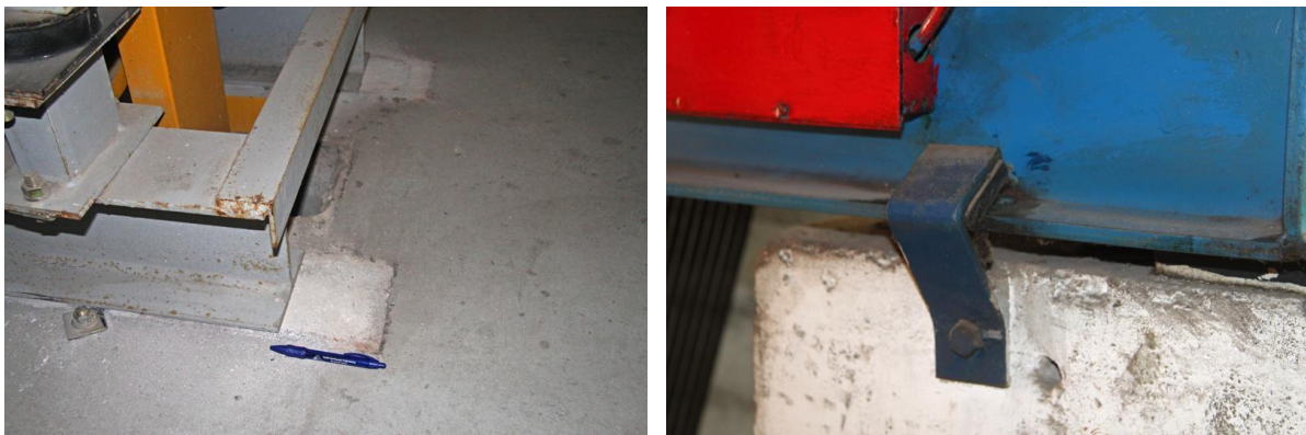
Figure 6.4.10.2-5 Details of bent bracket (left) and large displacement at the base of elevator machines (Photos courtesy of Eduardo Miranda, Stanford University).
