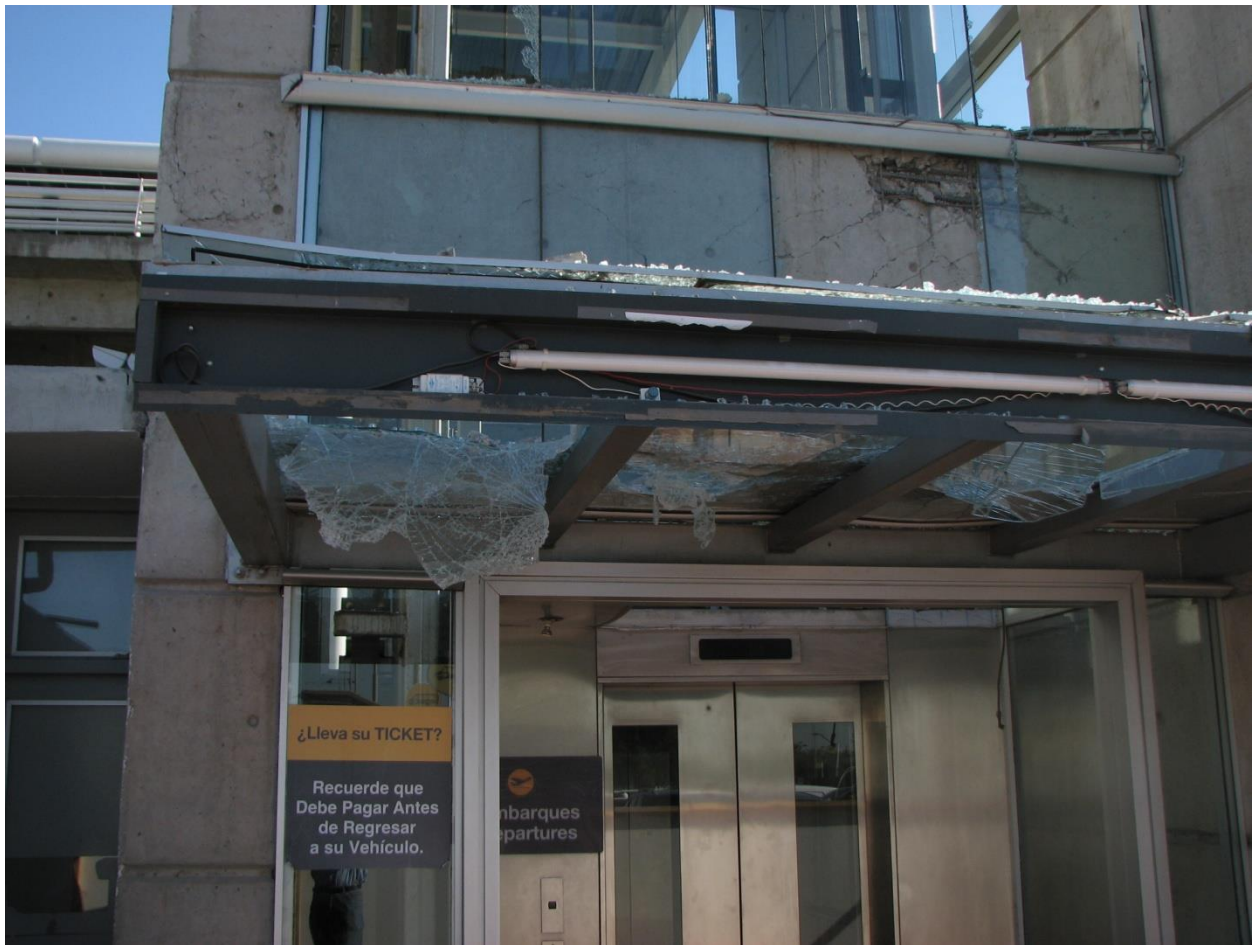
Figure 6.4.10.2-10 Glazing failures caused additional hazards at Santiago airport elevator in the 2010 Chile Earthquake (Photo courtesy of Antonio Iruretagoyena, Rubén Borsochek & Associates).
