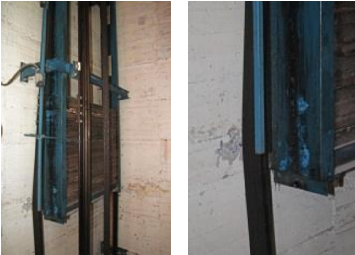
Figure 6.4.10.2-7 Damage to guide rails caused by derailment of the counterweight in a hospital in Chillan during the 2010 Chile earthquake (Photos courtesy of Eduardo Miranda, Stanford University).
