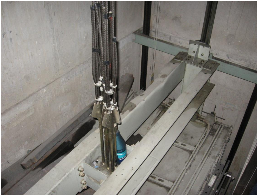
Figure 6.4.10.2-11 Unrestrained movement of the counterweights damaged the counterweight assembly and bent the counterweight guide rails; over half the subweights dropped onto the top of the cab and damaged the cab framing in the 2010
