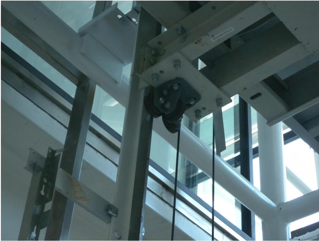
Figure 6.4.10.2-9 Derailed car roller assembly of the guide rail at the Santiago airport in the 2010 Chile Earthquake (Photo courtesy of Gilberto Mosqueda, SUNY Buffalo). The three rollers are supposed to travel along three sides of the stem of the T-shaped steel guide rail.
