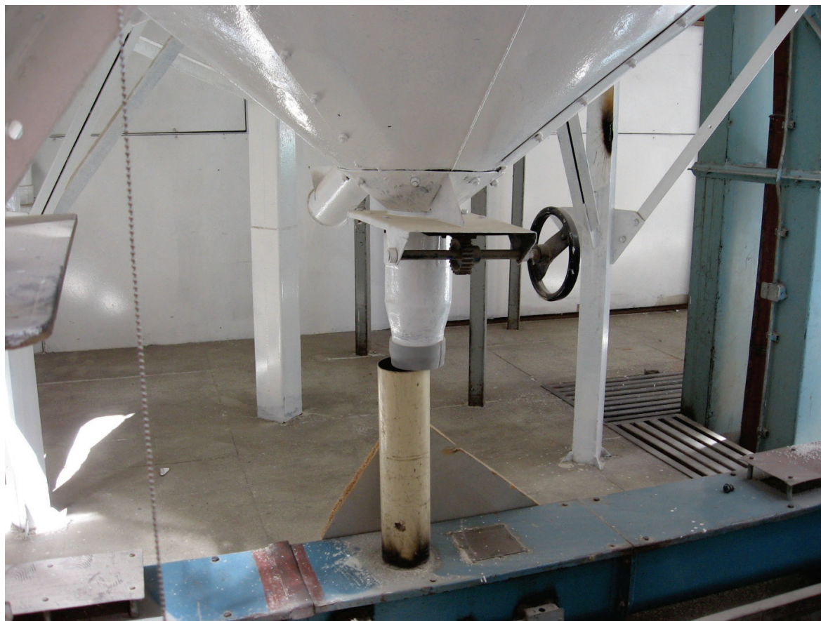
Figure 6.4.11.1-1 Misalignment between rice storage hopper and conveyor following the 2010 magnitude-8.8 Chile Earthquake (Photo courtesy of Rodrigo Retamales, Rubén Boroschek & Associates). Where various system components interface with a conveyor, the seismic restraints for the various parts should be coordinated to maintain alignment following an earthquake.
