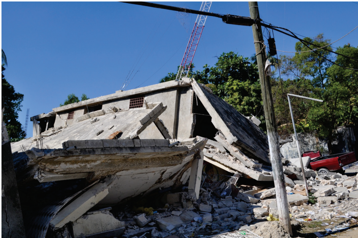
Figure 6.4.7.6-4 The antenna with guy wires remained upright atop a collapsed building in the 2010 Haiti Earthquake (Photo courtesy of Eduardo Fierro, BFP Engineers). Even though some of the guy wires went slack, the antenna did not fall into the street.
