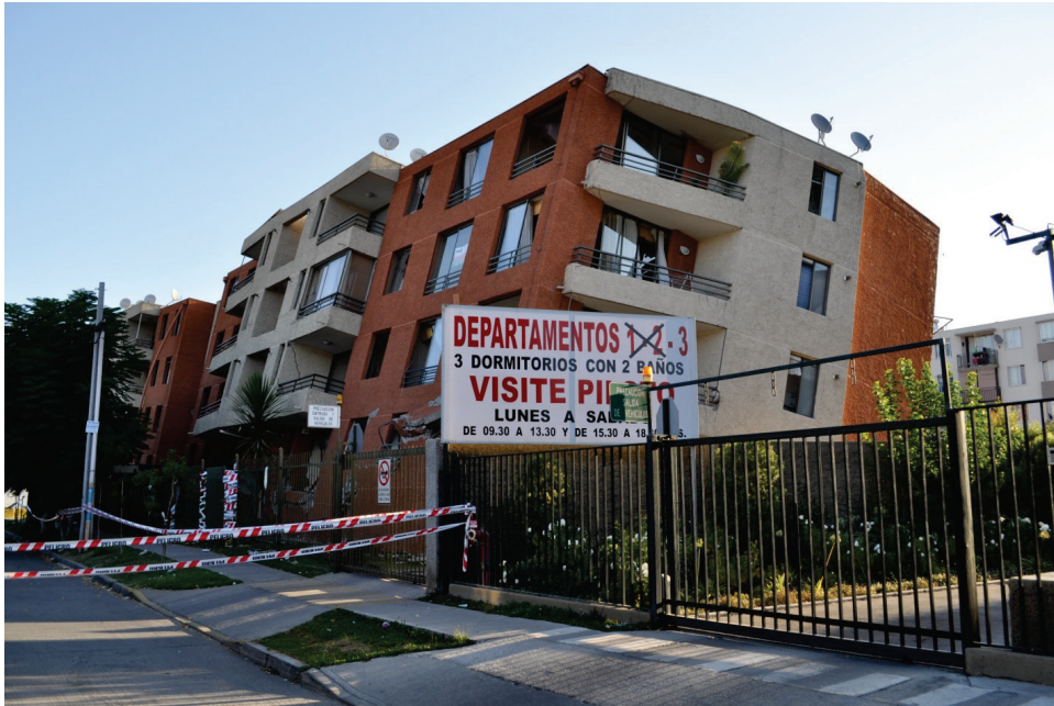
Figure 6.4.7.6-1 Most antennae are designed for wind and able to resist seismic loading. In spite of the collapse of the first story of this residential building complex, the roof-mounted antennae appear intact in the 2010 magnitude-8.8 Chile Earthquake (Photo courtesy of Eduardo Fierro, BFP Engineers).
