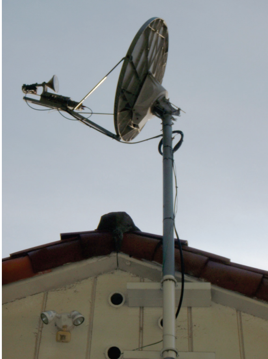
Figure 6.4.7.6-6 Antenna mast mounted to wood stud wall using blocking to clear eaves (Photo courtesy of Cynthia Perry, BFP Engineers).
