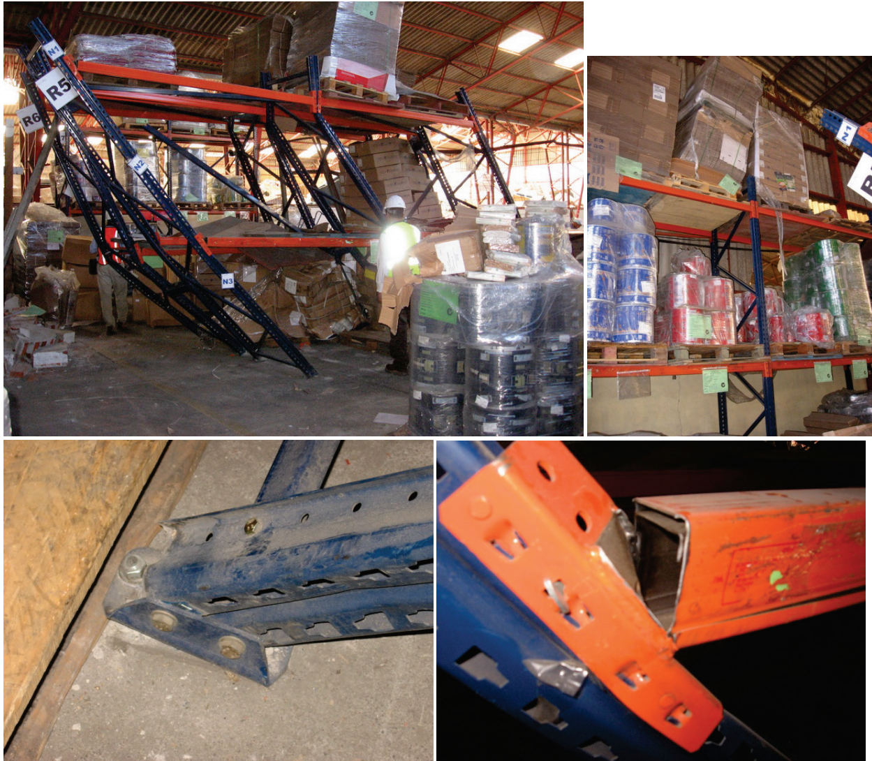
Figure 6.5.1.2-4 Failure of anchored racks in the 2010 magnitude-8.8 Chile Earthquake. The racks are leaning precariously due to inadequate bracing in the longitudinal direction and weak connections between the components. The welded fitting at the end of the beam failed at the weld in many places. Note that most items were shrink wrapped so merchandise did not scatter (Photos courtesy of Rodrigo Retamales, Rubén Boroschek & Associates).
