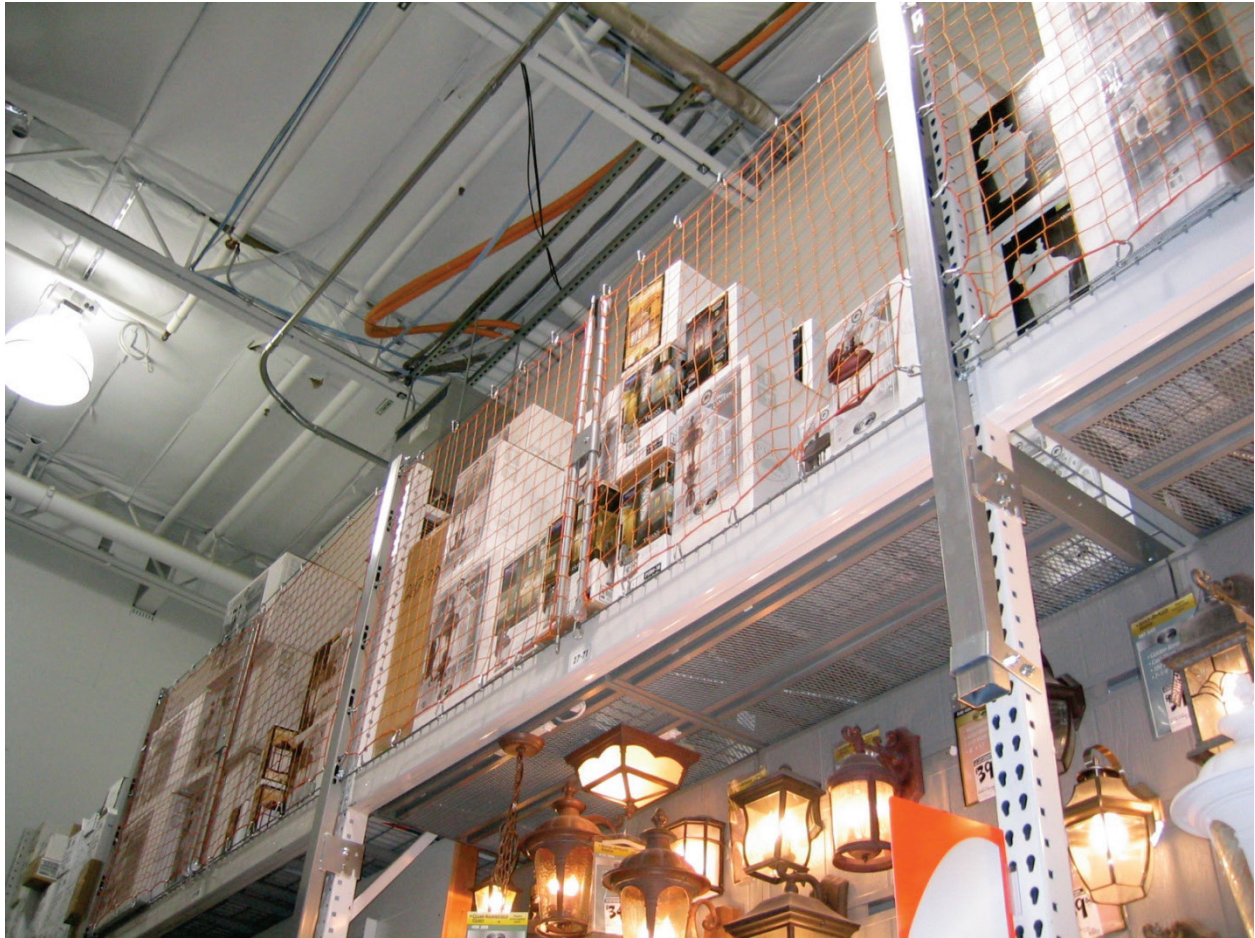
Figure 6.5.1.2-6 Photo showing netting used to keep storage on upper portions of steel storage racks in a big box hardware store (Photo courtesy of Mike Mahoney, FEMA).
