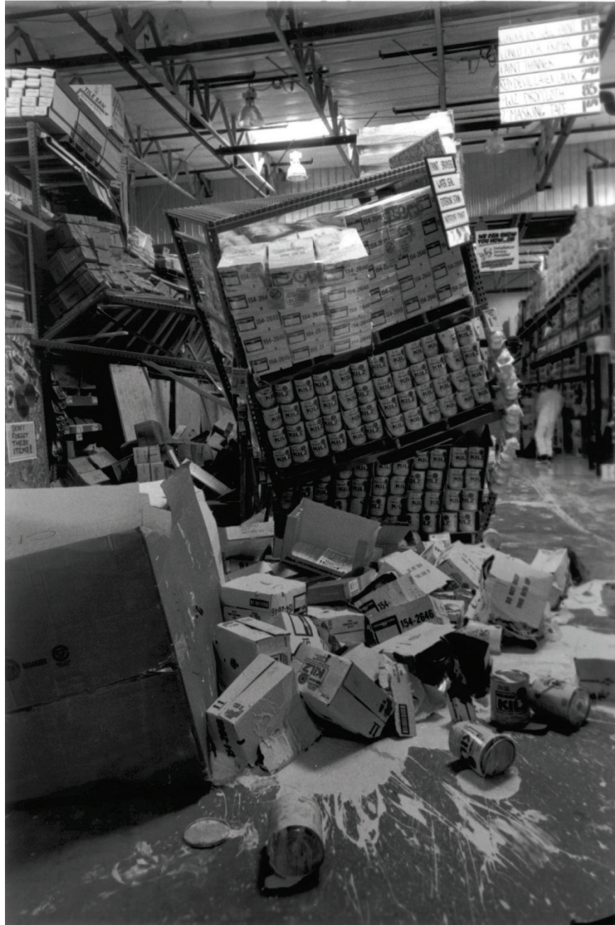
Figure 6.5.1.2-3 Rack collapse during the 1994 Northridge Earthquake. Note the minimal damage to shrink wrapped merchandise (FEMA 460, 2005).
